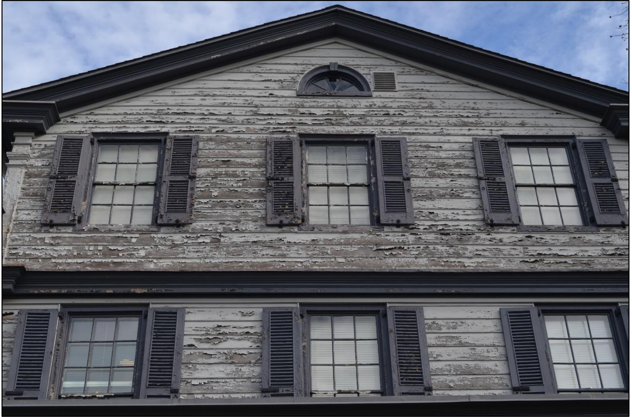
Above: Peeling paint on the exterior of the historic Fenwick Manor farmhouse, which was built in the 1820s and has been leased by the Pinelands Commission as office space since 1980.
