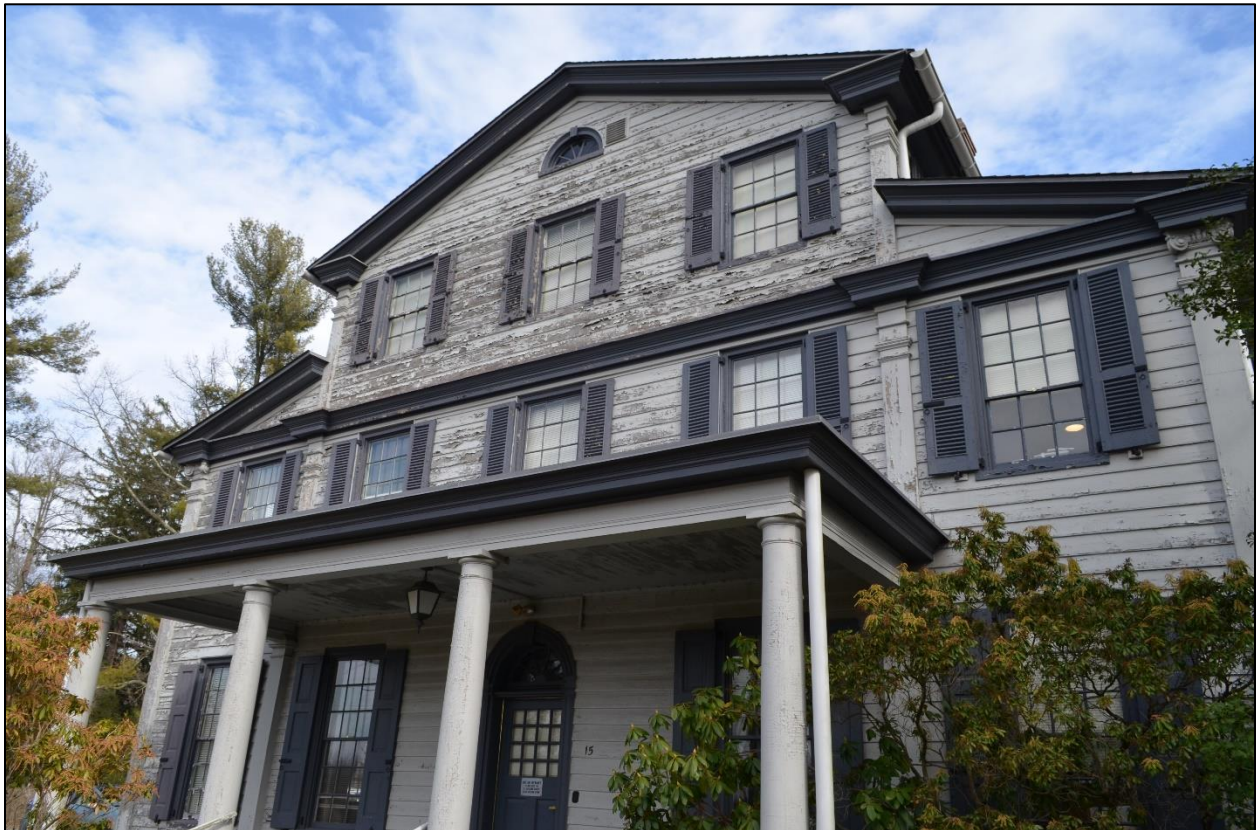
Above: Paint continues to peel off the exterior of the historic Fenwick Manor farmhouse in Pemberton Township, NJ.
