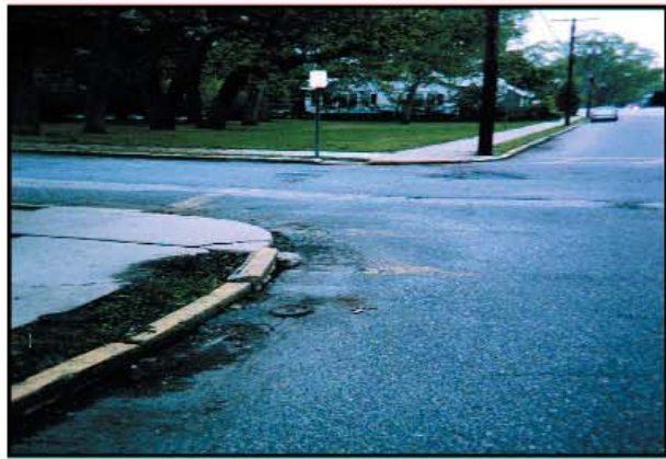
2nd & Farragut Streets, Mays Landing - deplorable maintenance for historic district
