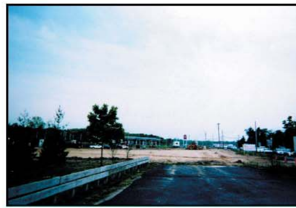
New construction on 322 & 40 - if you jam 10 pounds of mud into a 5 pound sack, you will have a problem
