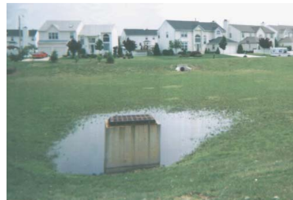
Ineffective stormwater management
