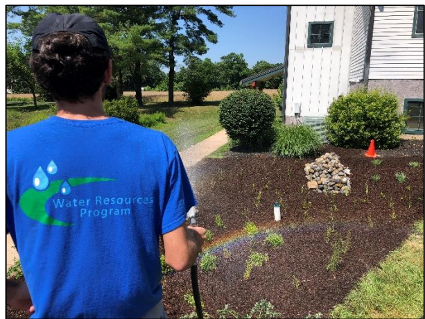
Above: The Commission installed a 340-square-foot rain garden filled with native Pinelands plants at its headquarters in late June 2022.
