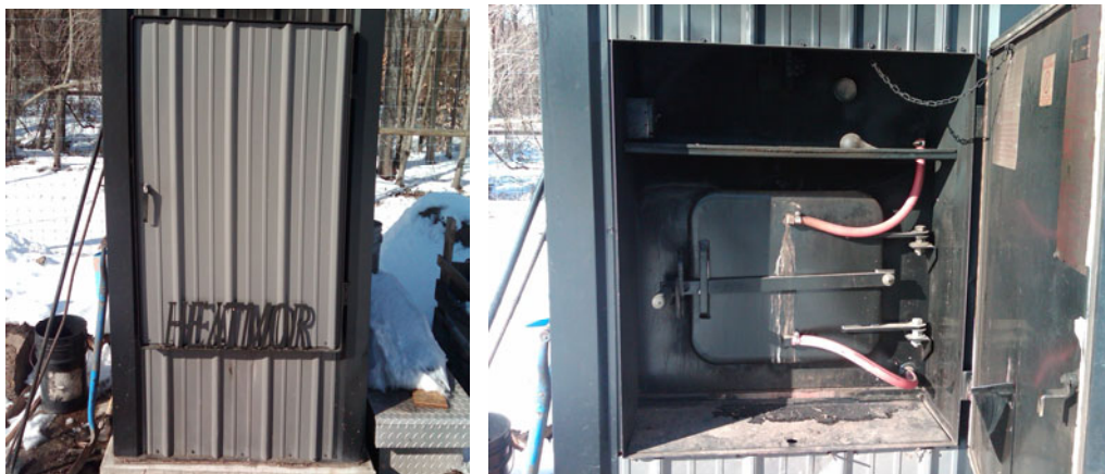
Source B – Natural Gas Boiler (Heat rating input =1 million Btu's/Hr.)
