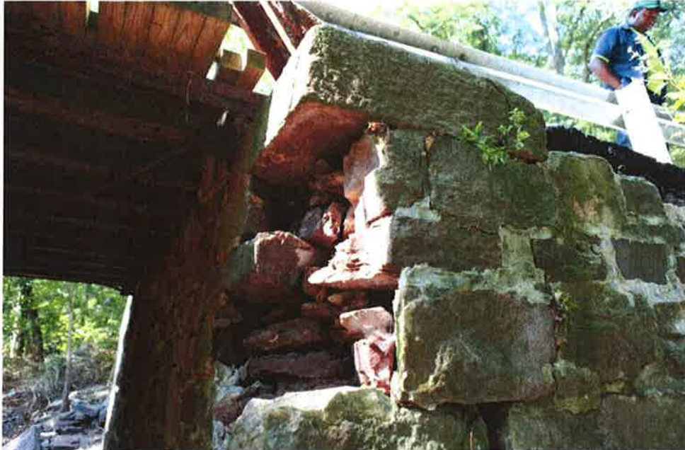
Photo 3: Area of significant concern at the northwest corner of the structure. A large void has developed below the capstone undermining more than 50% of the support area.
