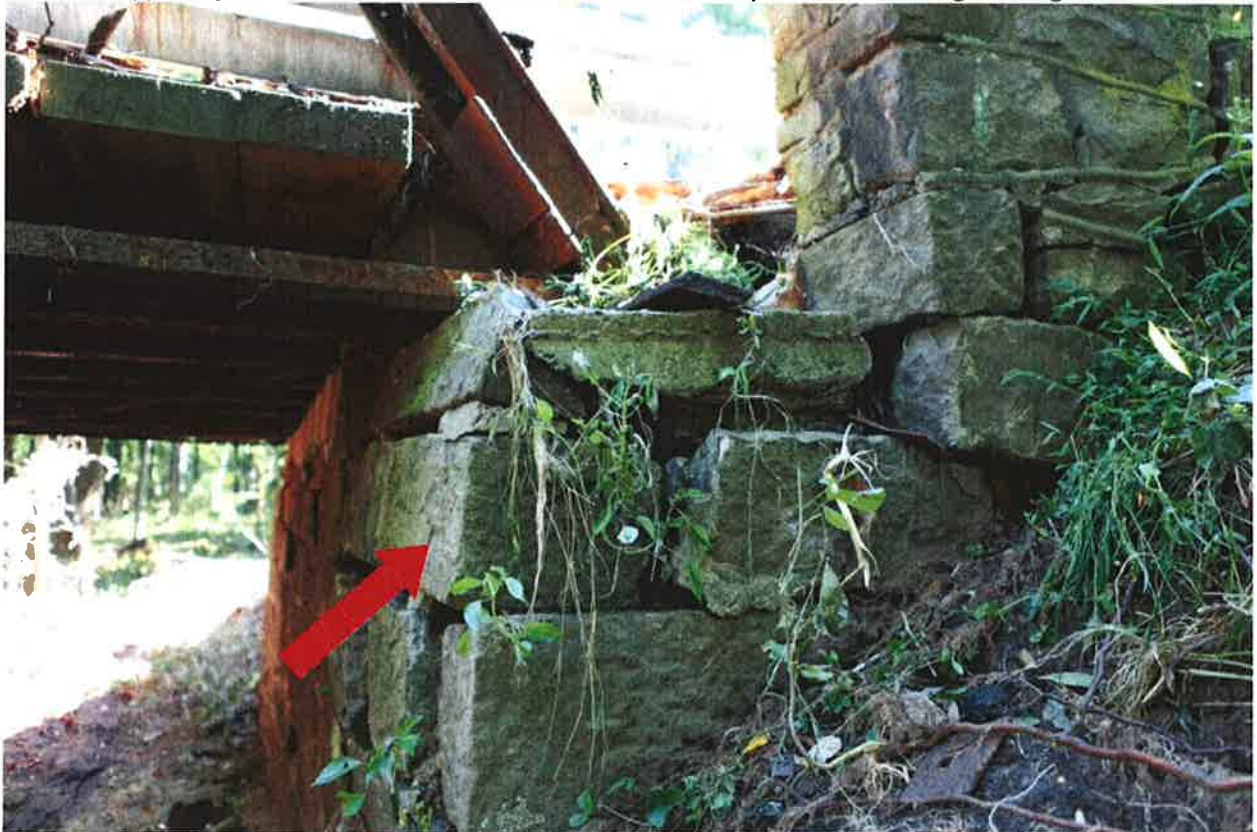
Photo 6: Loose bowed stone below the Southeast truss bearing. Looking south
