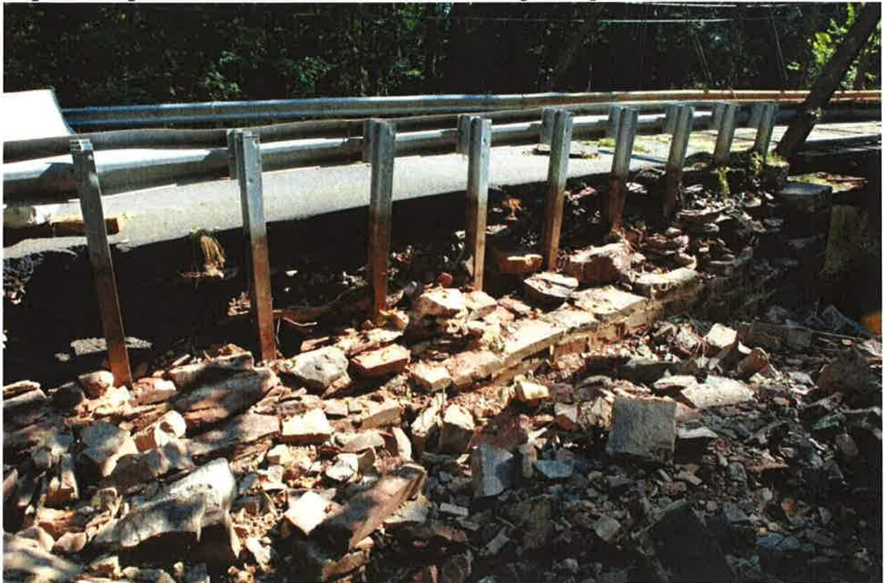
Photo 2: Complete failure of the stone wing wall on the southwest quadrant of the bridge due to large scour hole in front of the wall. Looking Northeast
