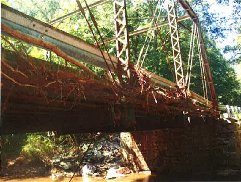
Photo 1: General view showing large amount of flood debris lodged between the lower chord of the truss and the bridge mounted guide rail. Photo taken on the north side of the bridge looking south-west.
