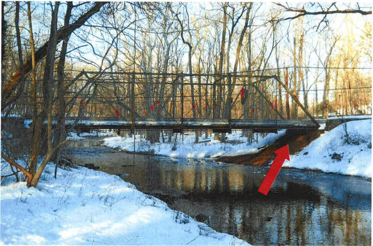
Photo 8: South Elevation of the bridge taken in February 2011. Note the location of the easterly riverbank. Looking North.
