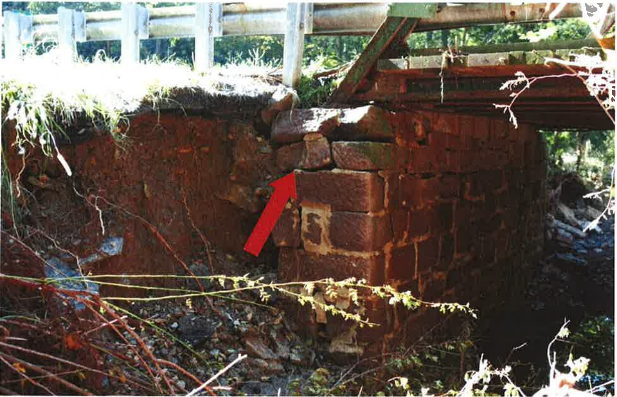
Photo 11: Large scour hole on the northeast corner of the bridge. Also note loose un-pointed stones below the truss bearing. Photo is looking southeast.
