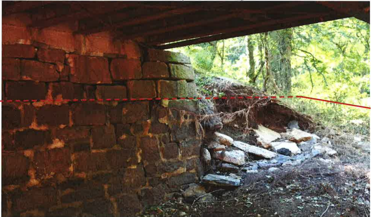
Photo 10: Location of embankment in front of the easterly abutment. Note the significant erosion in front of the stone abutment wall as compared with photo 9 and large scour hole on the southeast corner. Photo is looking southeast.
