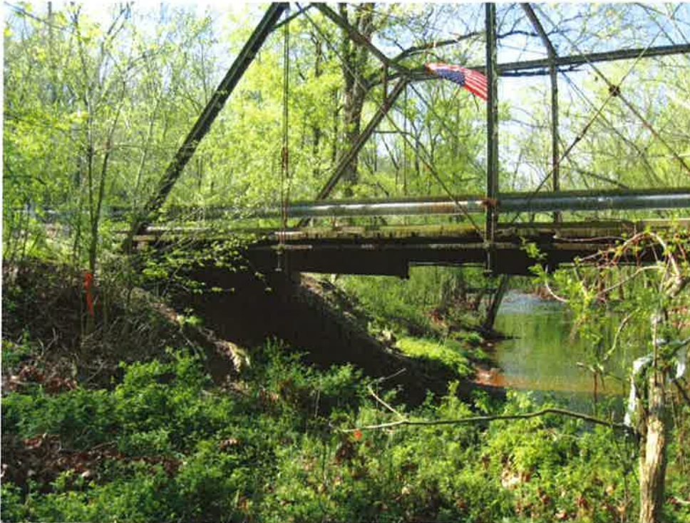
Photo 9: Location of embankment in front of the easterly abutment looking east. Photo taken on 4-27-11.
