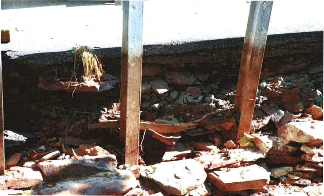
Photo 7: Undermining of the west approach roadway on the south side due to overtopping floodwaters. Looking North
