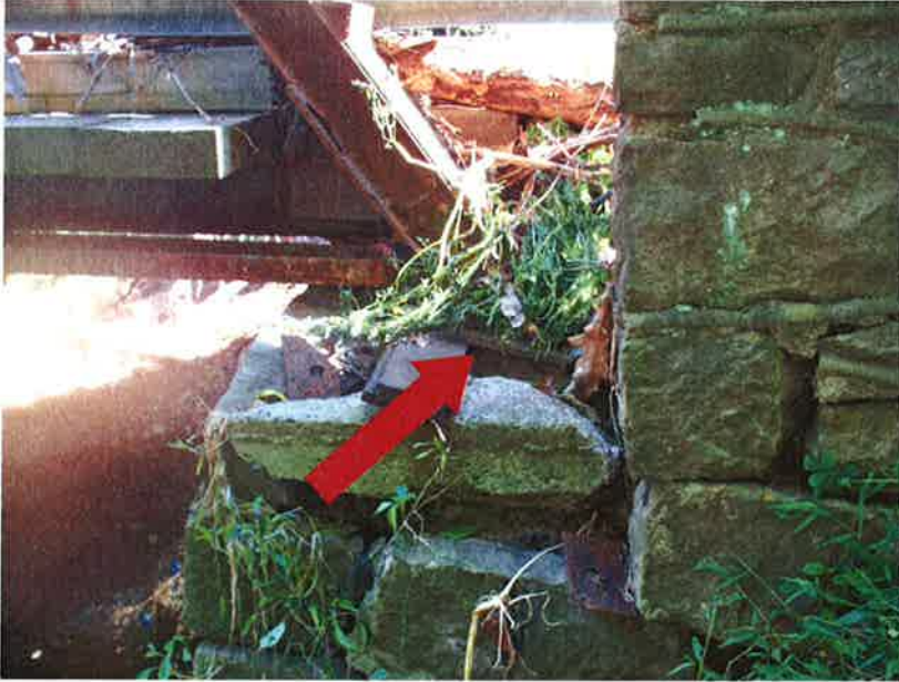
Photo 5: Southeast truss bearing exhibits settlement and rotation due to movements of the substructure. Note the loose supporting stone and lack of mortar between stones directly below the bearing. Looking north
