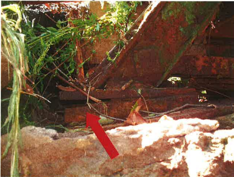
Photo 12: Rotated bearing and settled/bowed abutment.
