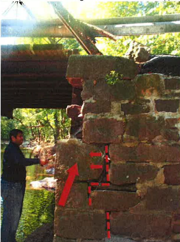
Photo 4: Note if one large stone becomes dislodged then a collapse or partial collapse of the superstructure is likely. Looking Southwest
