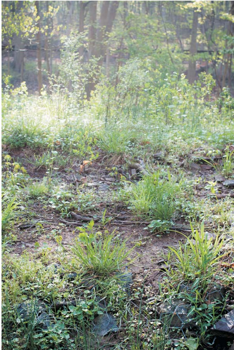
Plate 3. Exposed riprap on eastern bank of Jacob's Creel, looking east.
