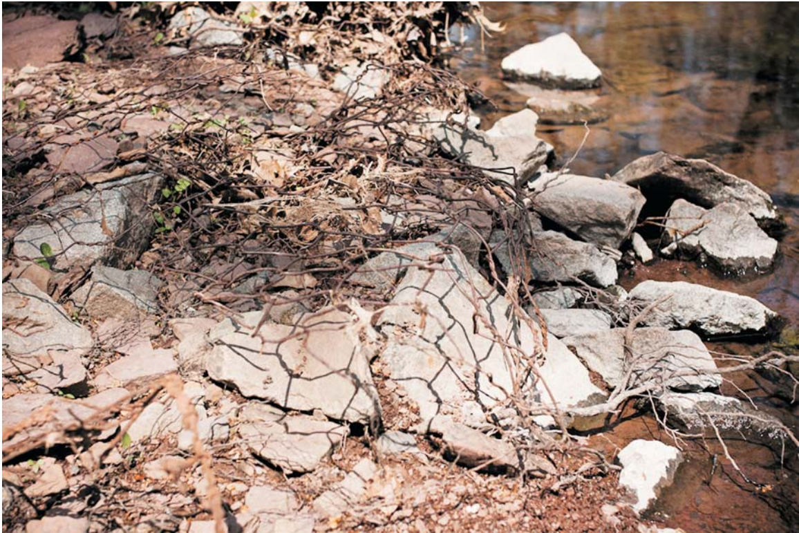
Plate 4. Exposed riprap on western bank of Jacob's Creek, looking north.
