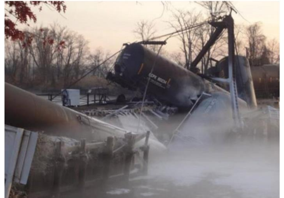
Seven train cars derailed when the bridge over the Mantua Creek collapsed Friday morning. Four tank cars containing vinyl chloride were dumped into the creek.
