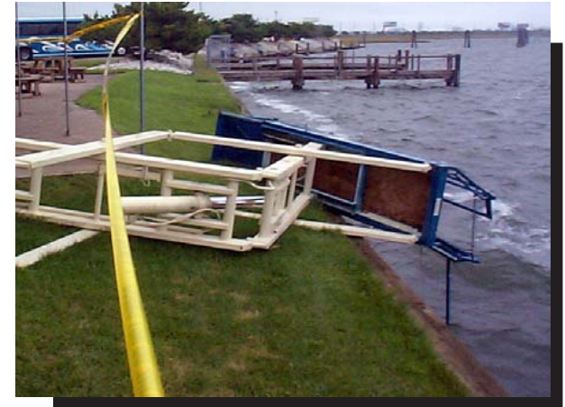
An electrician was killed when the scissor lift he was standing on tipped over. The indoor lift was being used outdoors on an uneven surface, causing it to fall. The victim was thrown into the water.
