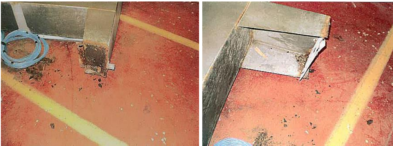
FIGURE 3. Views of cabinet foot at incident scene.
