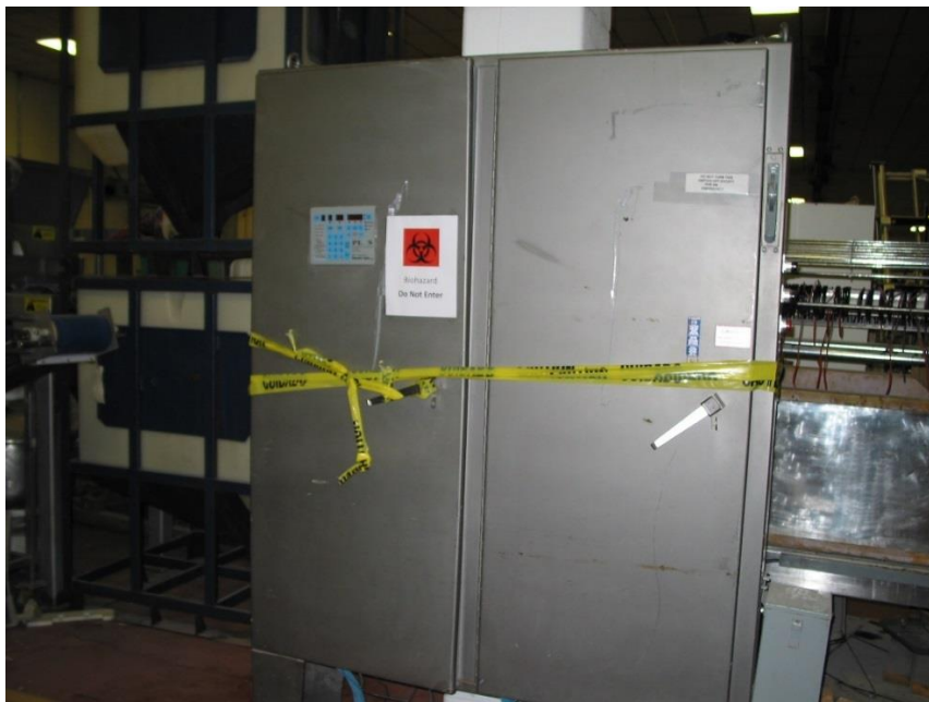
FIGURE 1: Front view of electrical cabinet upright.
