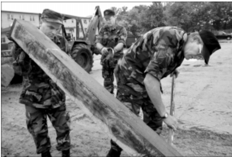
Tech. Sgt. Bob Leek (L) lifts a railroad tie while Chief Master Sgt. Herbert Mimler (R) shovels dirt underneath it. Staff Sgt. Andy Middleton (center) adjusts his gloves before joining in..
