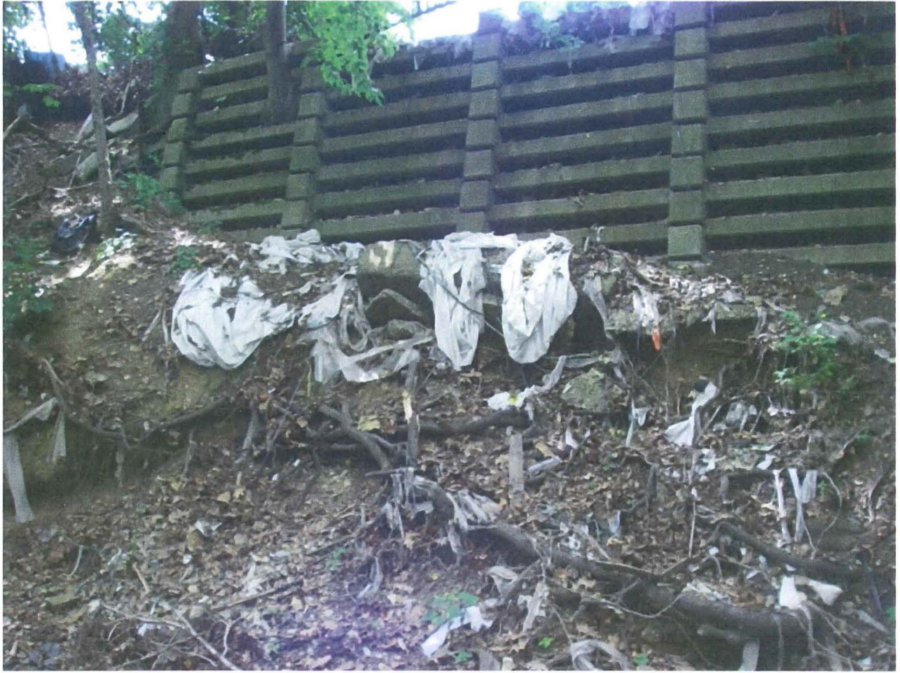
Figure 3 - Stream bank erosion and last resort erosion control - Mahwah Brook.
