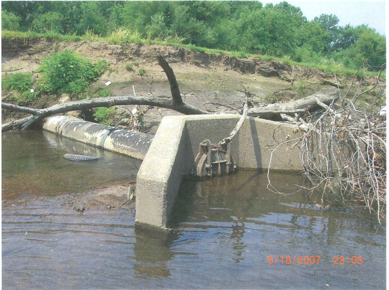
Figure 2 - This headwall once stood at the foot of the receding stream bank shown in background - Elizabeth River.
