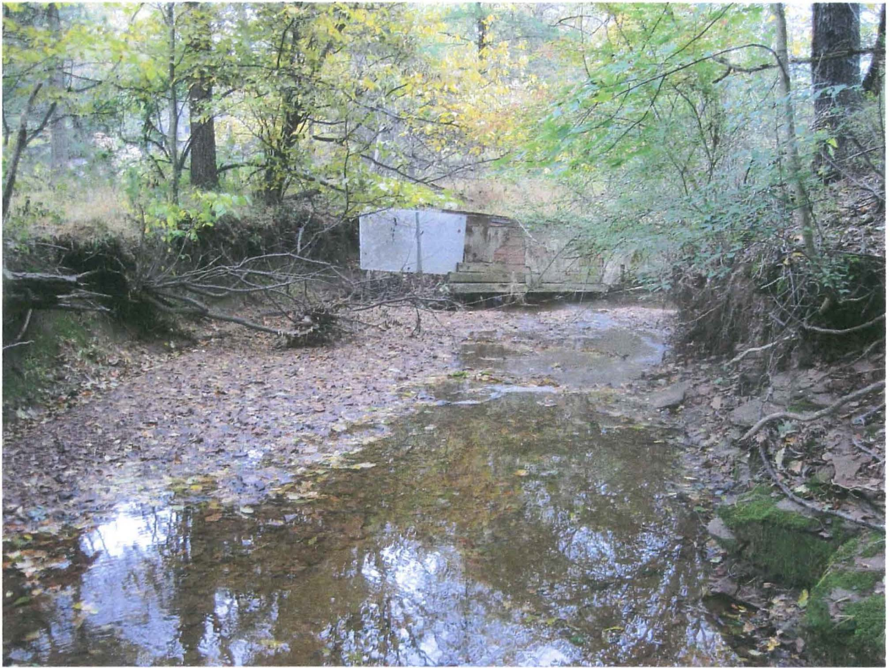
Figure 17 - The continuing onslaught of out of control Channel erosion forces homeowners to take drastic protective measures-See Figure 18.
