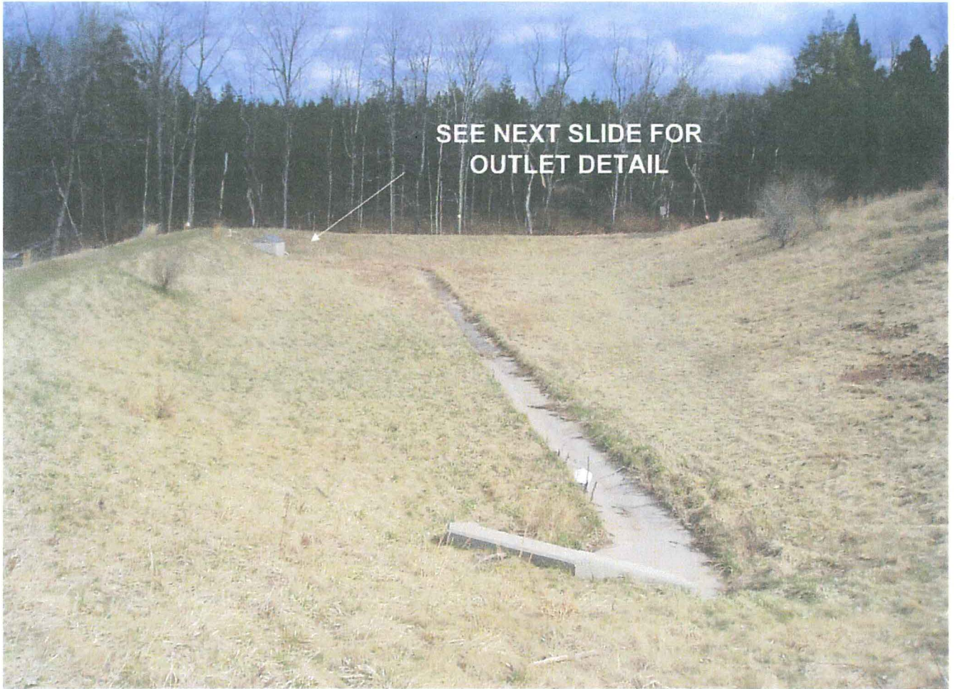
Figure 9 - Typical dry extended detention basin with concrete low flow channel - a frequently used Best Management Practice.
