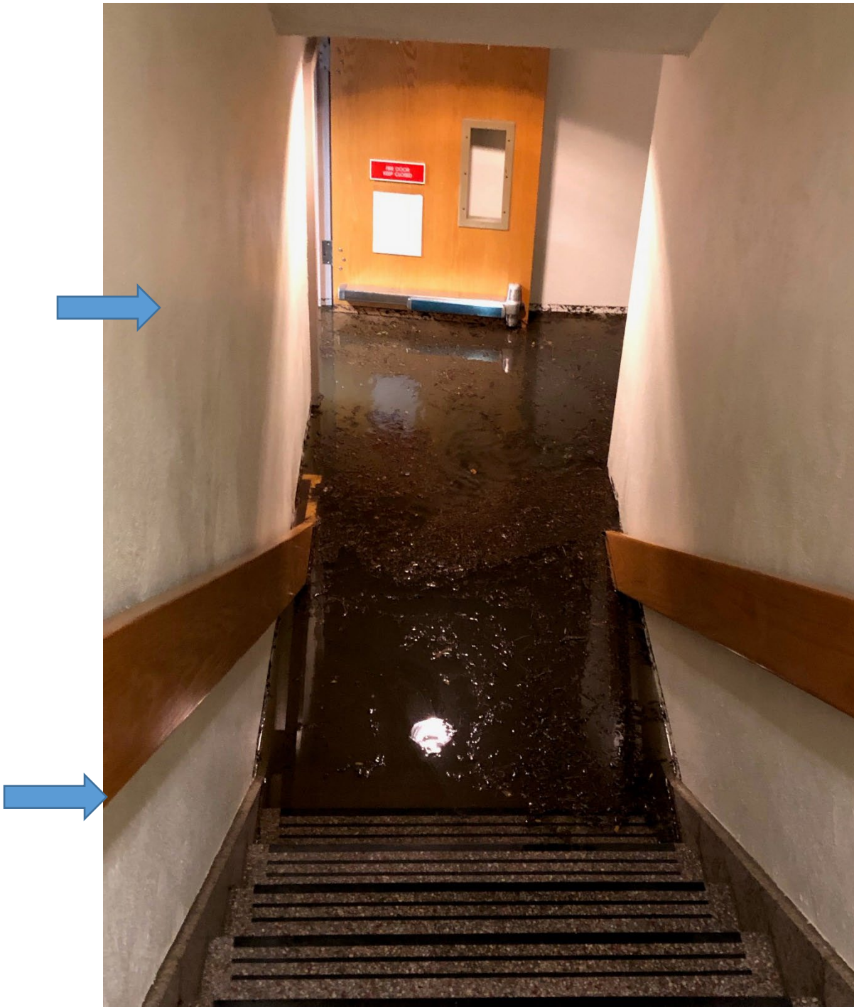
Police Department Basement Stairwell Flood Water Levels
