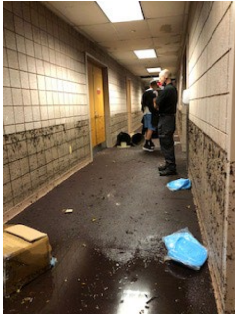
Image showing high water line and soaking floor in basement.
