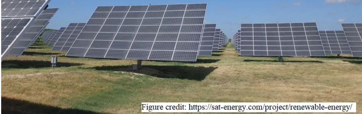
Figure C.4: Example of a dual-axis tracking array. Each unit is motorized rotating East to West through the day, and adjusting their angle of Southward tilt through the seasons of the year, always following the sun, and optimizing the solar energy production annually.
