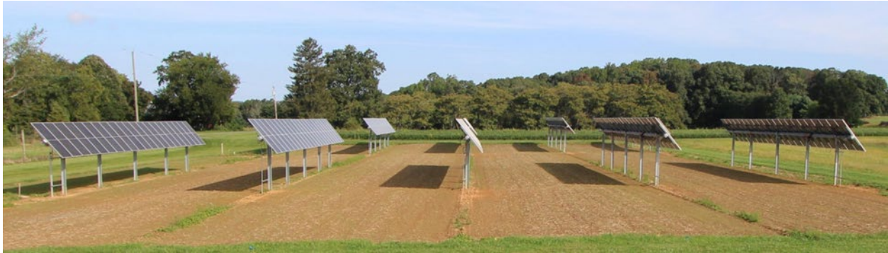
Figure C.2: Single-axis tracking solar array at Rutgers University's Snyder Research Farm, Pittstown, NJ. This array is built in rows that run typically North-to-South and are actuated by motors through the day to point more directly at the sun. Starting in 2023, agricultural research has commenced at this site funded by the US Department of Energy under the FARMS program and with support from the New Jersey Agricultural Experiment Station.
