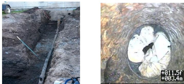
Figure 3 – Photos depicting damage of a waste line and camera view from inside showing a bedsheet obstruction in the line.
