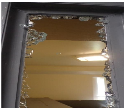
Figure 8 – Broken cell windows caused by an incarcerated person
