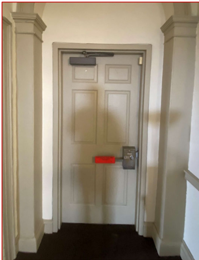
Second Floor Stairway Door, Frame, and Hardware Recommended to be Replaced
