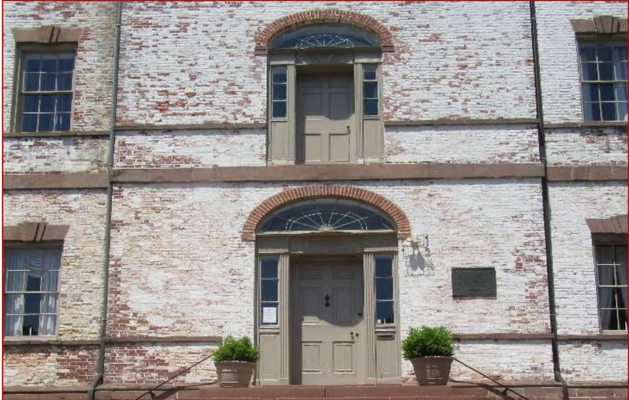
Image of the East Exterior Wall of the North Wing. Note Second Level Exterior Door
