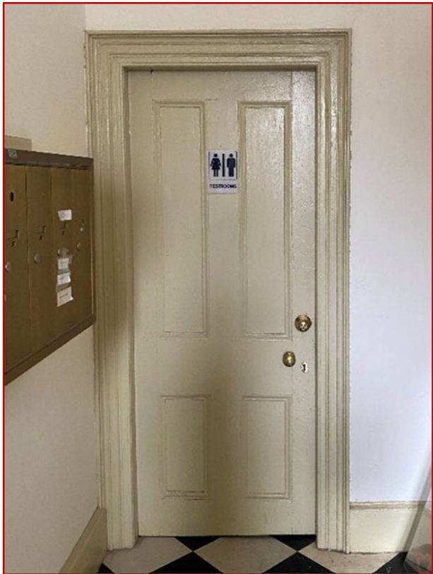
Door, Frame, and Hardware at Toilet Room
