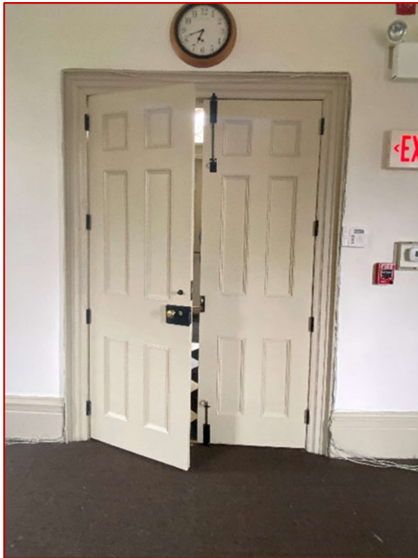
Door, Frame, and Hardware at Office No. 1
