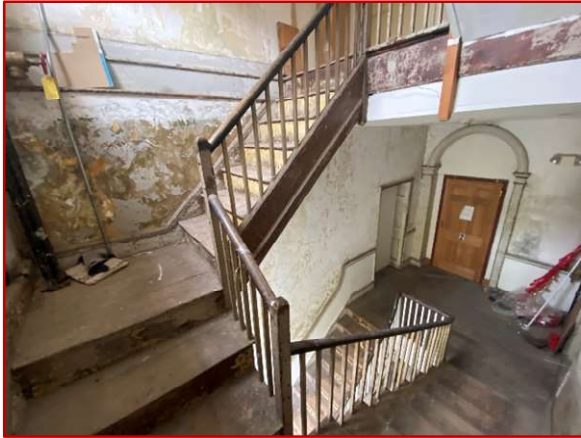
The photograph on the right was taken between the Third Floor and Second Floor of the North Wing. The North Wing Stair is enclosed at both levels
