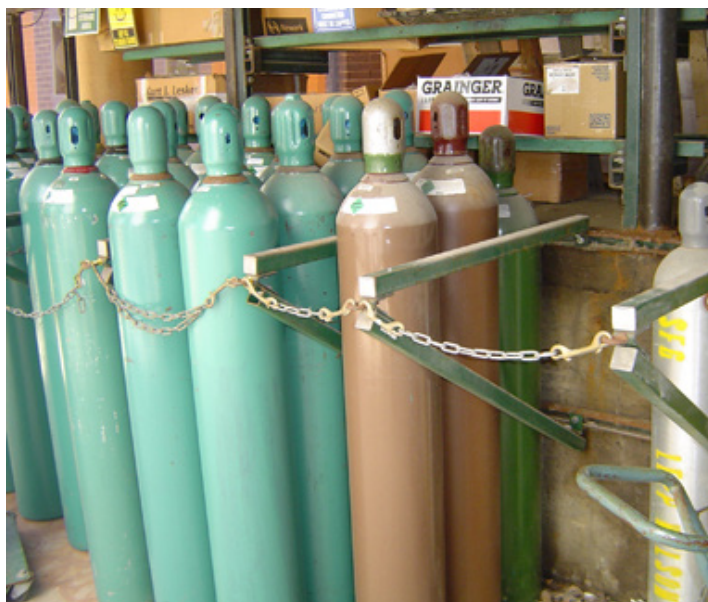
Figure C-32 Hazardous substances are stored or transported in a wide variety of containers. John Lewis.
