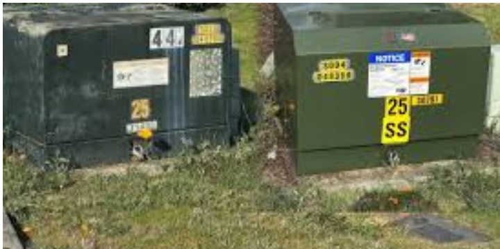
Figure D-6 A Pad Mounted Transformer. From prior edition of NJ FF Addendum from Bob Green PSEG.
