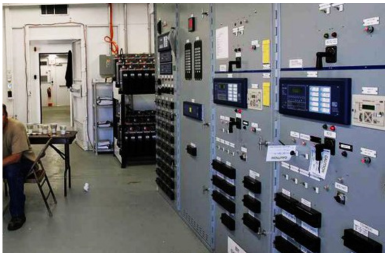
Figure D-8 Sub Station Control Room. From prior edition of NJ FF Addendum from Bob Green PSEG.
