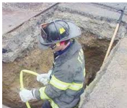
Figure D-19 Never enter a trench/excavation without proper training and NEVER attempt to kink a flowing gas line. Lee Calderio.
