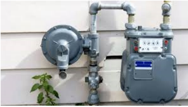
Figure D-15 A typical meter set with a relief valve. John Lewis.
