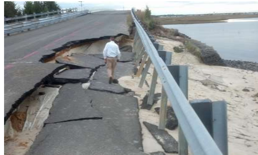
Figure 7: Roadway Damage on Great Bay Boulevard
