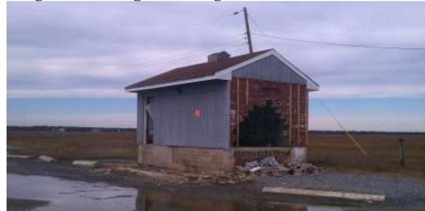
Figure 14: Damaged Building at Parkertown Beach Area
