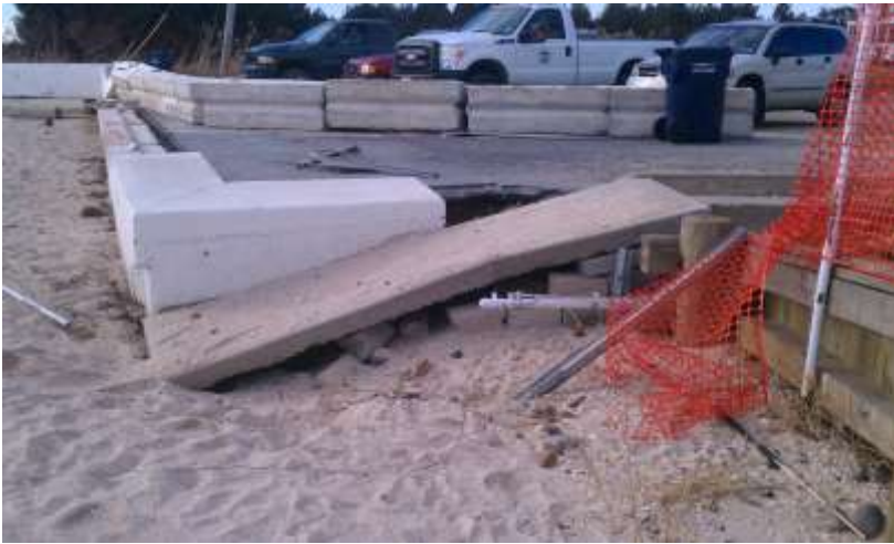
Figure 8: Roadway and Sidewalk Damage at the end of Radio Road
