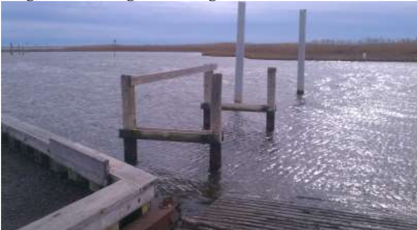
Figure 13: Damaged/Missing Docks at Parkertown Dock
