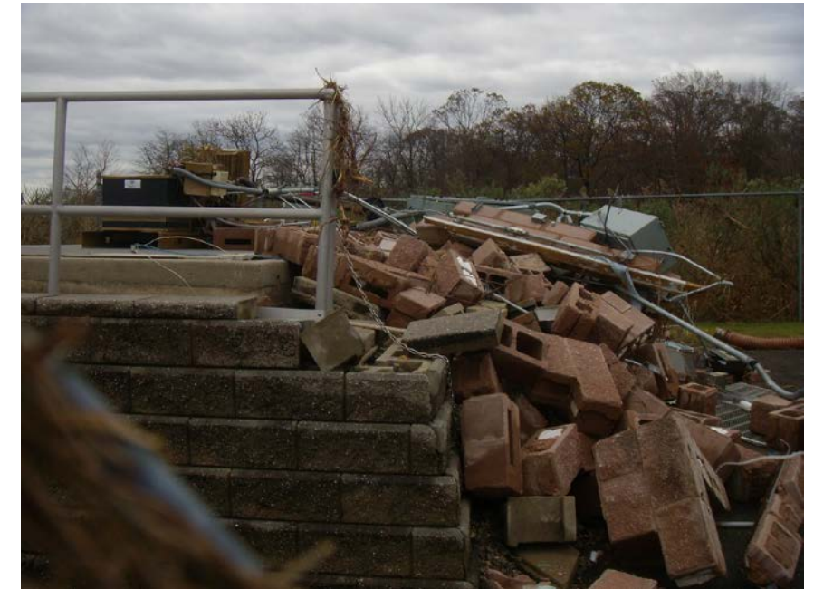
Figure 3: The remnants of Pump Station #4 after Sandy (aberdeennjlife.blogspot.com)
