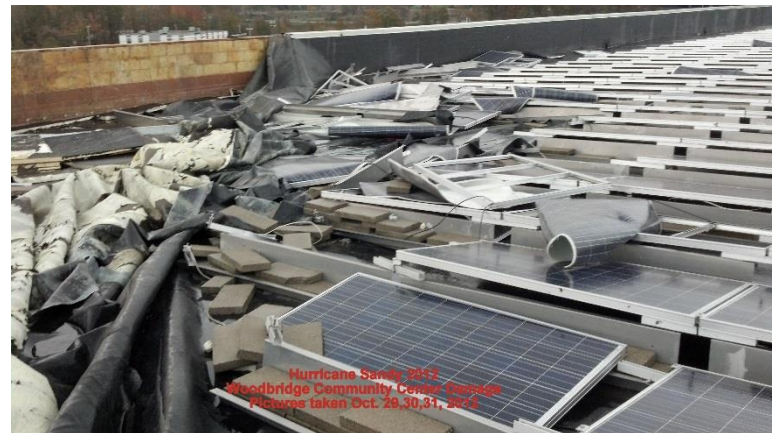
Damaged Roof of Community Center
