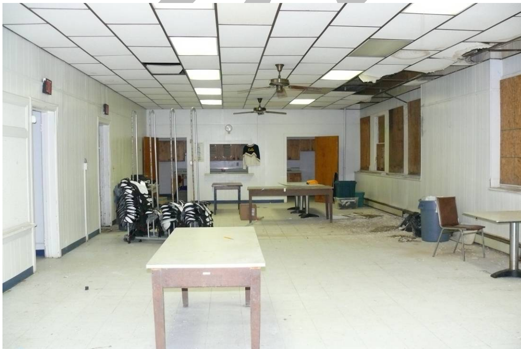
Photo 0010: Overall view of the two classroom spaces with the dividing partition removed; camera facing east.
