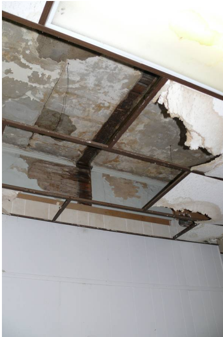
Photo 0011: Partial view of the original ceiling above the acoustical tiles at the first floor, showing scarring from the removed center partition that divided the two classrooms.
