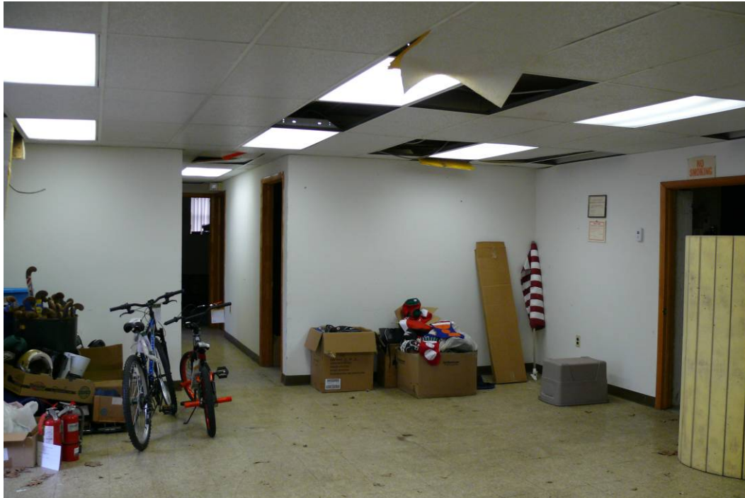
Photo 0007: Overall view of the main basement-level space showing typical late-twentieth-century finishes, which hide some still intact earlier finishes; camera facing west.
