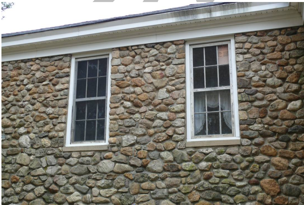
Photo 0002: Close-up view of typical original wood windows at the first floor level.
