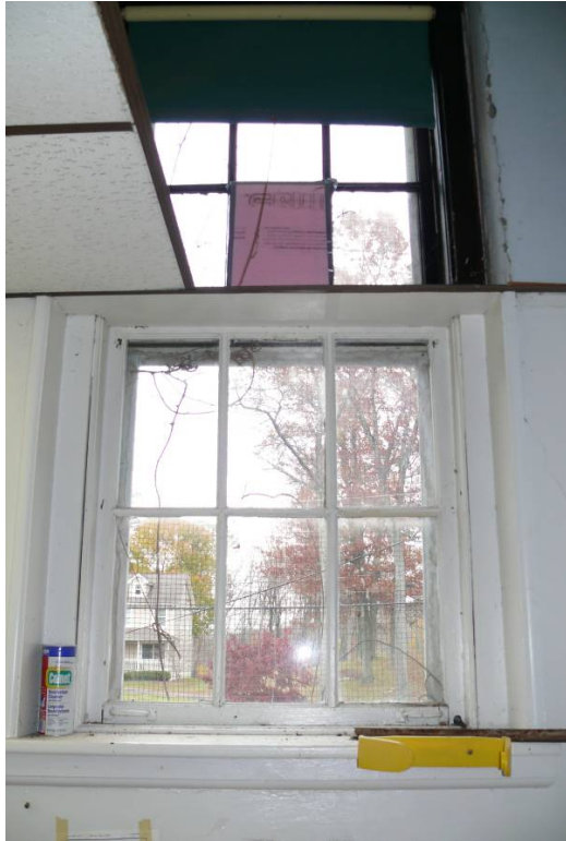
Photo 0013: View showing typical treatment of a first-floor original window where the suspended ceiling divides the upper and lower sashes.
