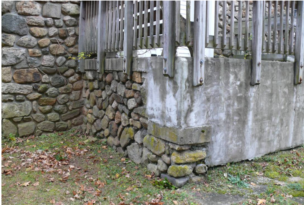
Photo 0003: View of original stone steps that remain but are encapsulated under concrete; camera facing southwest.
