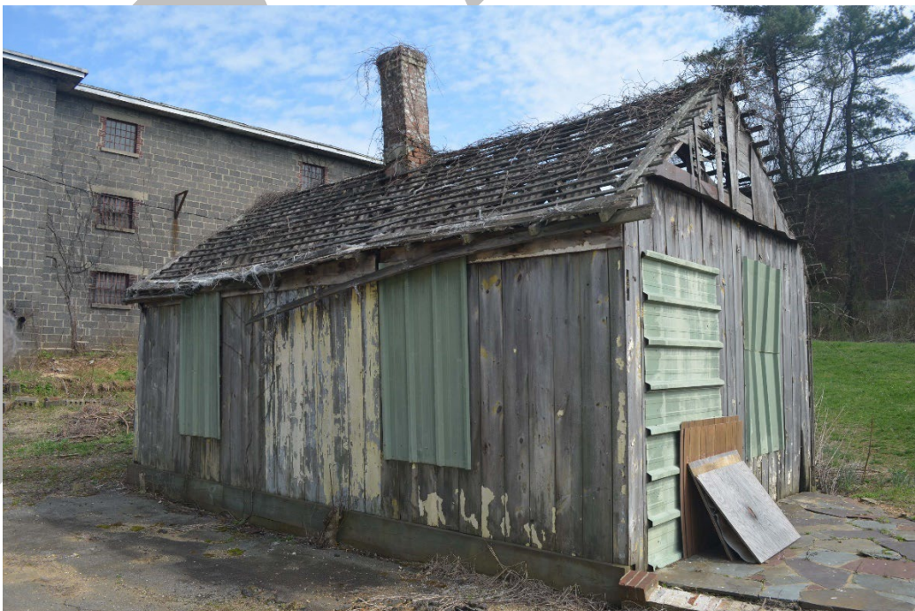
Figure 35. Exterior view of the Office, prior to the roof's collapse, west (primary) façade and north elevation, camera facing southeast (April 11, 2019).
