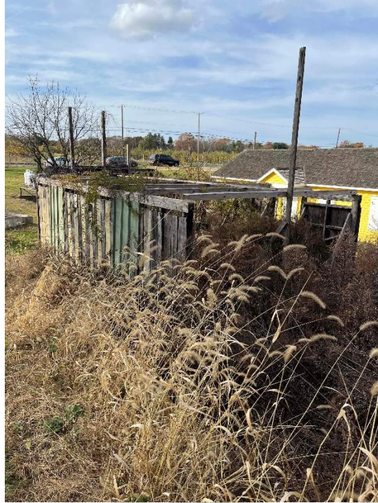
Photo 29. Exterior view of the Office, collapsed east elevation with temporary bracing and vegetation growth, camera facing northwest (November 17, 2023).
