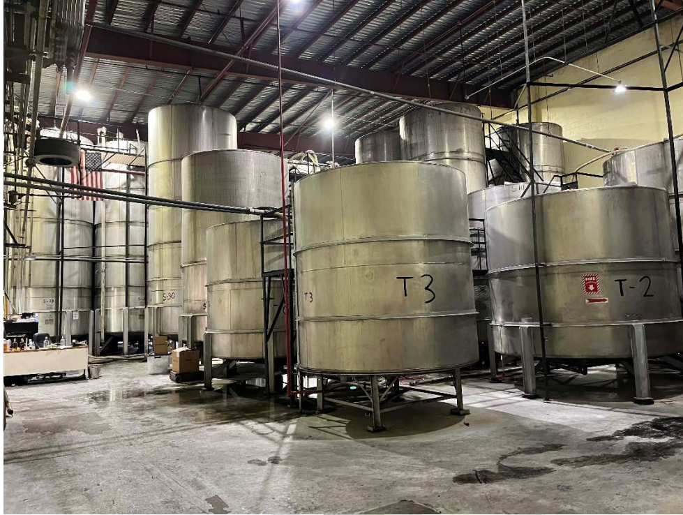
Photo 61. Interior view of the Current Bottling Plant, modern fermentation tanks, camera facing northeast (November 17, 2023).
