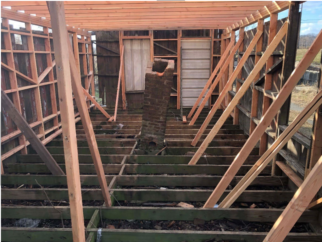
Figure 37. Interior view of the Office, after east elevation roof collapse prior to current vegetation growth, camera facing west (January 14, 2020).
