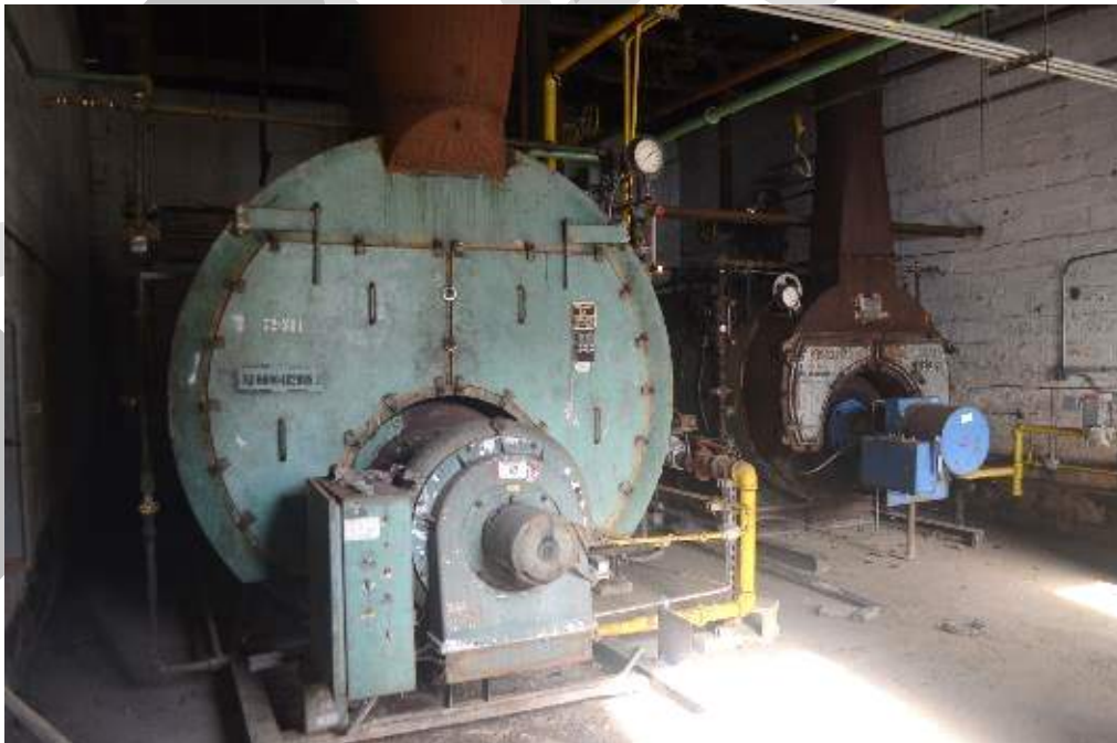
Photo 40. Interior view of the boiler room in Volume D attached to the Still House, including an original boiler (right), camera facing northeast (November 17, 2023).
