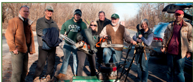
Not afraid to get his hands dirty, Michael chaired the Petty's Island trail construction crew.
