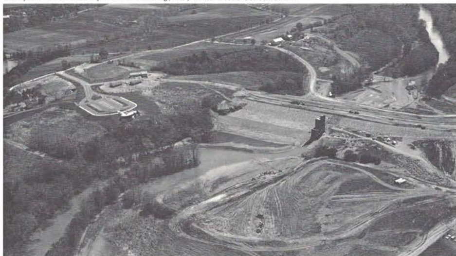
Corps of Engineers photograph shows Blue Marsh reservoir, on a Schuylkill River tributary west of Reading, Pa., in advanced construction.
