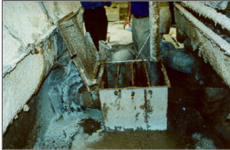
Figure 1 Photo of paper pulp chest hatch (Safety bars were installed after the incident)
