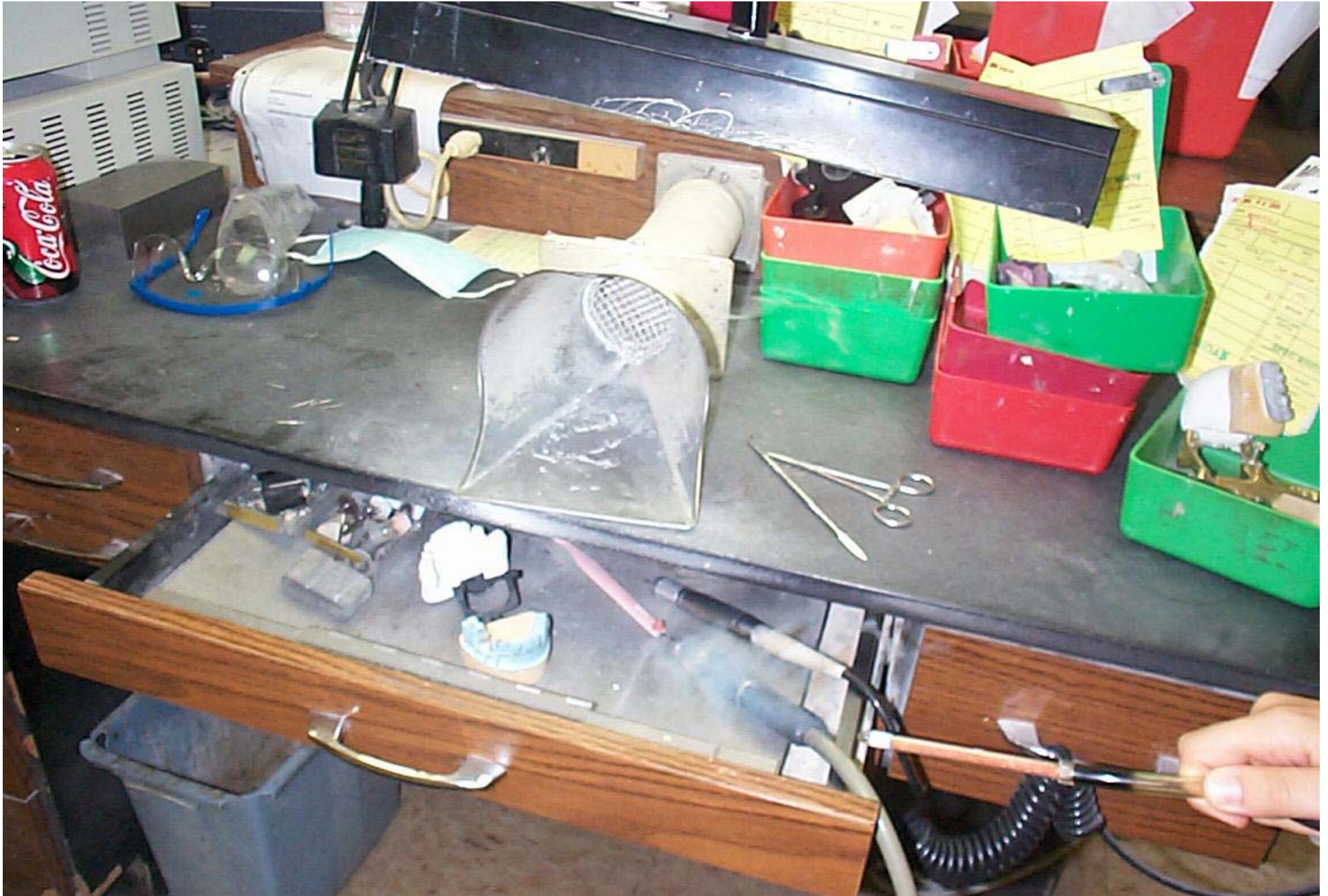
work station local exhaust ventilation
