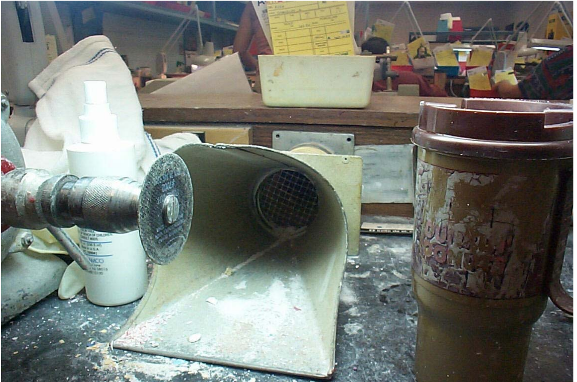
local exhaust ventilation hood
