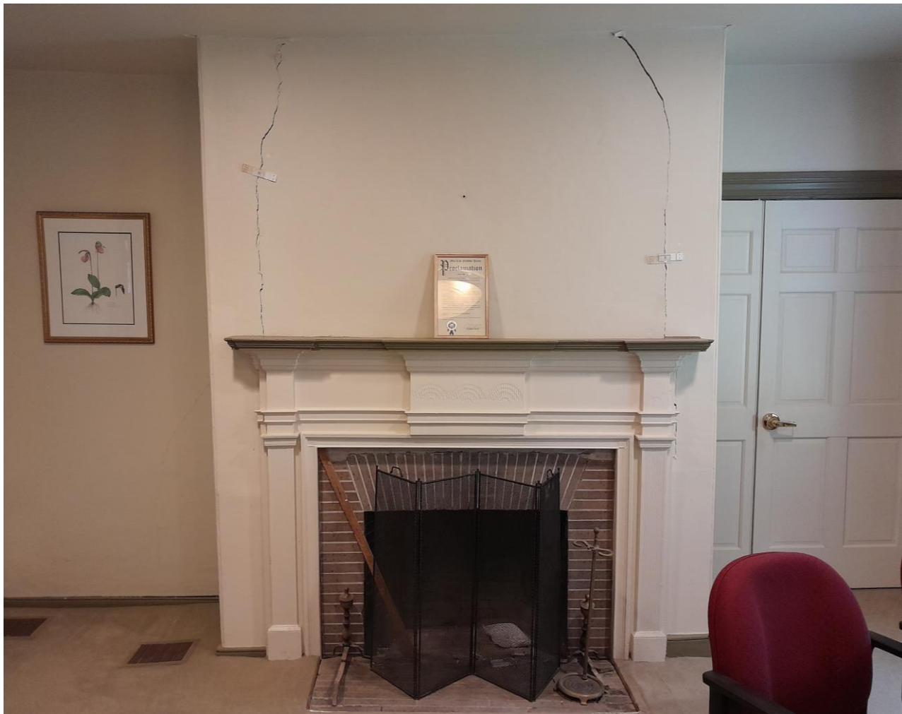
Cracks in wall due to slumping chimney
