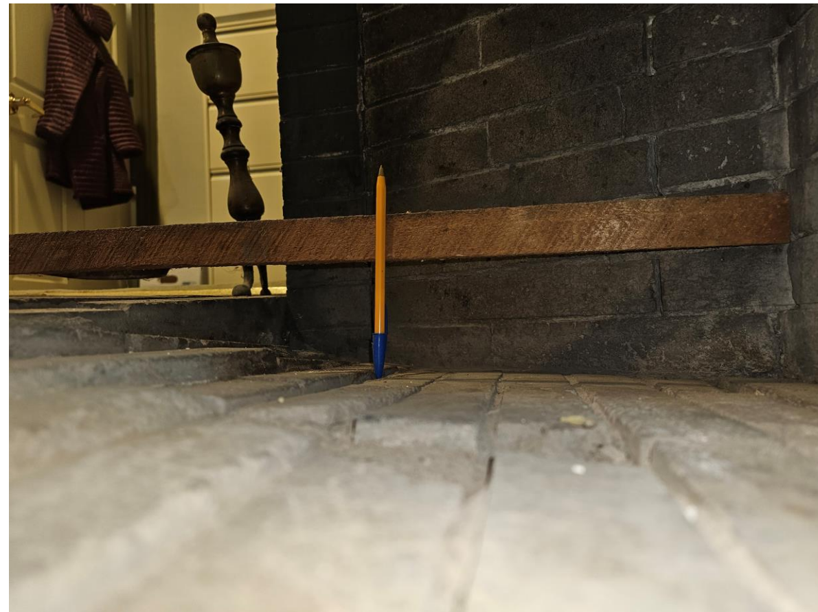
Inside fireplace showing slumping
