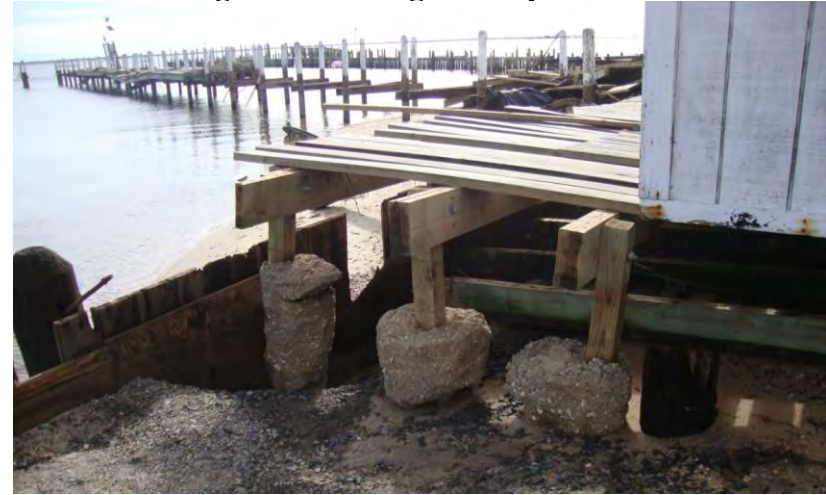
Figure 11: Damages at Bryant Park
