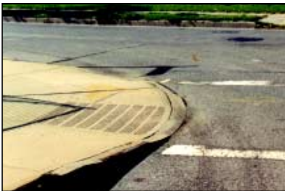
Figure 2.32: Fifteen-foot mountable corner with truck tire tracks, Queens, New York.
