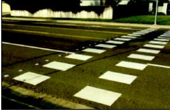
Figure 2.22: High visibility pavement markings, New York, New York (top) and Sacramento, California (bottom).
