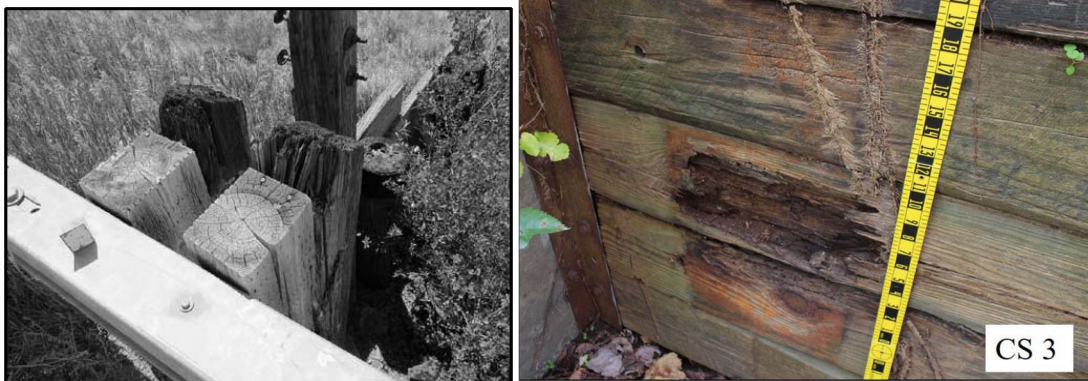
Figure C.4.2.4-1: Decay in Timber Railing Posts (left) and Defect 1140-Decay/Section Loss Condition State 3 (right).
