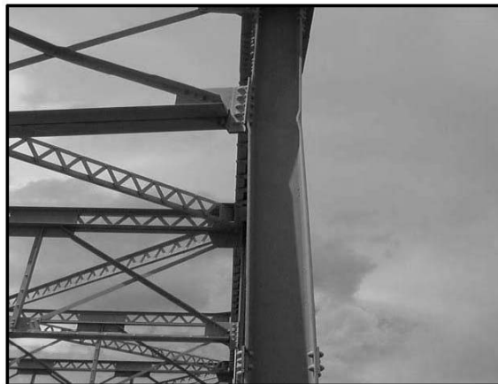
Figure C.6.2.2-1: Sway Bracing Impact Damage in Span 1
