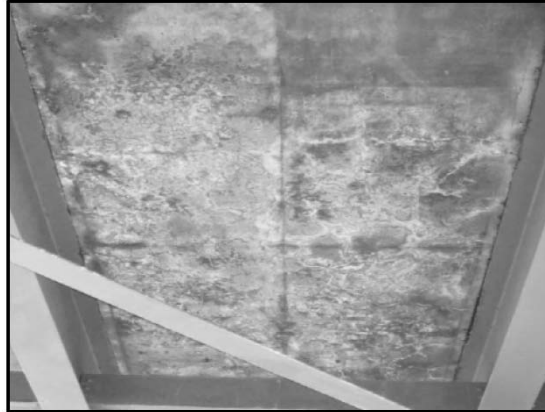
Figure C.6.2.1-1: Efflorescence on the Underside of the Deck in Span 1
