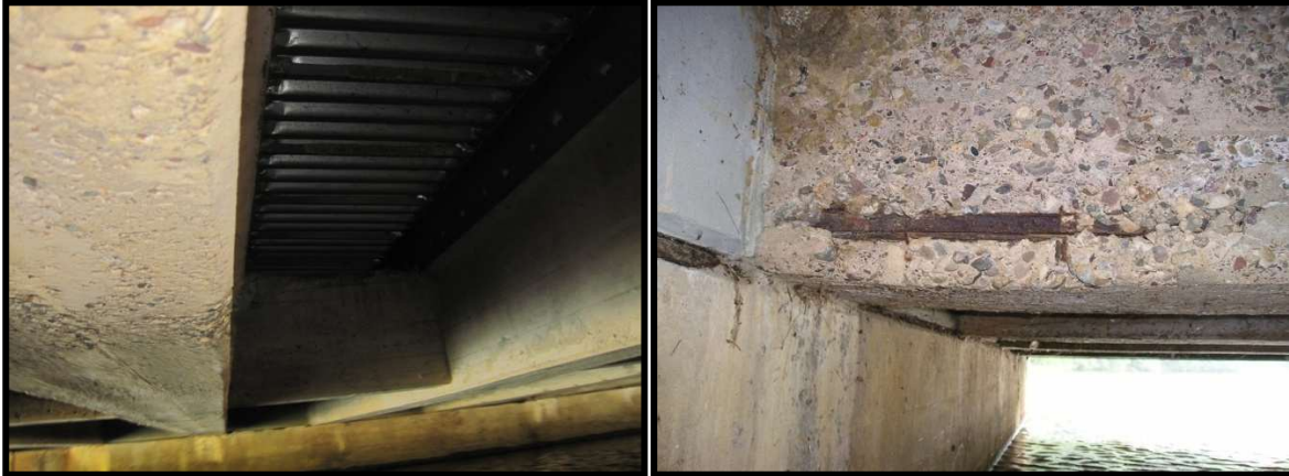
Figure C.1.2.5-1 – Typical Concrete Encasement Condition (Left), Localized Spalling of Concrete Encasement (Right)
