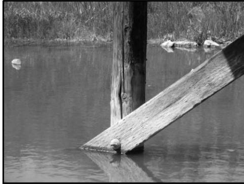
Figure C.4.2.3-1 – 7-inch Deep Check in Right Exterior Pile of Bent 2
