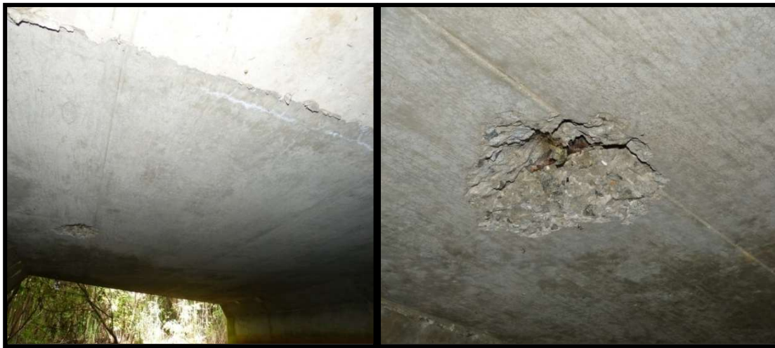
Figure C.3.2.1-1 – Spalls with exposed Rebar at Roof Slab
