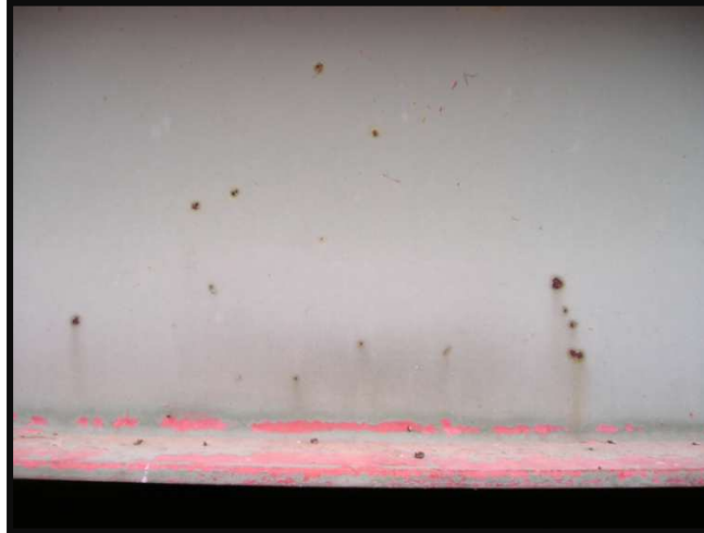
Figure C.1.2.3-1 – Fascia Beam Paint Condition
