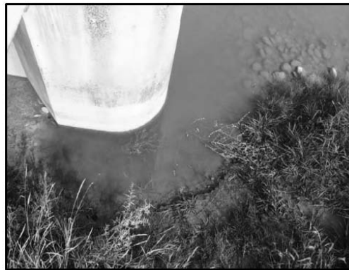
Figure C.6.2.7-1: Scour Hole at the Upstream End of the Pier Wall
