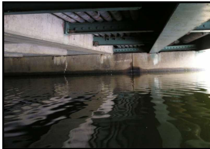
Figure C.1.2.6-1 – Typical Efflorescence Staining
