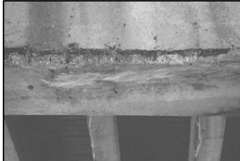
Figure C.5.2.5-1: Spall, underside of Pier 2 cap
