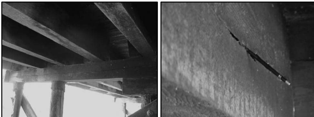
Figure C.4.2.2-1 – 1-in. Deep Check in Bent Cap at Bent 2
