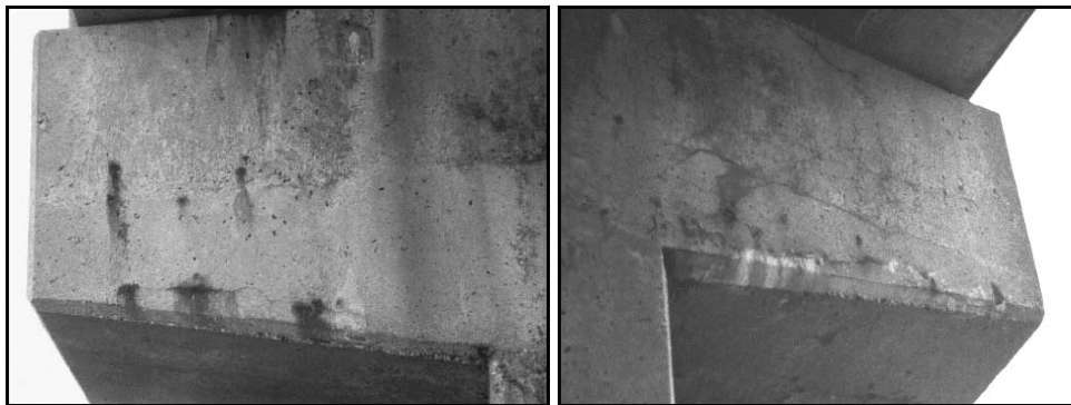
Figure C.5.2.6-1: 0.04 in. width cracks with rust staining in the cantilevers of the Pier 3 cap
