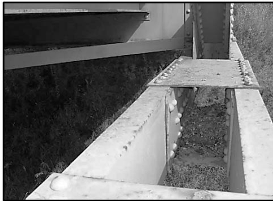
Figure C.6.2.3-1: Freckle Rust, Typical, Both Trusses, Both Spans
