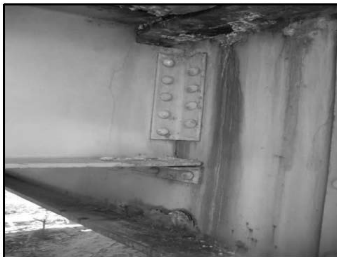
Figure C.6.2.4-1: Corrosion at Floor Beam Ends
