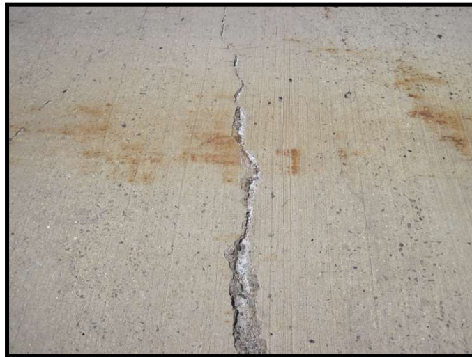
Figure C.1.2.2-1 – Wide Transverse Crack on Approach Slab
