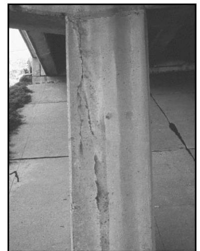
Figure C.5.2.7-1: 3/16 in. width vertical crack in left column of Pier 4
