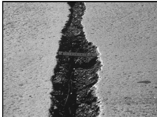
Figure C.5.2.4-1: Deep spalls in the deck adjacent to the joint seal at Pier 3
