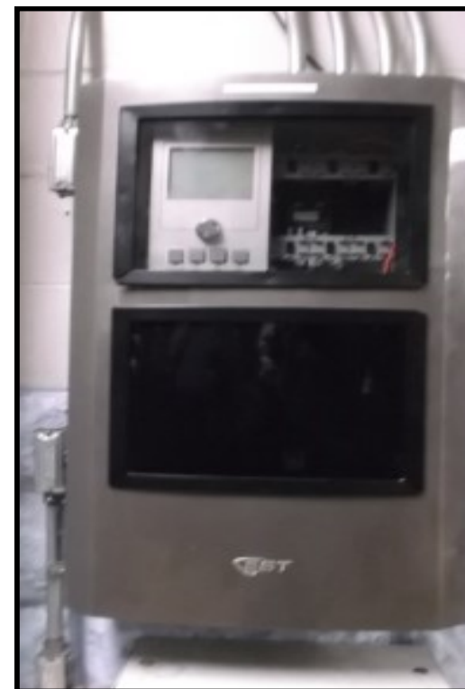
Not Operational Alarm Annunciator
