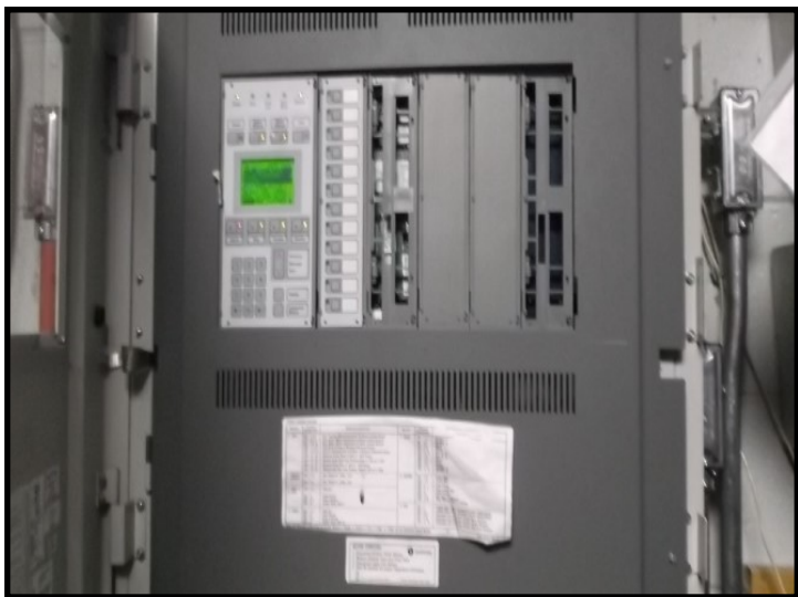
Main Fire Alarm System Panel
