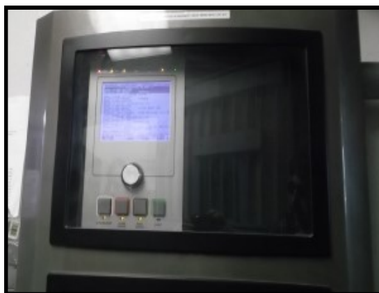
Operational Alarm Annunciator
