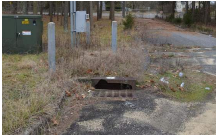
Figure 2.11: Example of Damaged Inlet
