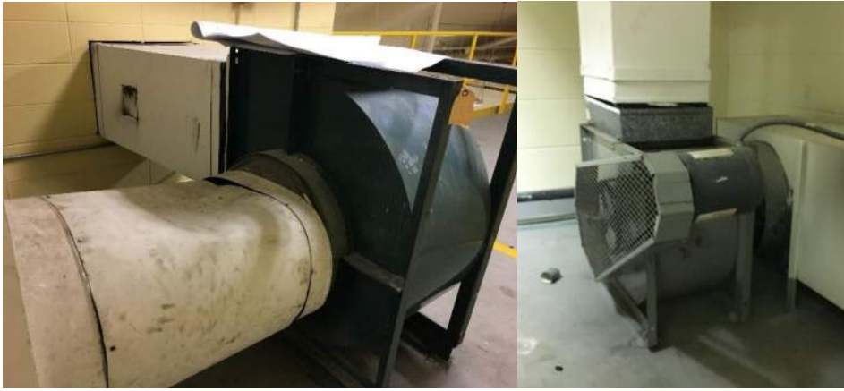
Figure 4.7 Existing space mounted exhaust fans
