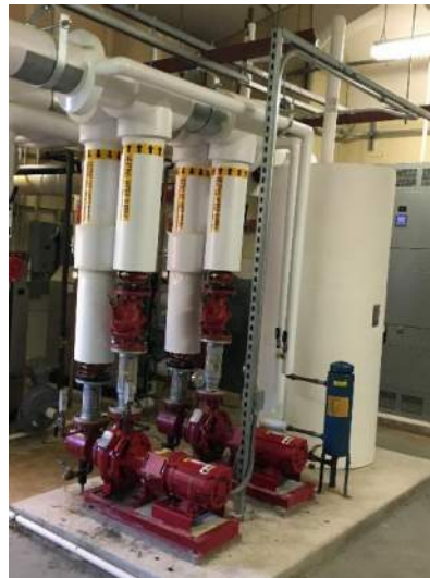
Figure 4.2 Existing two hot water circulating pumps, an expansion tank and a chemical pot feeder
