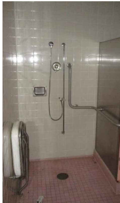
Figure 6.8 - Plumbing Fixtures, Shower
