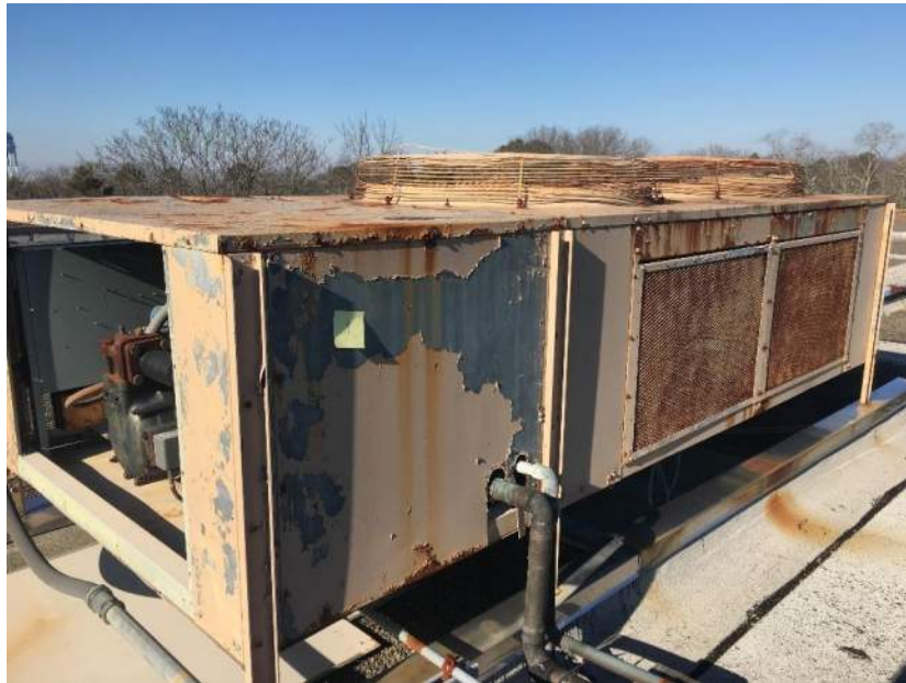
Figure 4.5 Existing roof mounted condensing unit
