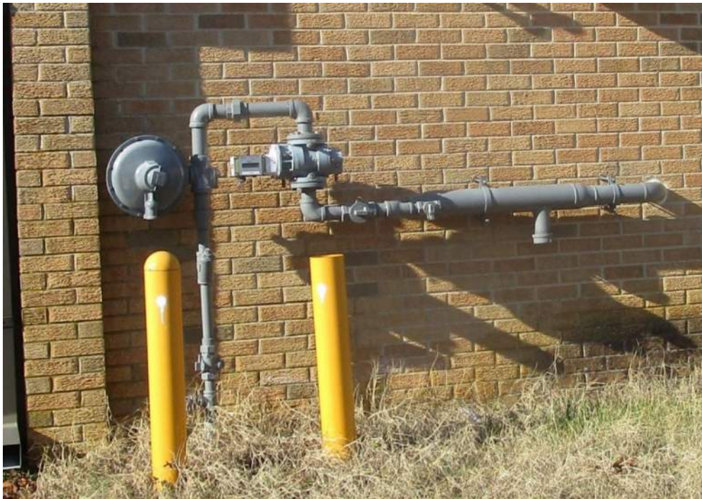
Figure 6.10 - Natural Gas Meter and Regulator
