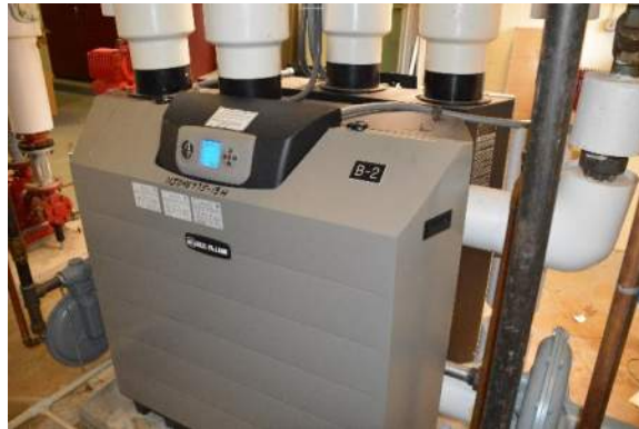
Figure 4.1 Existing gas-fired, heating hot water condensing boilers
