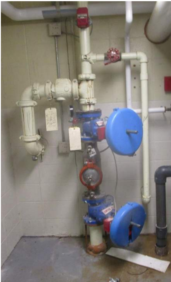
Figure 7.1 - Fire Protection Backflow Preventer Gage
