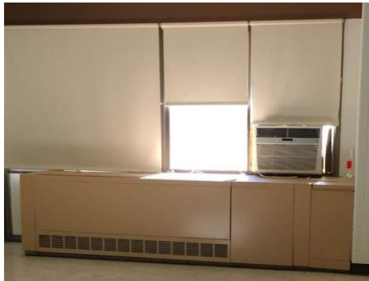
Figure 4.6 Existing unit ventilator and window type air conditioning unit
