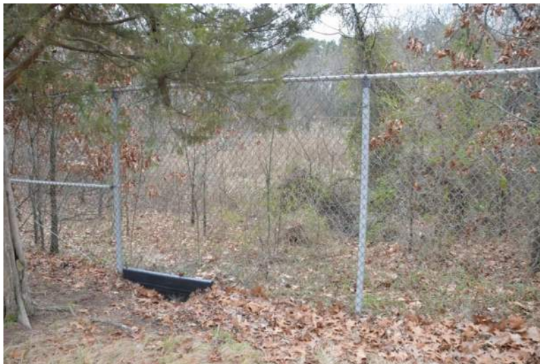
Figure 2.12: Unmaintained Infiltration Basin
