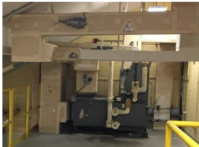
Figure 4.4 Existing air handling unit in the Mezzanine
