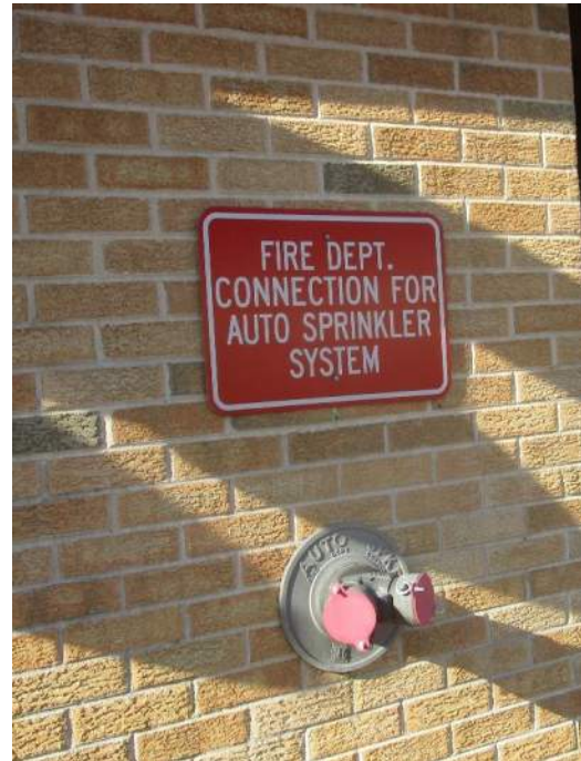
Figure 7.4 - Fire Department Connection
