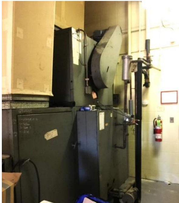
Figure 4.3 Existing air handling unit in Mechanical Equipment Room 129
