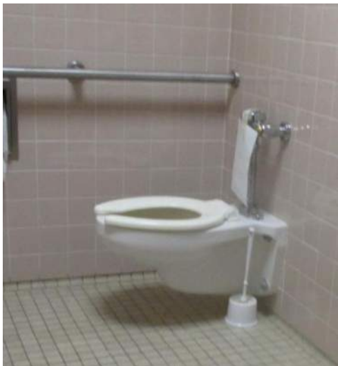
Figure 6.4 - Plumbing Fixtures, Water Closet
