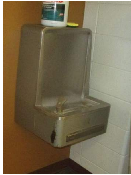
Figure 6.6 - Plumbing Fixtures, Fountain
