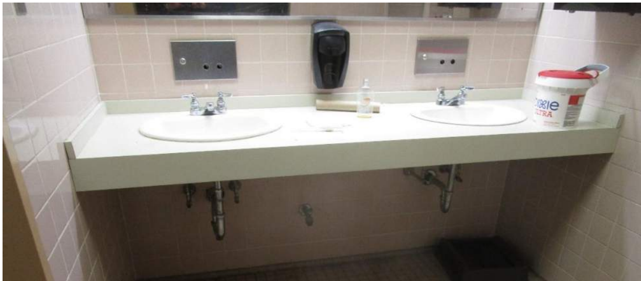
Figure 6.2 - Plumbing Fixtures, Lavatories
