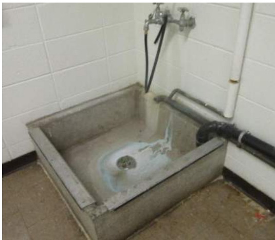
Figure 6.7 - Plumbing Fixtures, Mop Sink
