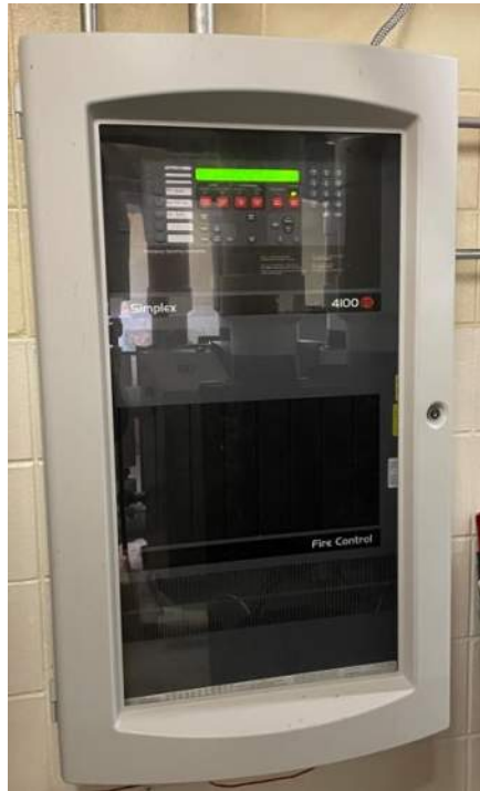
Figure 8.1 - Main Fire Alarm Control Panel
