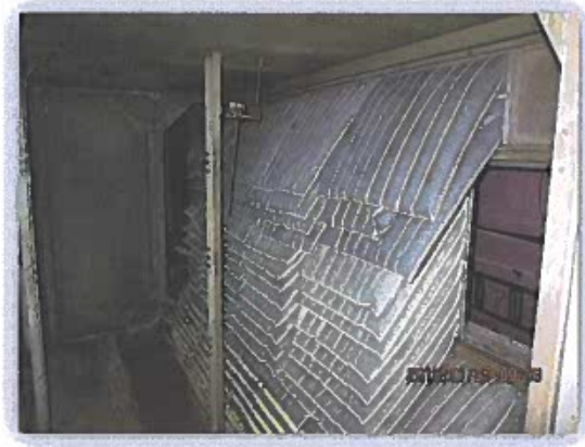
Figure 8: Blocked Outside Air
