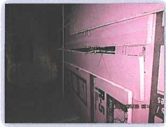
Figure 7: Blocked Outside Air
