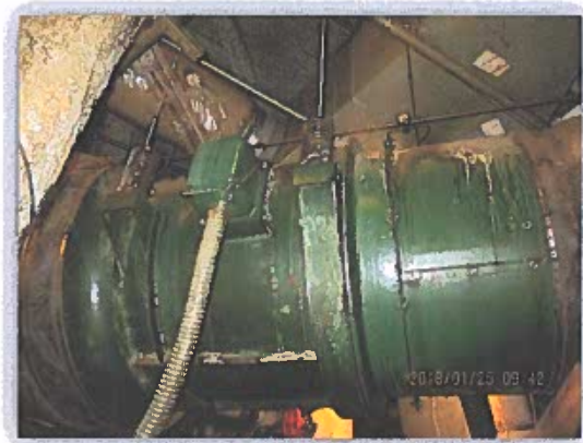
Figure 4: Existing Exhaust Fan
