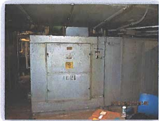
Figure 3: Existing Air Handling Unit (AC-21 shown)
