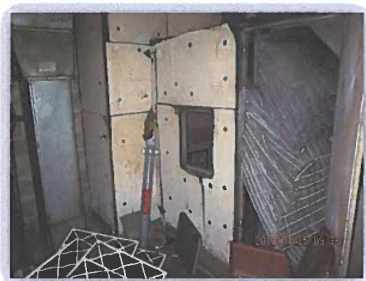
Figure 5: Existing Air Handling Bag Filters
