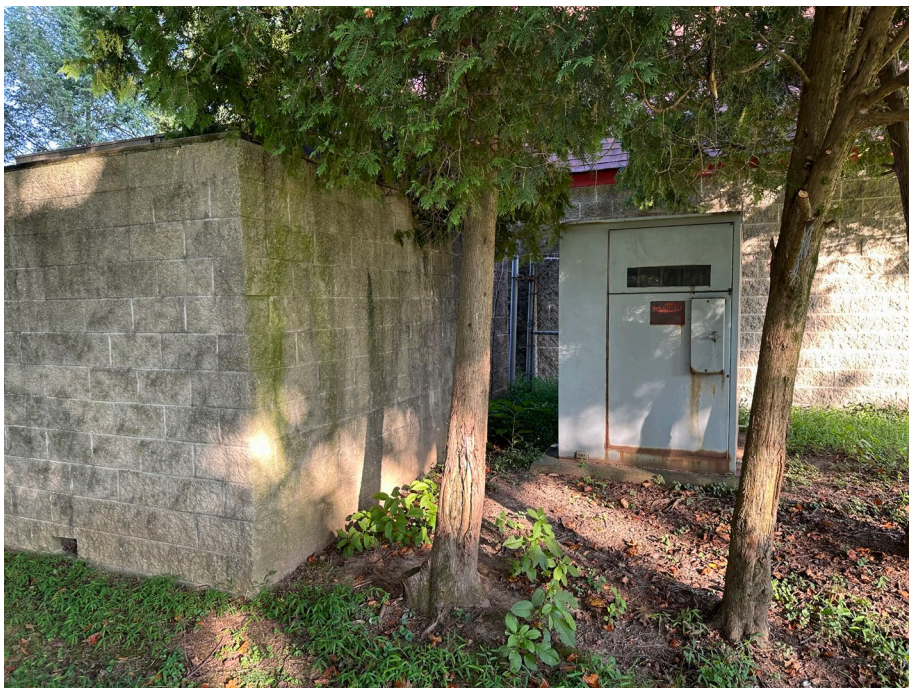
Existing outdoor combination 5kV primary switch and transformer
