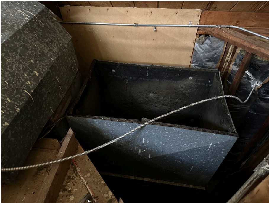
Open-end return duct in chase behind the electrical room
