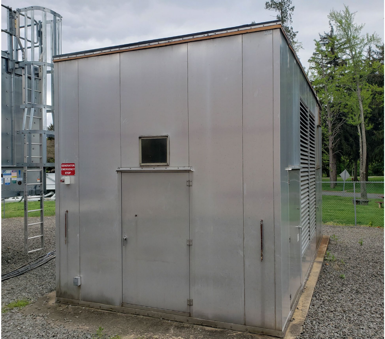
EXISTING GENERATOR ENCLOSURE
