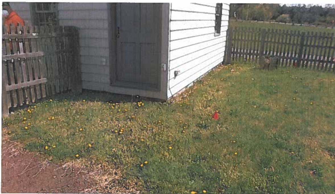
Entrance to Children's Museum. ADA access required here.
