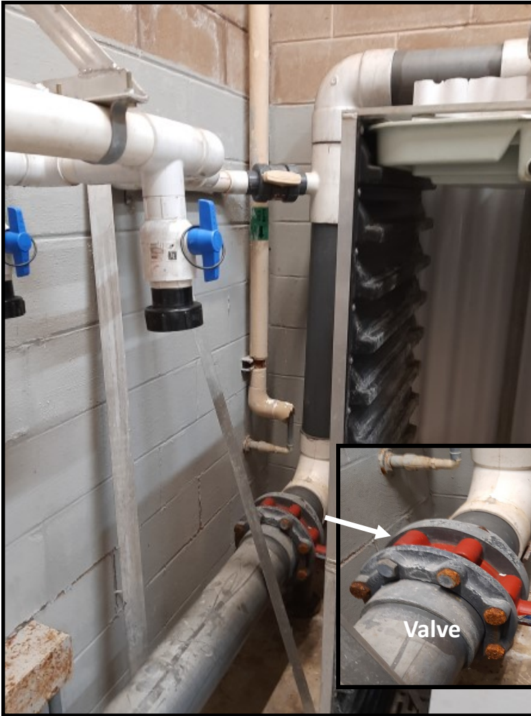
Incubator Room Piping & Valve
