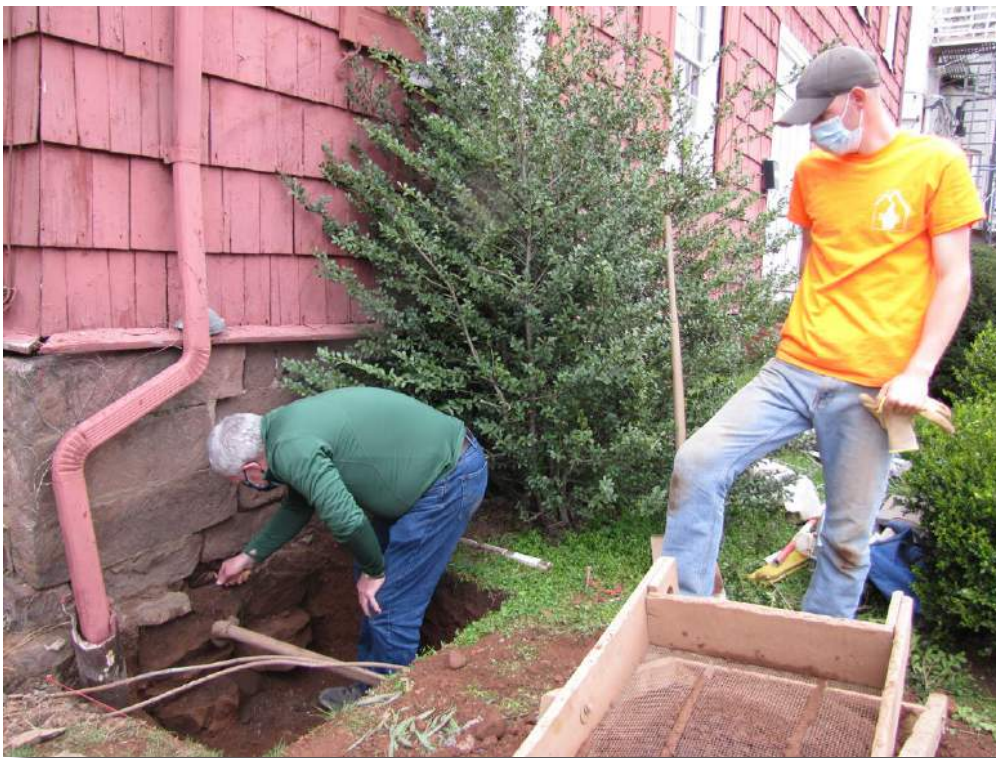
Plate 4.3: Structural engineer, Tom Langan, inspecting the extent of damage to the foundation with the drainage gutter, the oil tank pipe, and the copper piping visible to his left.
