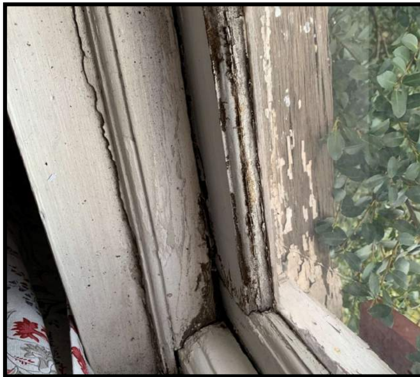
Damaged/Deteriorated Interior Meeting Rail
