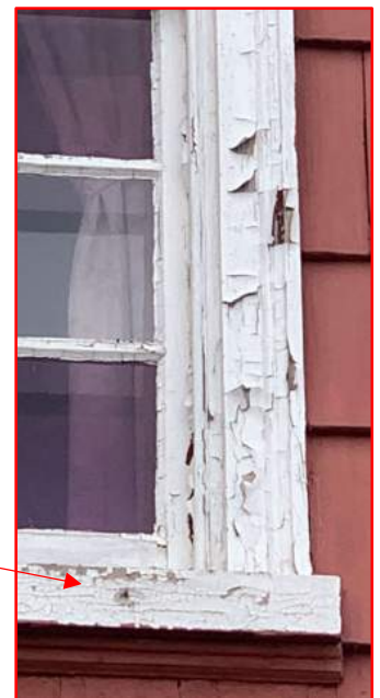
Degradation of Exterior Paint
