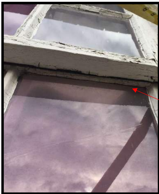
Damaged Meeting Rail
