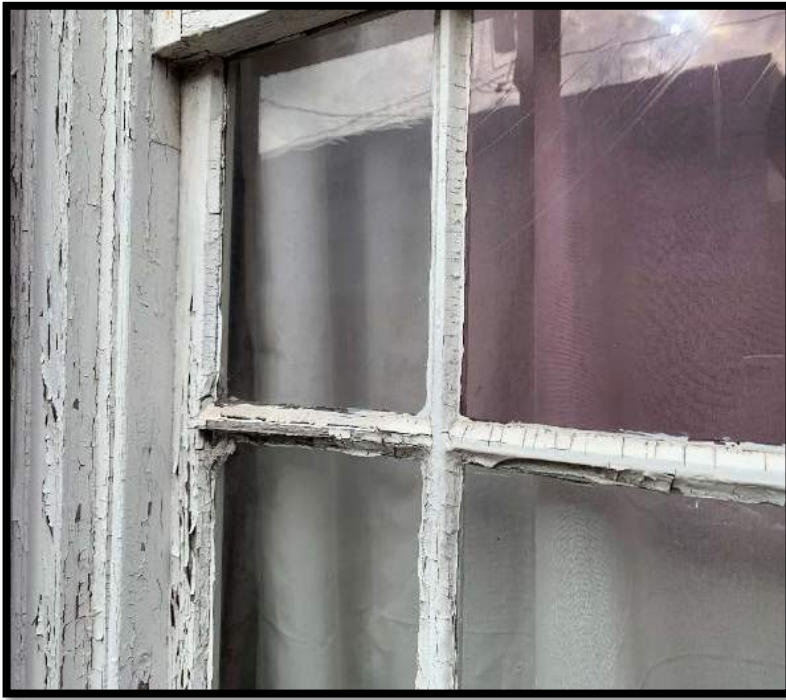
Damaged Muntin at Exterior
