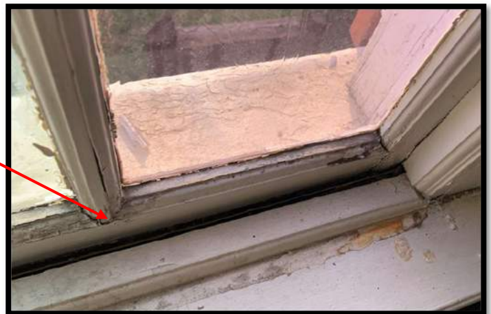
Gap Between Sill and Window
