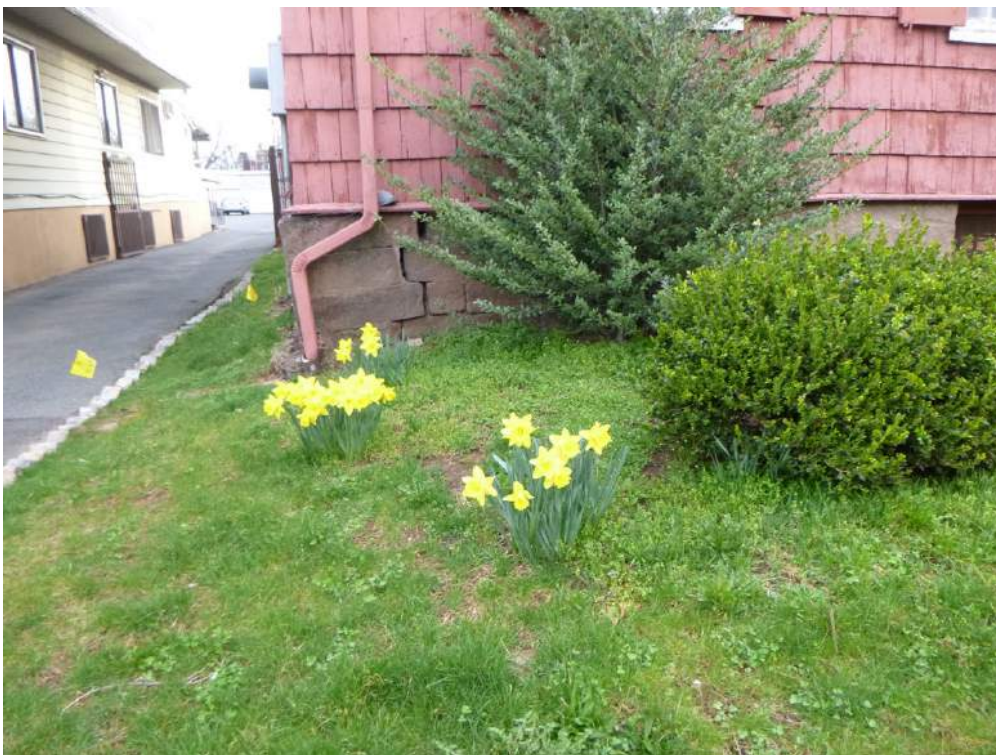
Plate 4.2: Close-up view of the project location showing the damaged foundation and the current location of the drainage gutter, marked-out utility, and landscaping elements.
