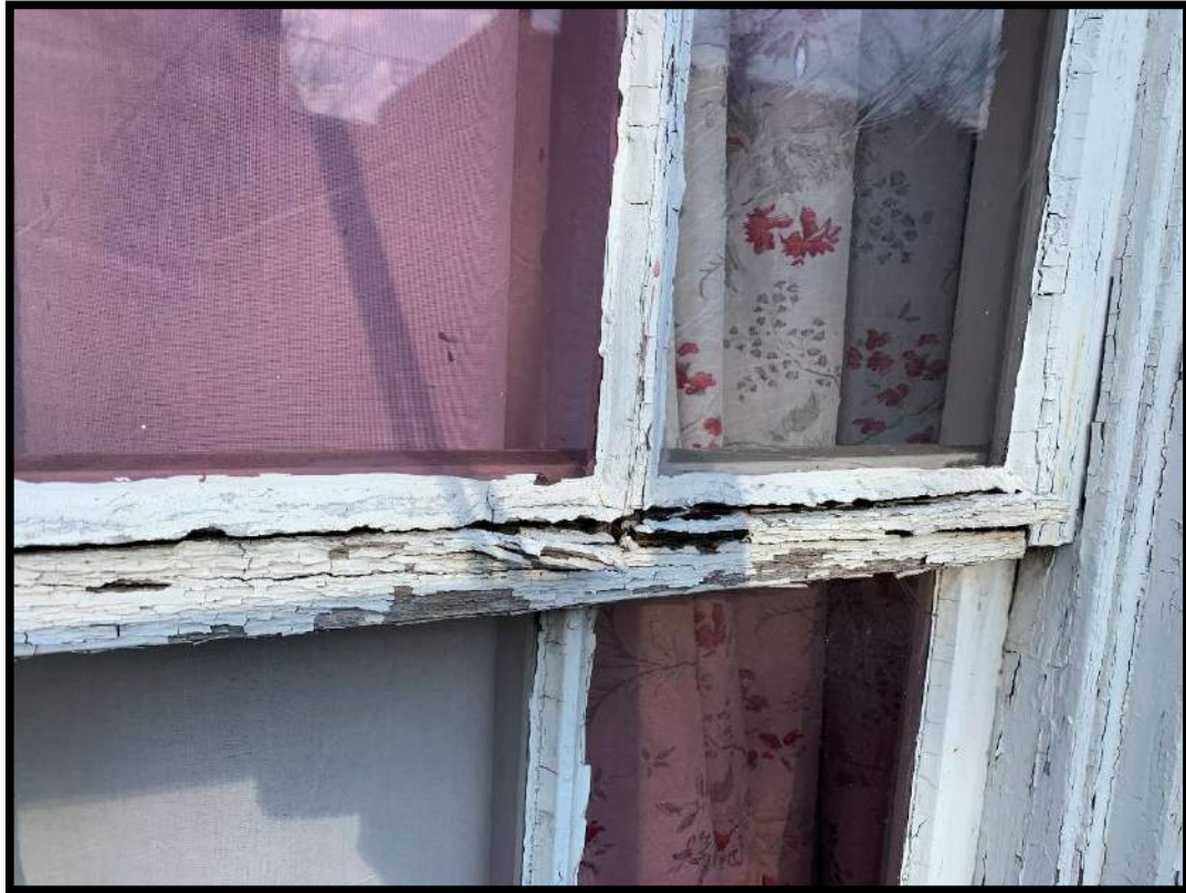
Damaged/Deteriorated Exterior Meeting Rail
