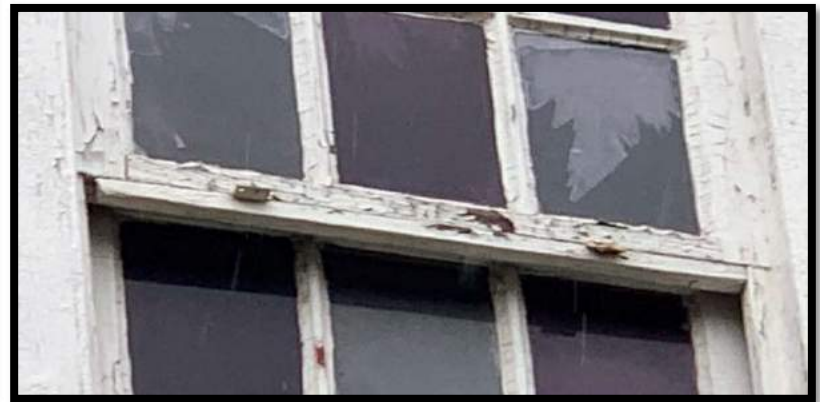
Damaged Meeting Rail
