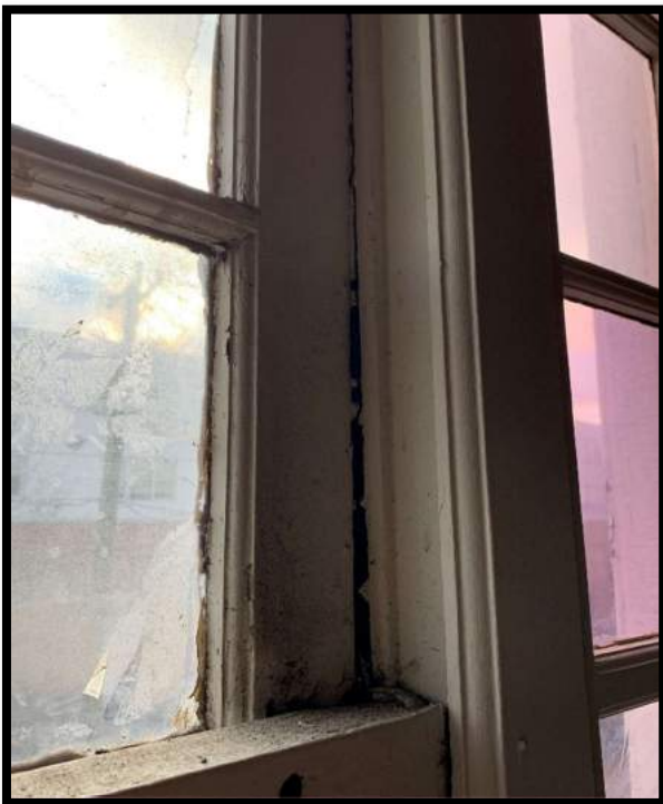
Gap at Window Frame
