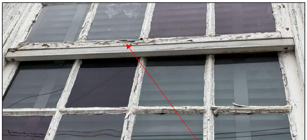
Damaged Meeting Rail and Support Block
