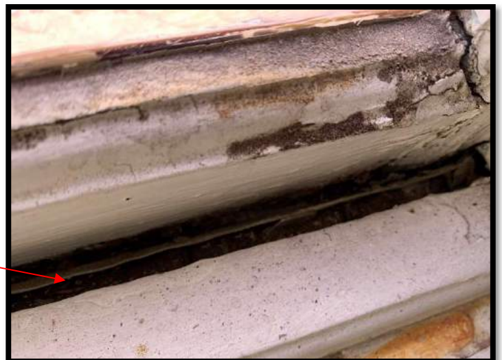
Gap Forming at Interior Windowsill
