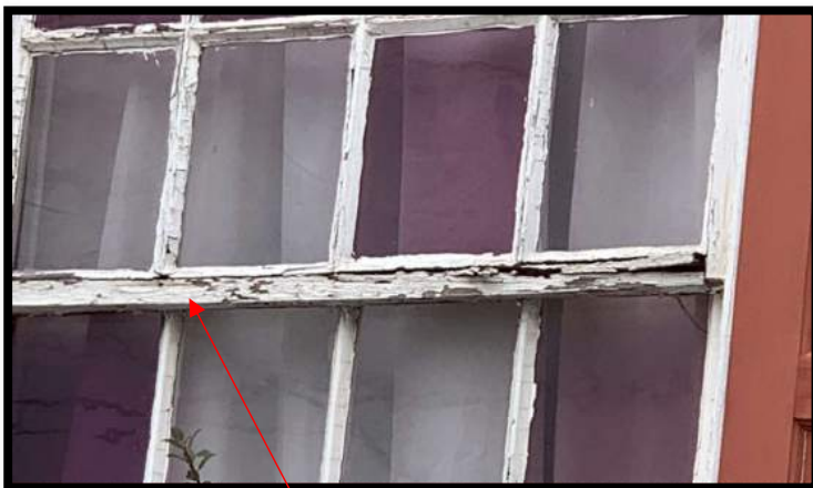
Destroyed Meeting Rail
