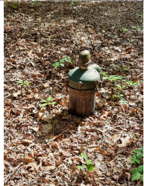
Water Well Head
