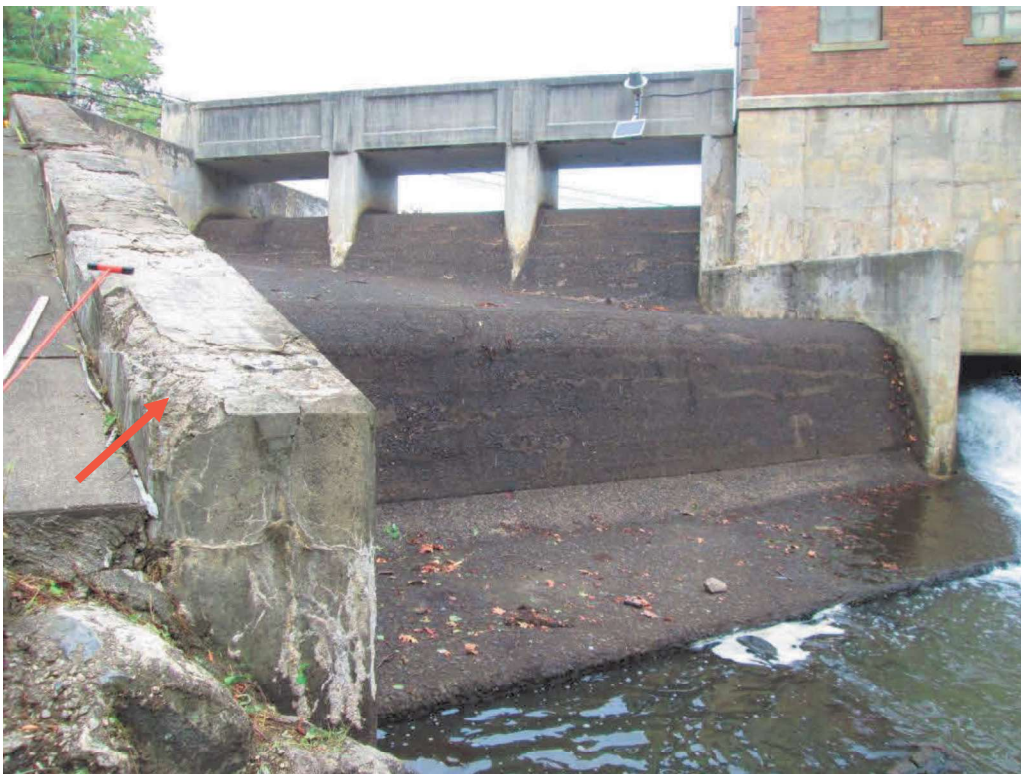
Photo No. 22: Downstream face and apron of the 30-foot long spillway weir looking upstream. Note the cracks and spalls in the previous repair material in the downstream right wing wall.
