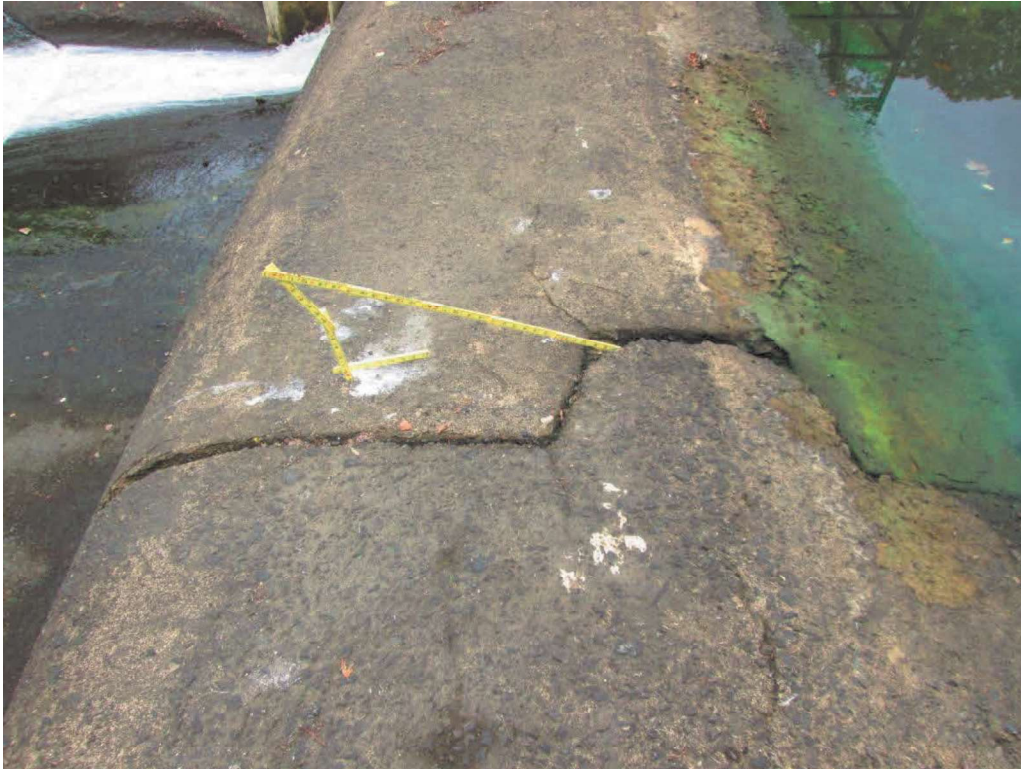
Photo No. 27: Closeup of the eroded right keyway joint in the 90-foot long spillway weir.
