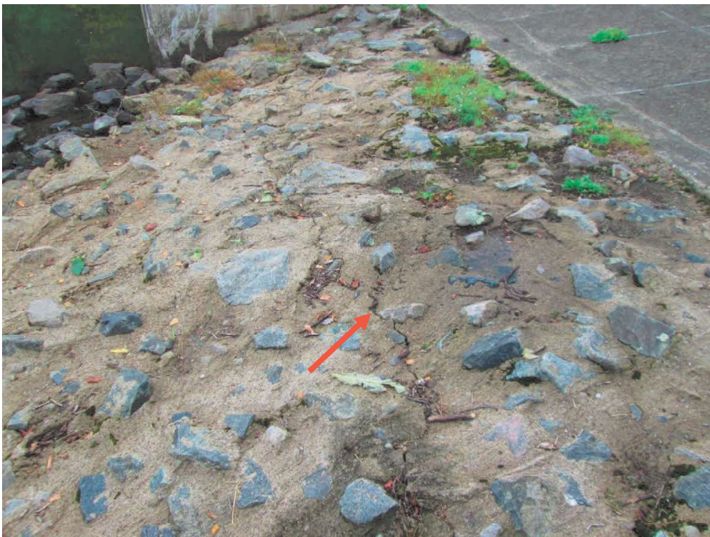
Photo No. 6: Closeup of grouted riprap upstream slope looking left. Note the various cracks throughout the grout.
