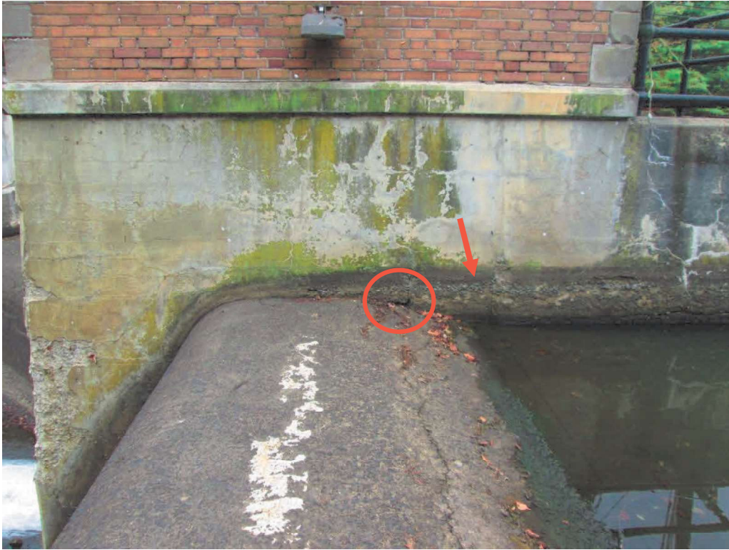
Photo No. 37: Left sidewall of the gatehouse at the contact with 90-foot long spillway weir. Note the horizontal crack and void in the wall.
