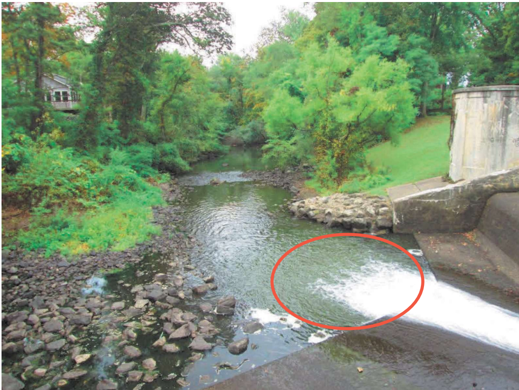
Photo No. 46: Downstream channel from the 90-foot long spillway crest. Note the approximate location of the downstream scour hole.
