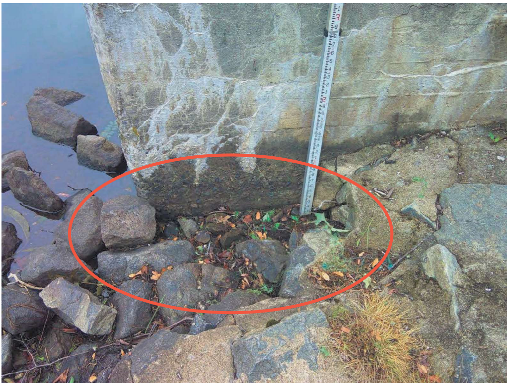
Photo No. 8: Area of displaced grouted riprap along the right side spillway training wall.
