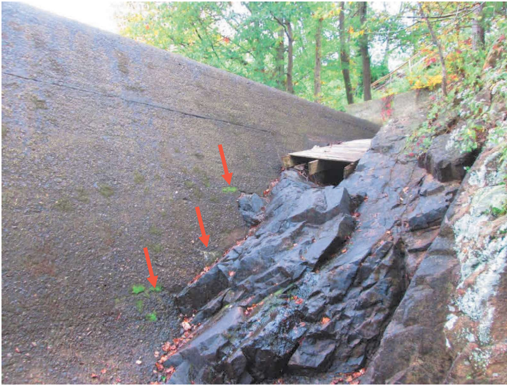
Photo No. 33: Contact of the downstream face of the 90-foot long spillway weir with rock at the left abutment. Note the horizontal cracks/lift joints in the downstream face of the weir. Note the dock lodged on the rock abutment.
