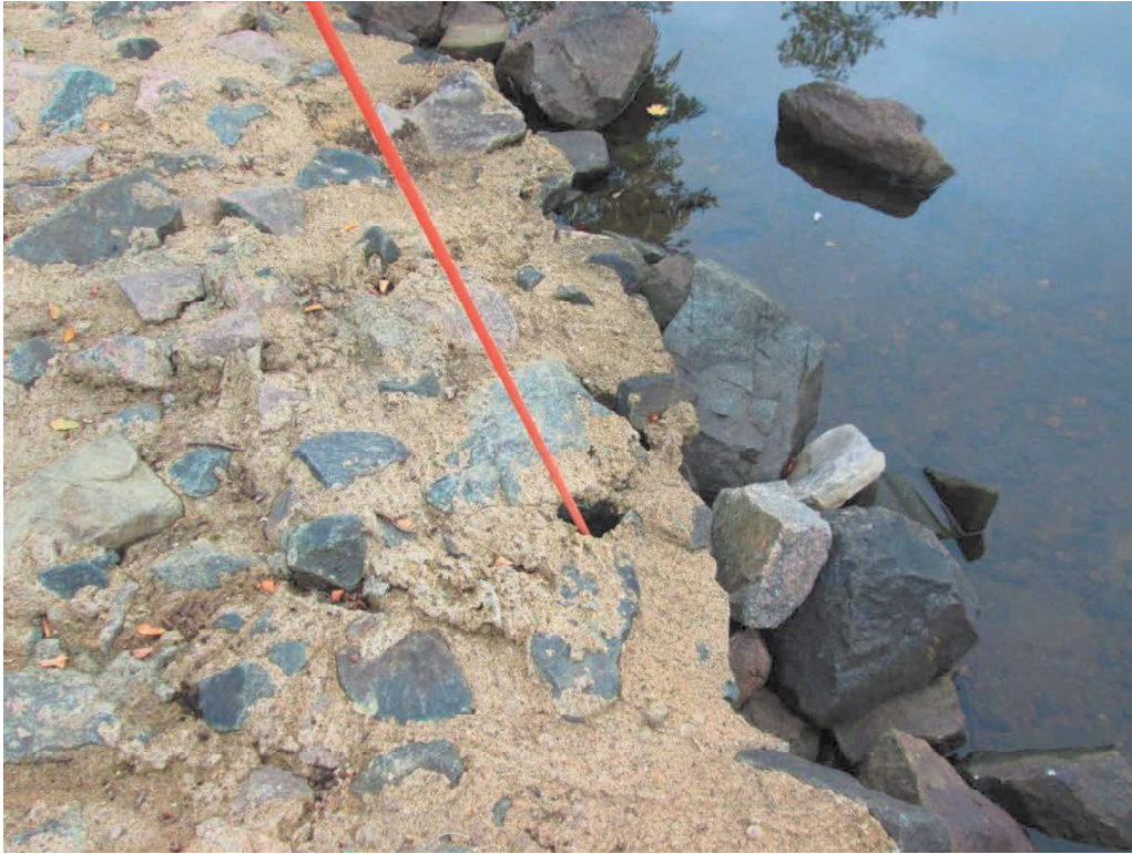
Photo No. 7: Closeup of voids and loss of grout within grouted riprap on the upstream slope of dam along the lake edge.
