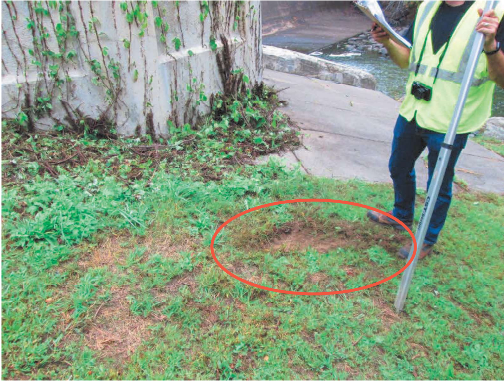
Photo No. 11: Closeup of rutting within exposed cellular concrete blocks on downstream slope to the right of the surge tank.
