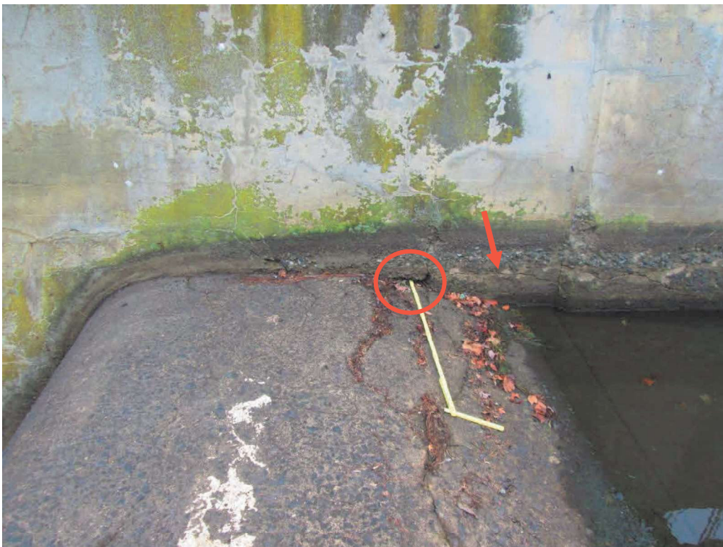
Photo No. 38: Closeup of the horizontal crack and void in the left sidewall of the gatehouse at the 90-foot long spillway weir.
