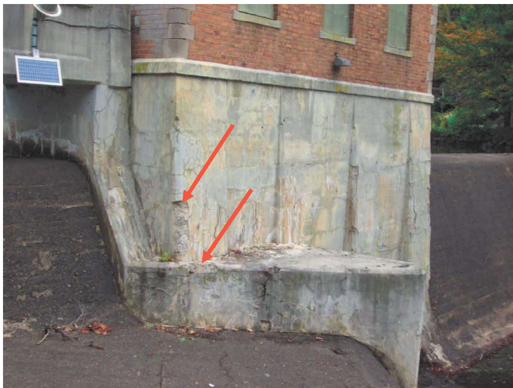
Photo No. 24: Downstream left wing wall and right gatehouse sidewall at the 30-foot long spillway weir looking left. Note the cracks and spalls in the gatehouse walls.
