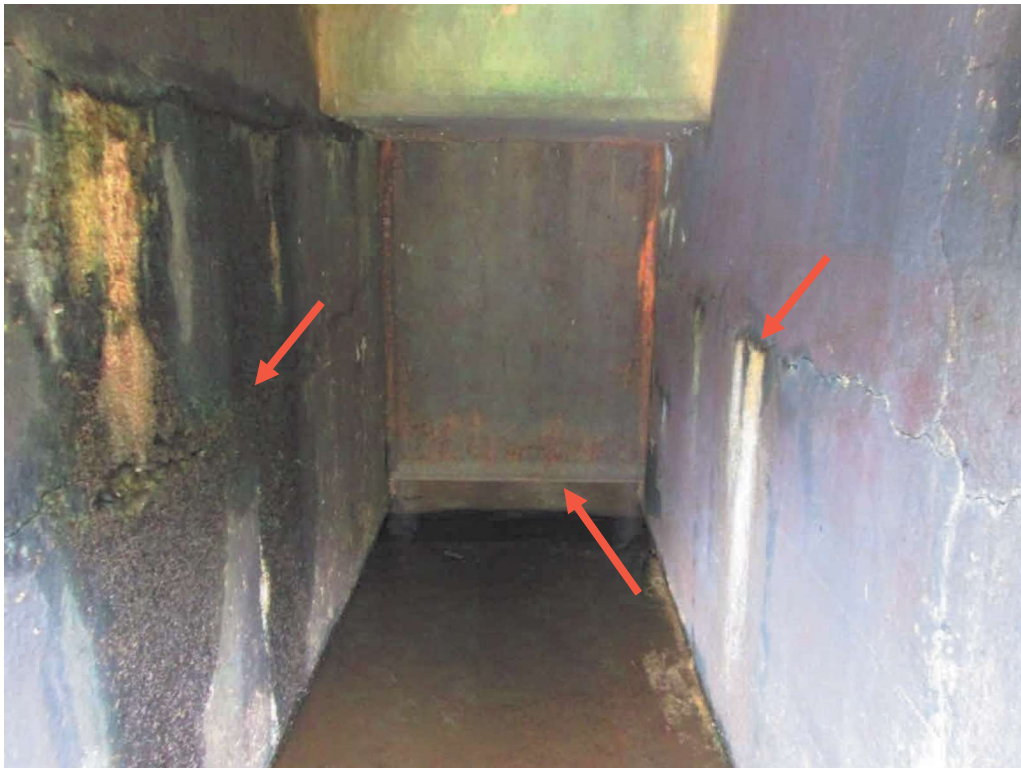
Photo No. 44: Downstream side of left low level outlet sluice gate and discharge chute. Note that the gate was partially open. Note the cracks with minor weeping in the discharge chute.
