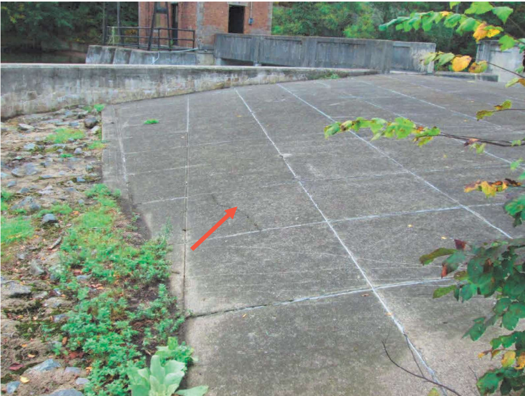
Photo No. 4: Concrete paving sections on the upstream slope of dam looking left. Note the crack in one of the concrete sections.
