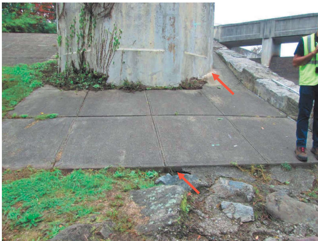
Photo No. 16: Closeup of concrete paving at the contact with the downstream and left sides of the surge tank. Note the efflorescence on the surge tank wall where wetness has been observed in the past. Also note the void in the grouted riprap at the contact with the paving.
