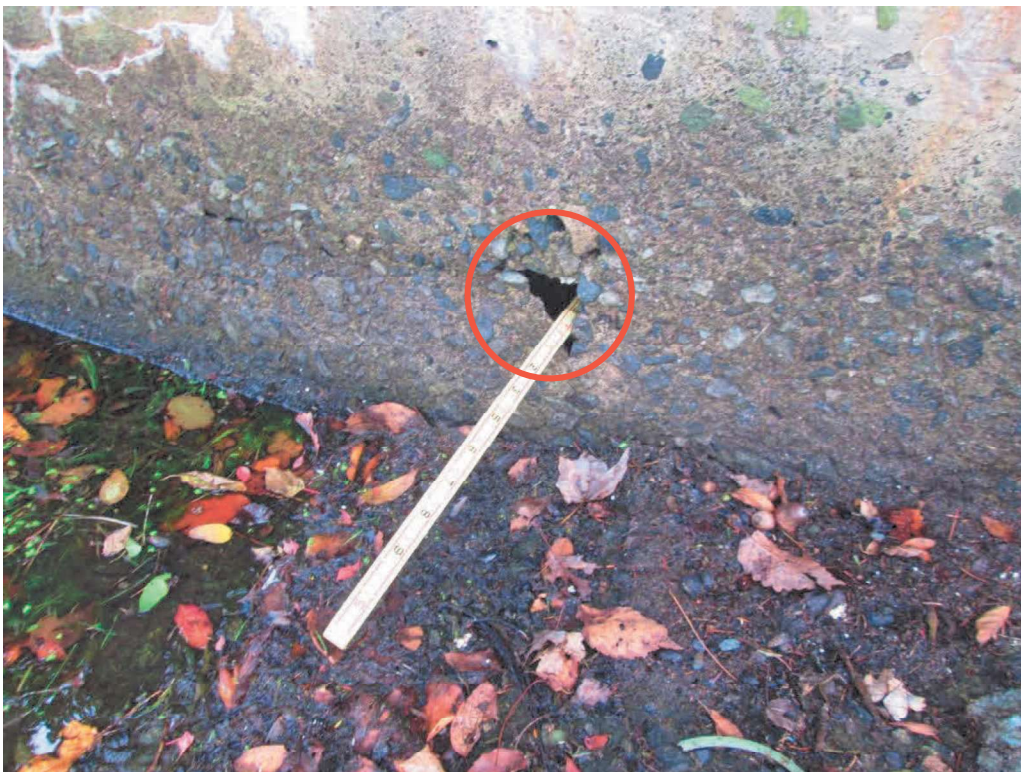
Photo No. 36: Closeup of the small void (24 inches deep) in the left training wall of the 90-foot long spillway weir.
