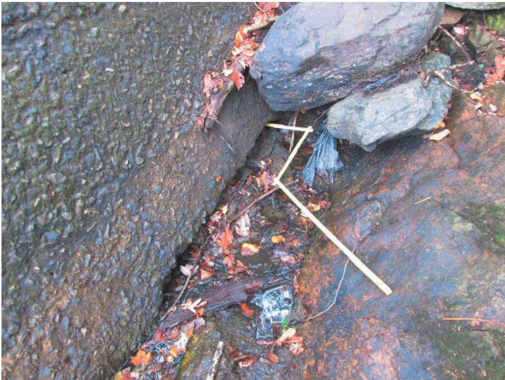
Photo No. 34: Closeup of the gap at the contact of the downstream face of the 90-foot long spillway weir with rock at the left abutment.
