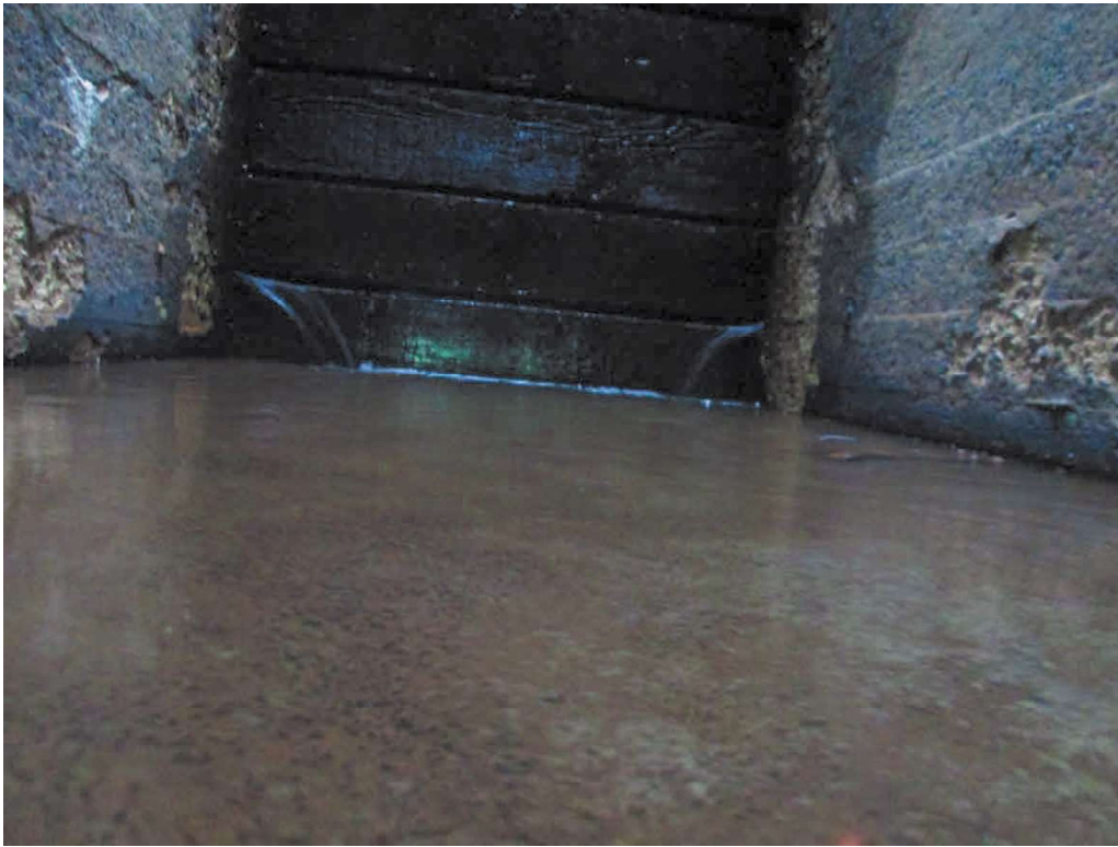
Photo No. 45: Closeup of stop logs upstream of left low level outlet sluice gate. Note the minor leakage through the stop logs.
