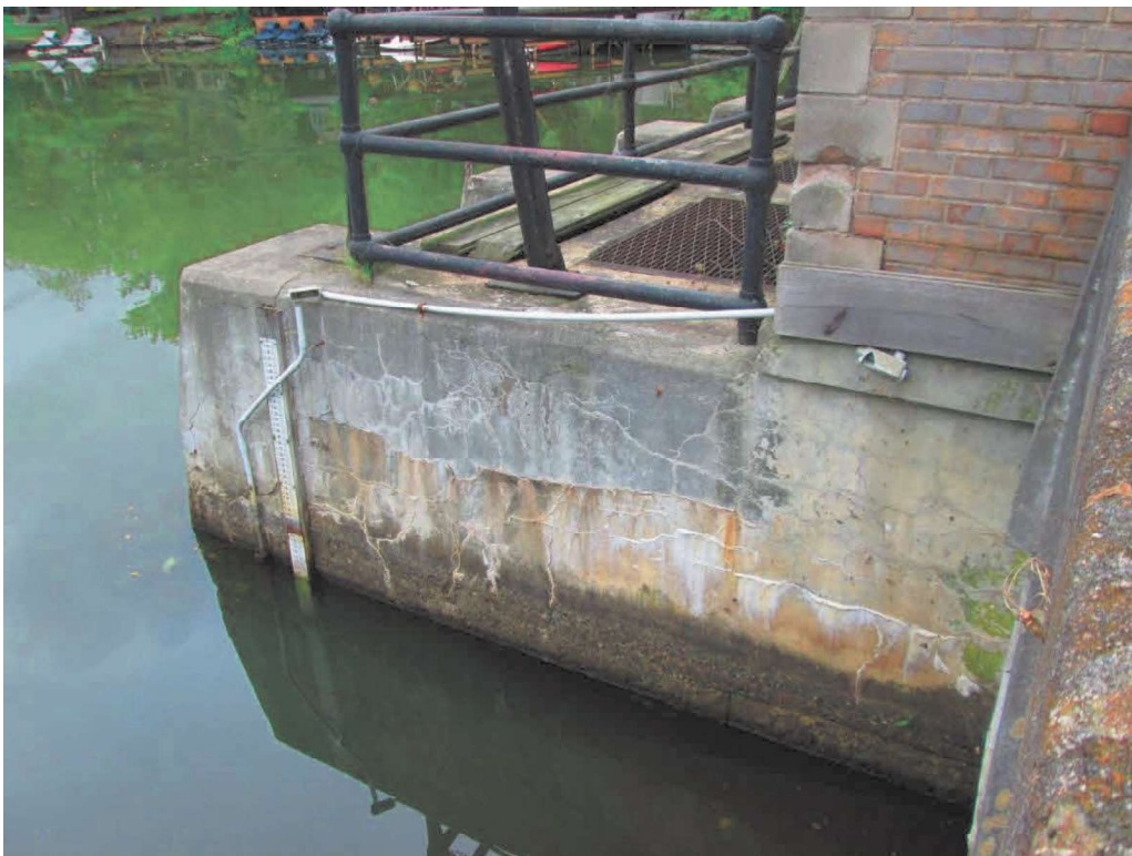
Photo No. 40: Closeup of the upstream portion of the left sidewall of the gatehouse at the 30-foot long spillway weir. Note the various minor cracks in the wall.
