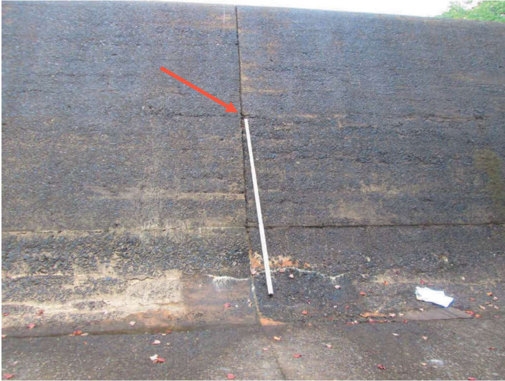
Photo No. 31: Right construction joint in the 90-foot long spillway weir. Note the minor spall at the construction joint.
