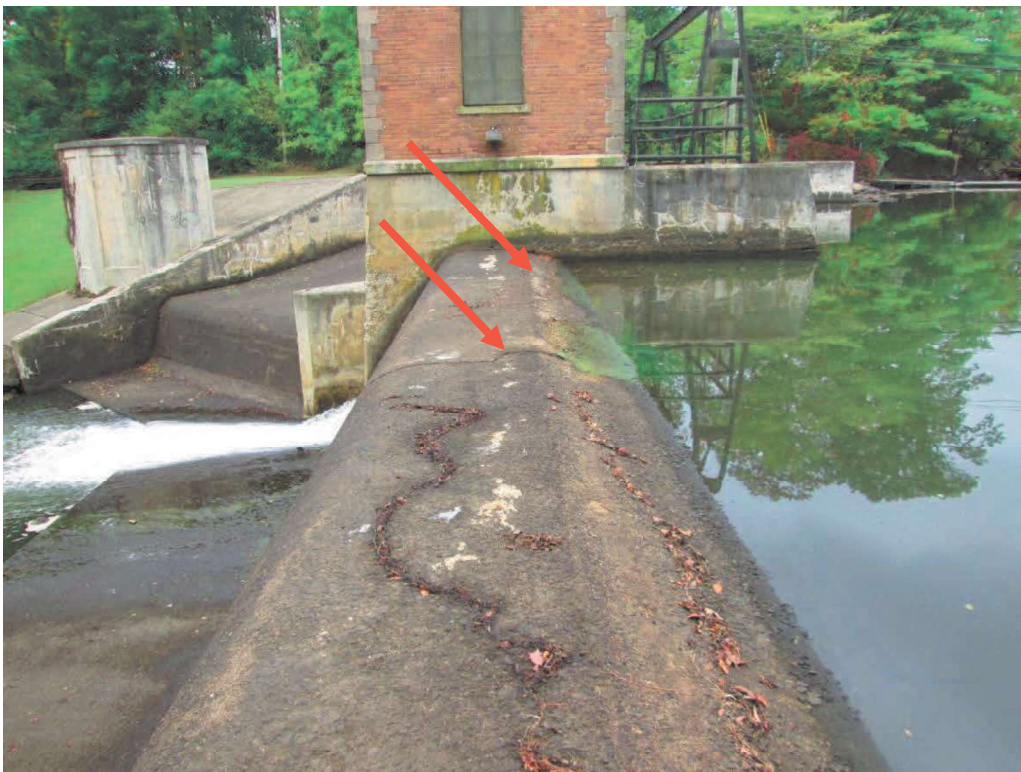
Photo No. 26: Crest of the 90-foot long spillway weir looking right. Note the right keyway joint. Also note the longitudinal crack along the upstream edge of the crest.
