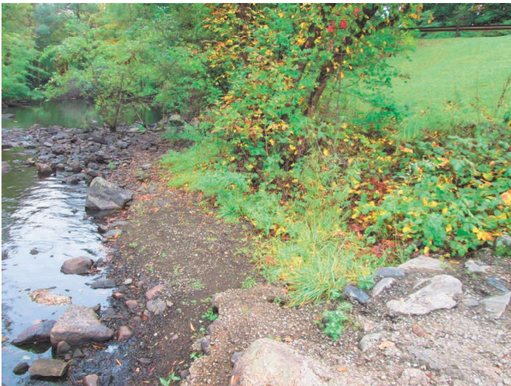
Photo No. 18: Lower downstream slope and toe of dam looking right. Note the trees and vegetation growing in the grouted riprap along the toe.
