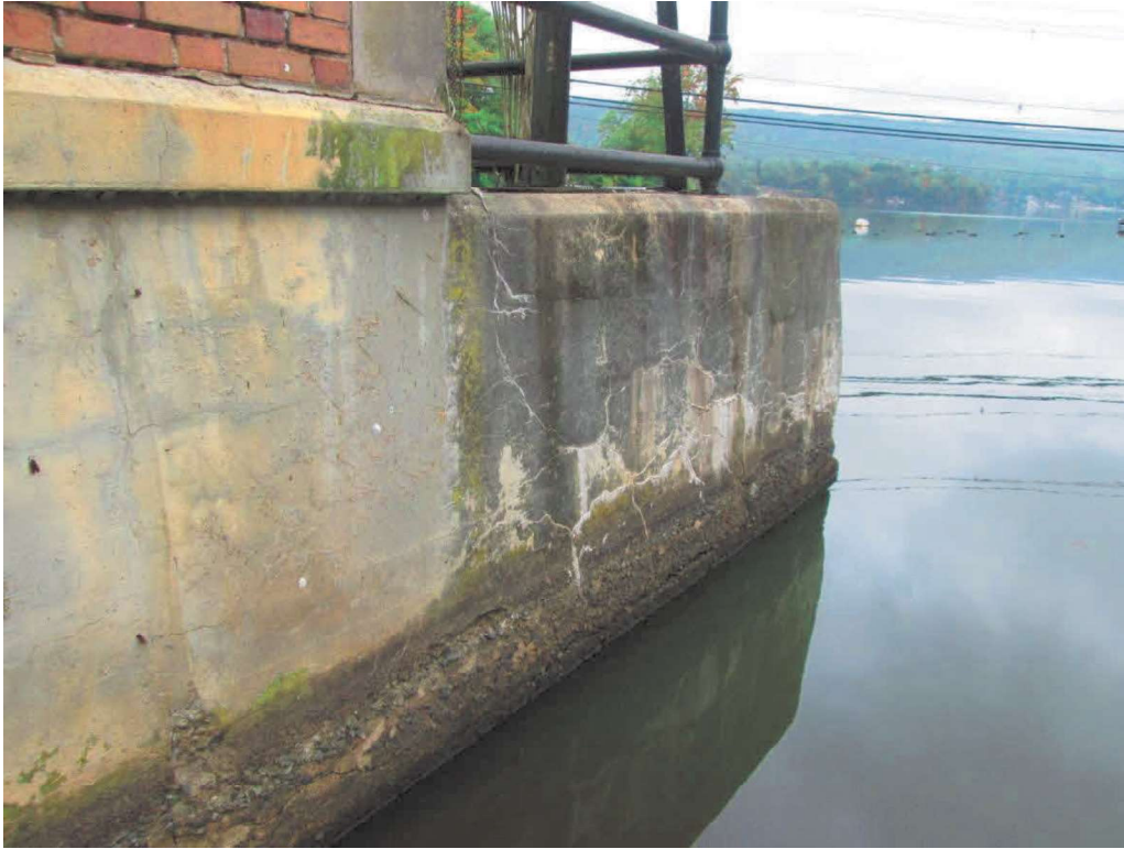
Photo No. 39: Closeup of the upstream portion of the left sidewall of the gatehouse at the 90-foot long spillway weir. Note the various fine cracks in the wall.
