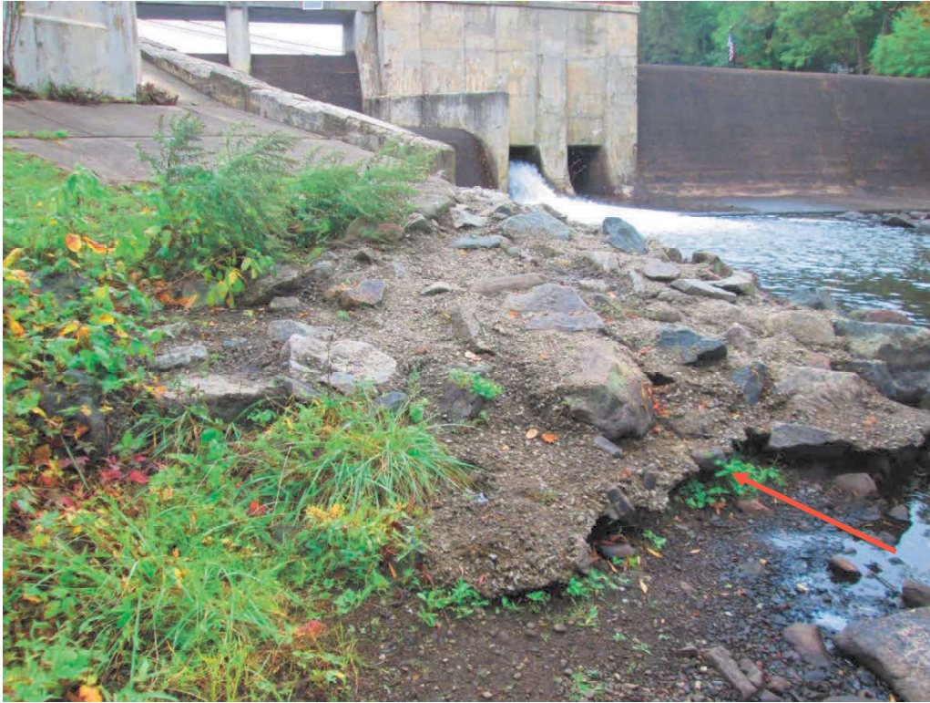
Photo No. 17: Grouted riprap along the lower downstream slope and toe of dam immediately downstream of the concrete paving looking left and upstream. Note the undermining at the downstream end of the grouted riprap.
