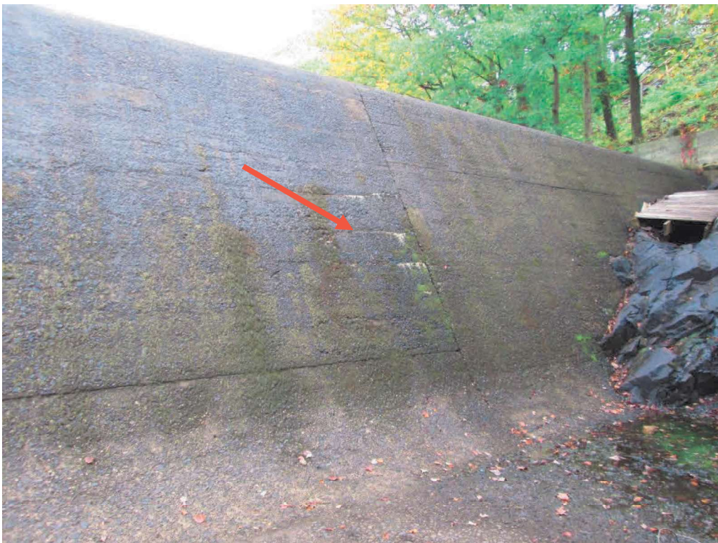
Photo No. 32: Left construction joint in the 90-foot long spillway weir. Note the efflorescence at horizontal cracks which are likely concrete lift joints.
