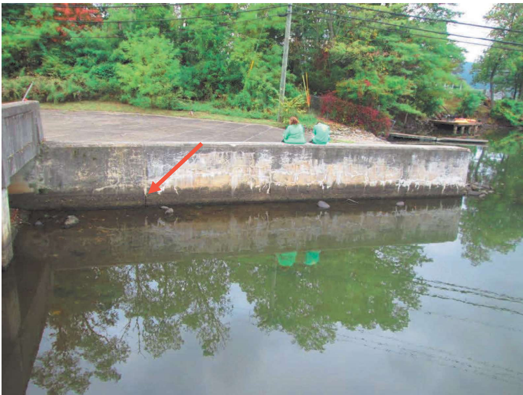
Photo No. 20: Upstream right training wall along the entrance to the 30-foot long spillway weir. Note the location of the gap at a construction joint.
