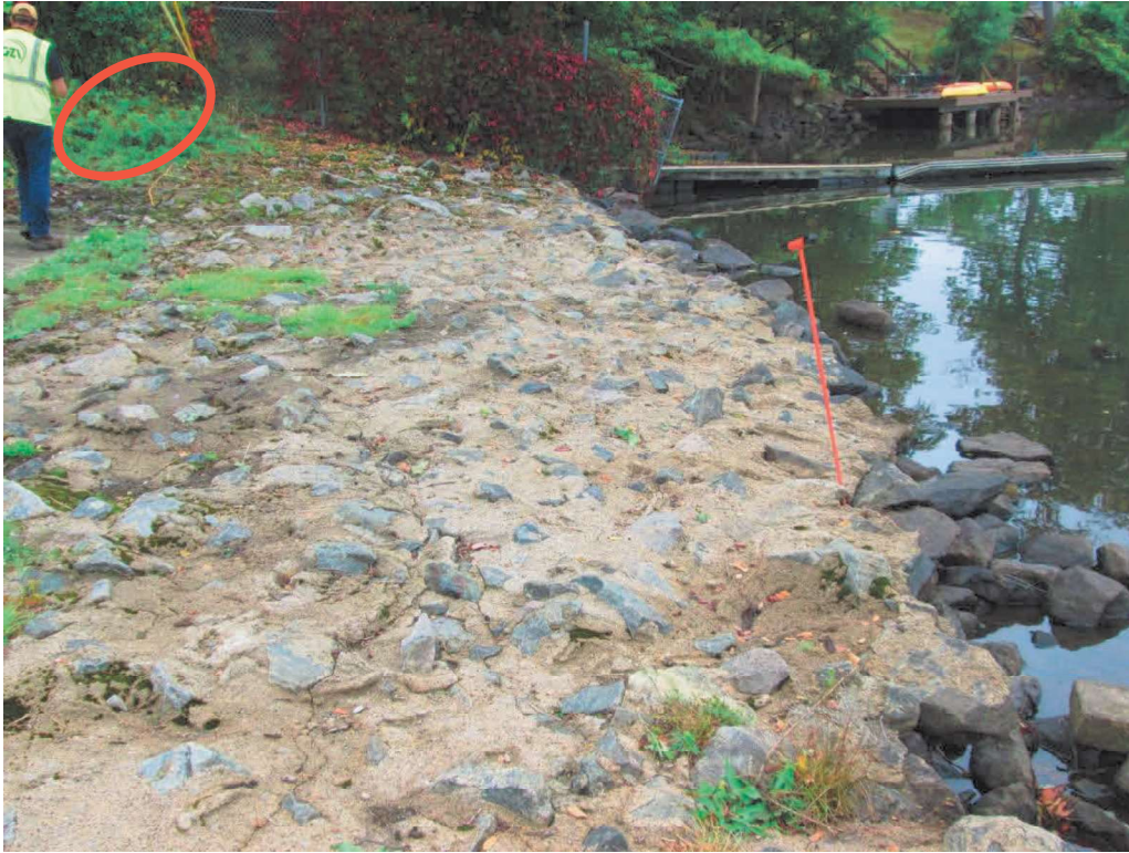
Photo No. 5: Grouted riprap on the upstream slope of dam looking right. Note the area of minor depressions and undermining of the grouted riprap at the contact with the grass near the right abutment.
