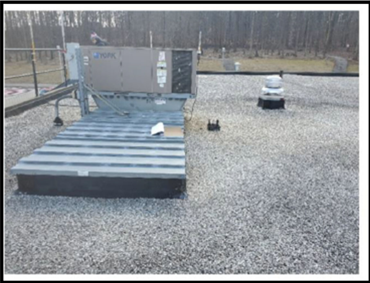
Rooftop Air Handling Unit (AHU)
