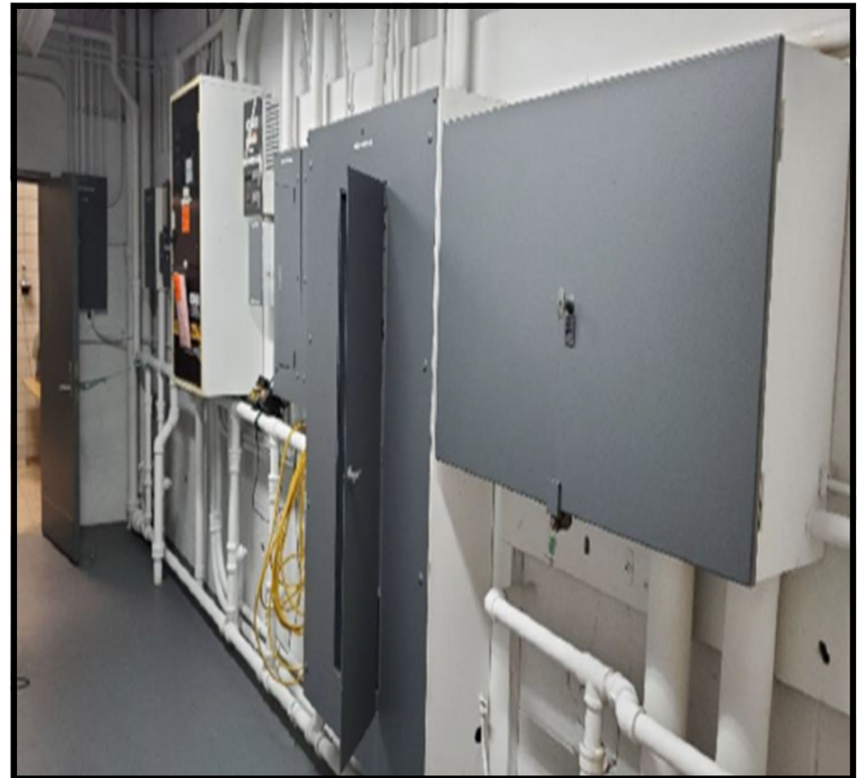
Transfer Switch & Electrical Panels
