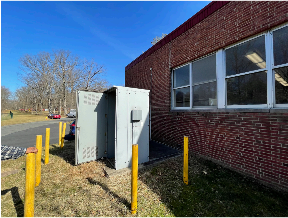
Existing Outdoor Switchboard
