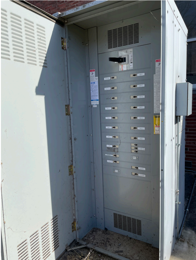
Existing Outdoor Switchboard
