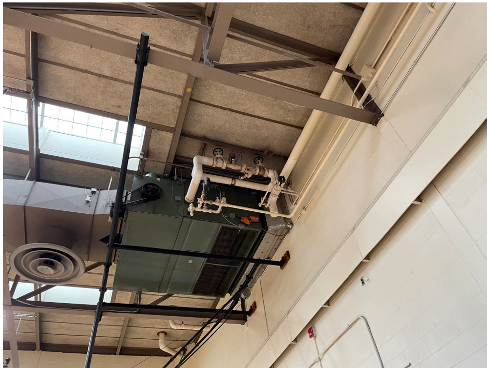
Existing Heating and Ventilation Unit
