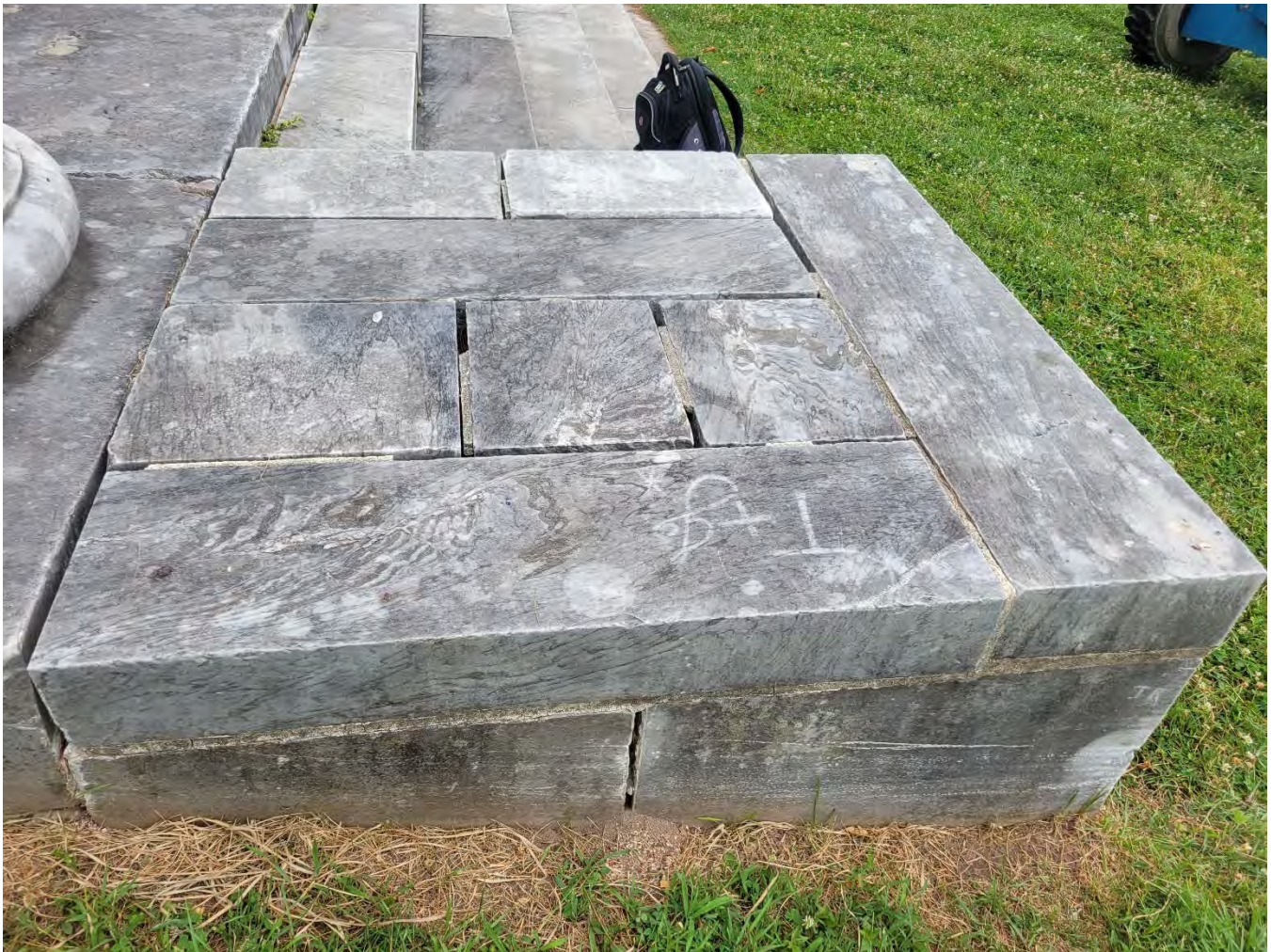
Photo 14: View of the west stair cheekwall showing open joints and masonry displacement. The bright white scratches and chip along the bottom edge are probably due to a lawnmower being run against the masonry.
