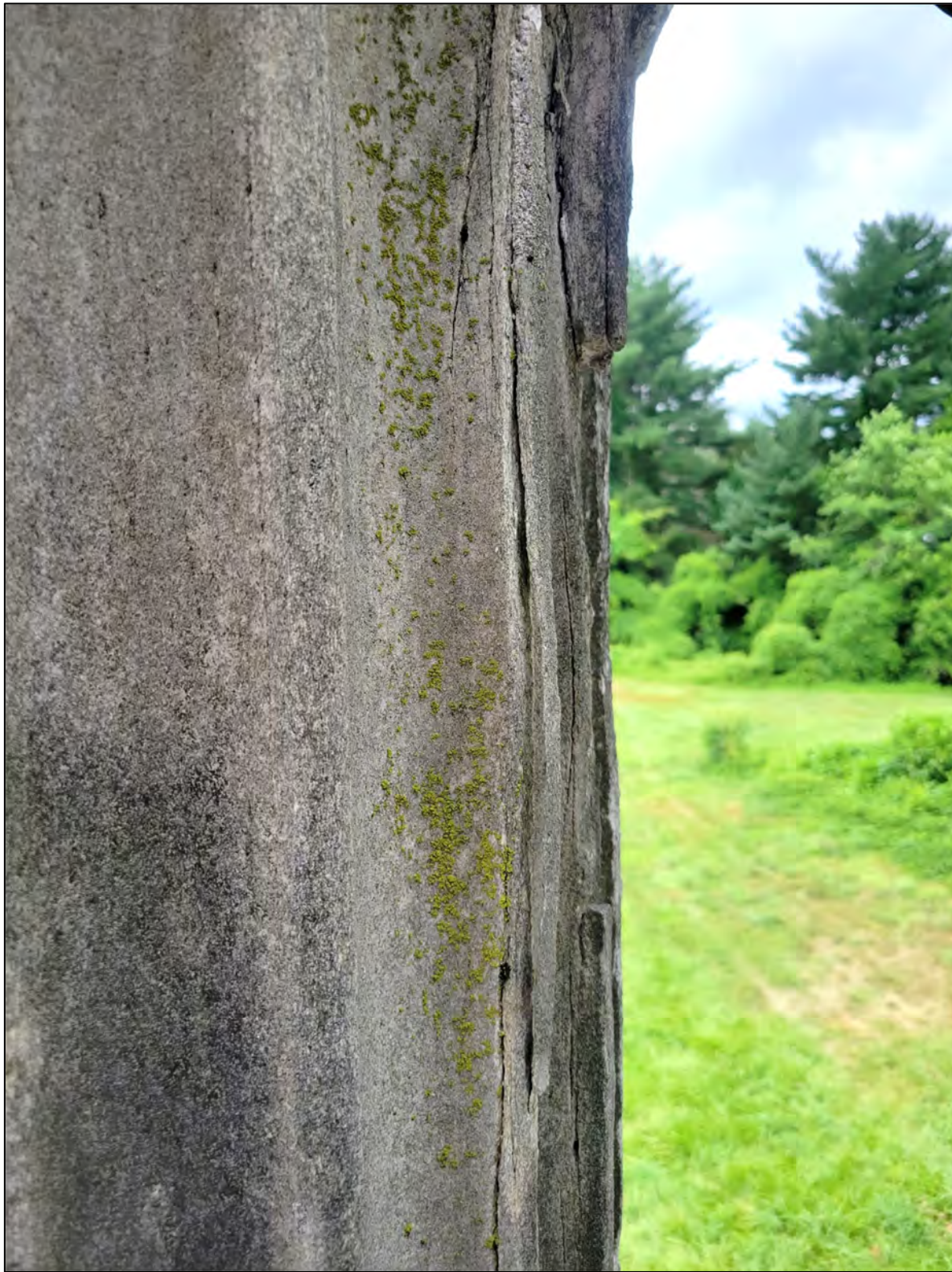
Photo 18: Detail of the deteriorated fluting at the west side of the south-center column.
