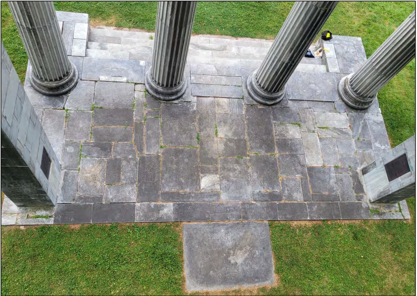
Photo 15: View of the southeast corner from above. Note the numerous open and deteriorated joints. Note also the top stone of the relief panel is pushed out to the east.
