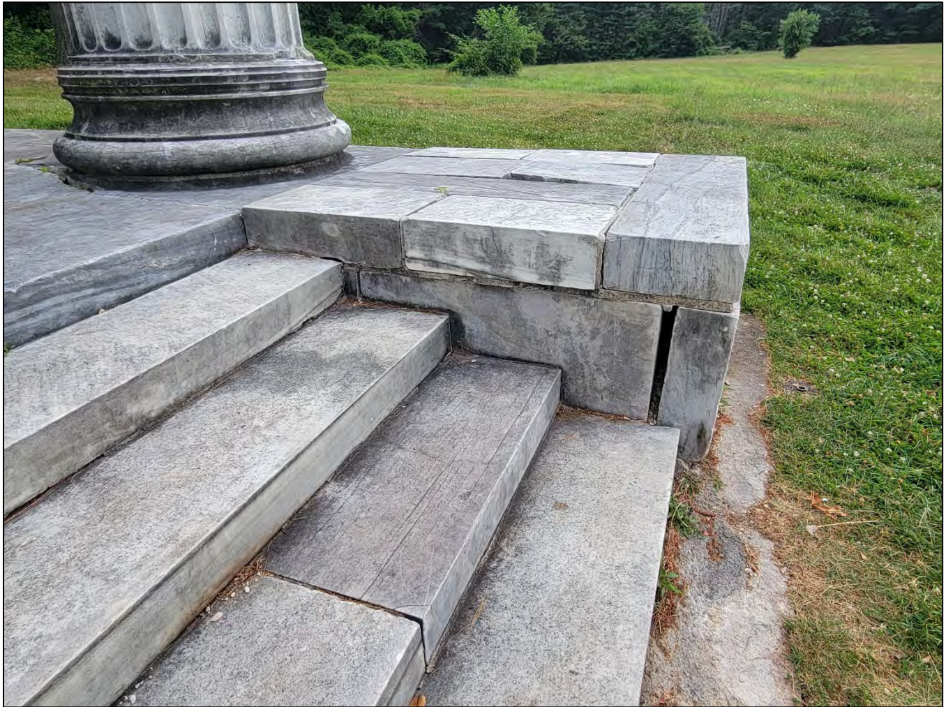
Photo 13: View of the east cheekwall from the west showing the extent of stone displacement and mortar conditions. The mortar joints in the stair are also open.
