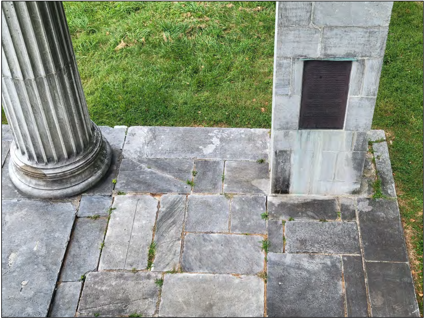
Photo 7: View of the paving at the west side of the construction. Note the cracked blocks, wide joints with vegetation, and the depression immediately behind the stone between the columns.
