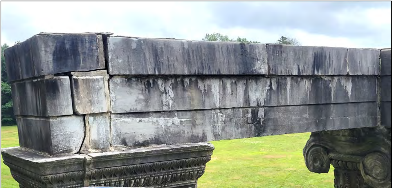
Photo 4: View of the west side of the east architrave block. The top section is comprised of three smaller pieces; note the white streaks below, indicating water is moving through the joints. Note the movement of the small blocks at the end above the square pier. There are horizontal fissures in the bottom section of the architrave stone.
