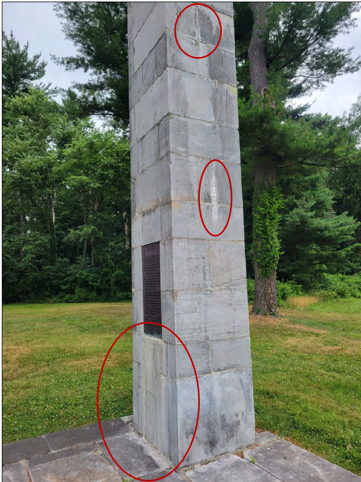
Photo 11: View of the south and west faces of the east pier showing calcium carbonate crusts below the plaque, exuding from a crack in a stone, and coming out of mortar joints.
