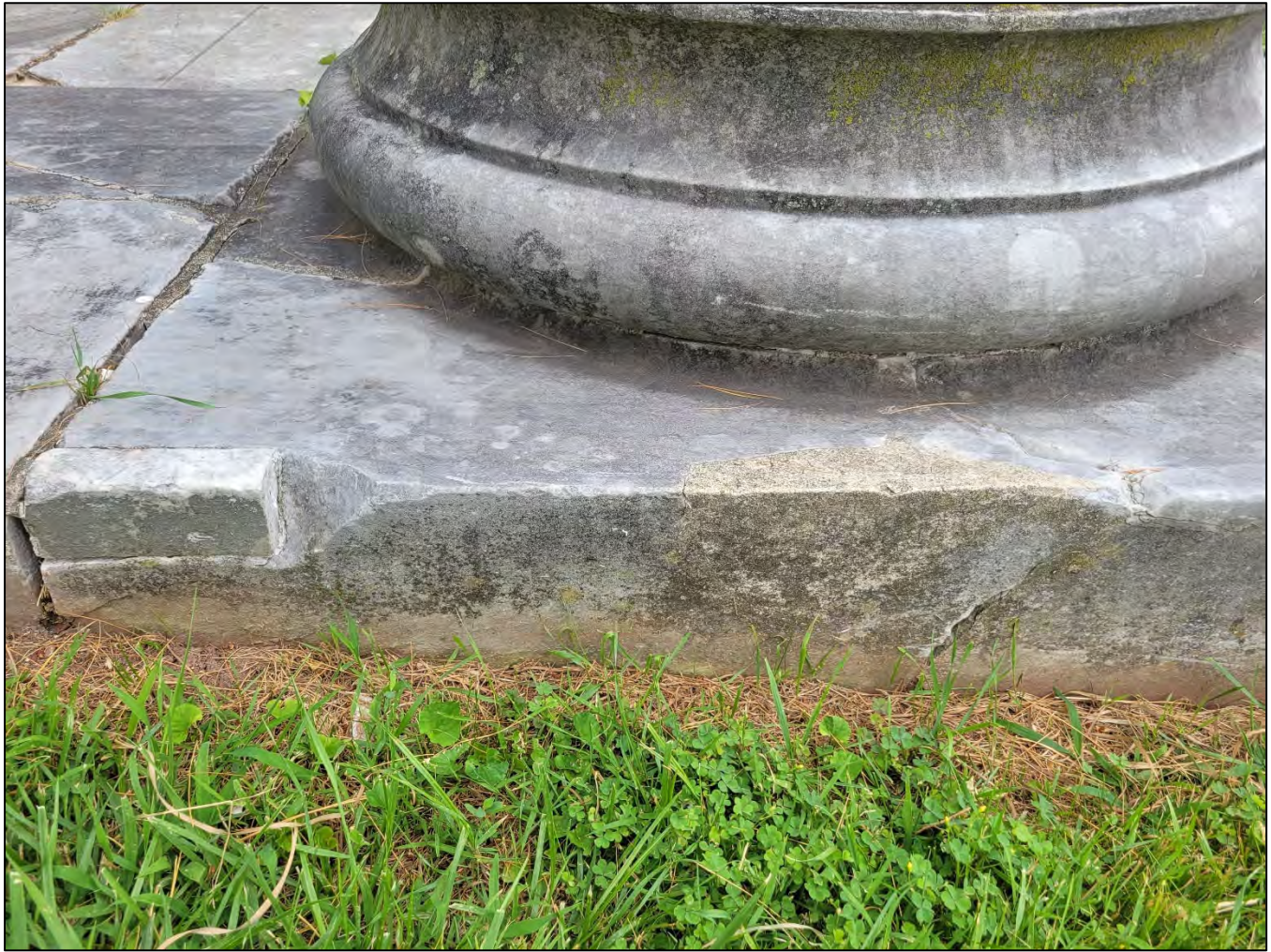
Photo 16: View of the west end of the colonnade showing the cracked column base and the adjacent cracked paver. There are two repairs to this stone: one dutchman and one patch.
