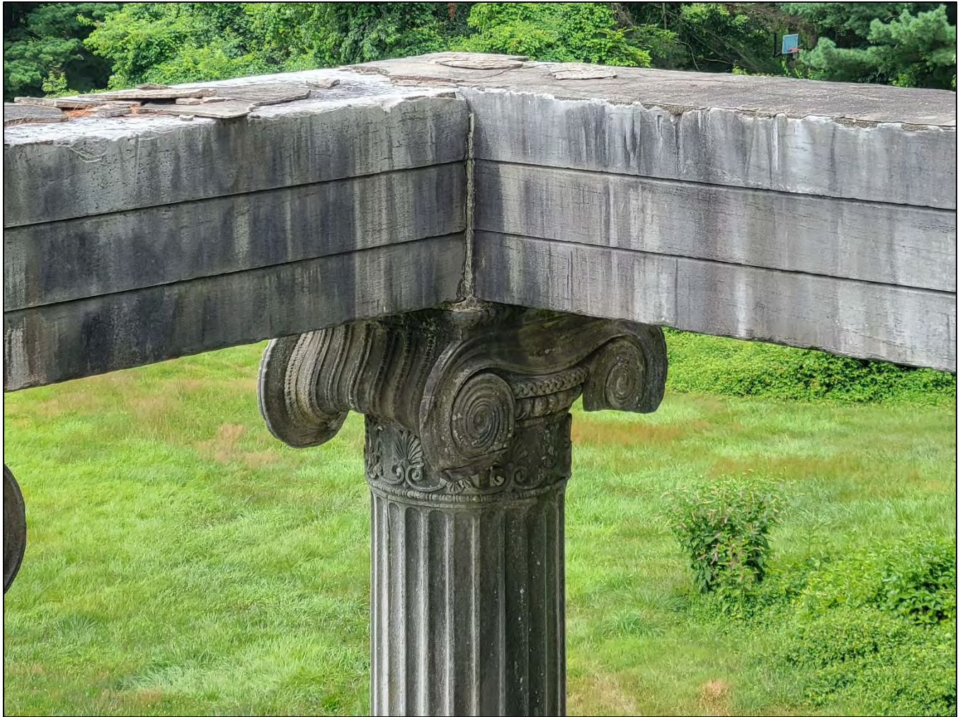
Photo 21: Loss and incipient spall at the north side of the southwest column capital.
