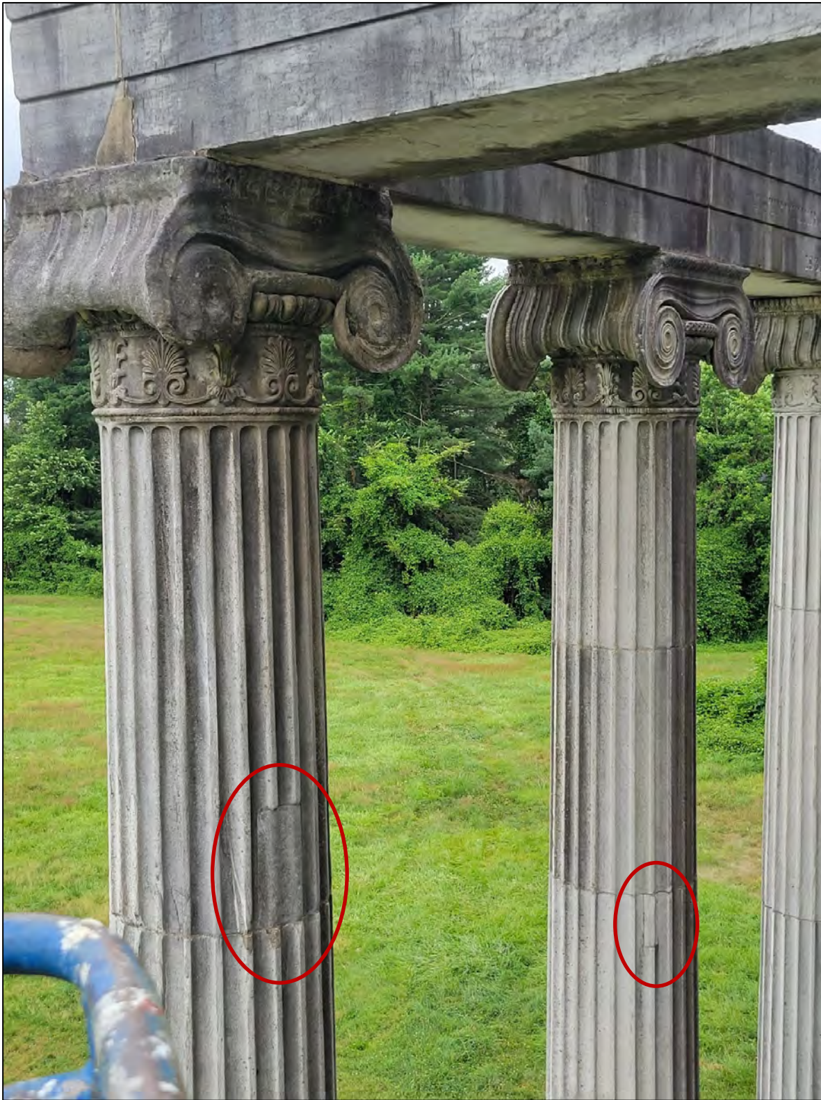
Photo 20: View of the north side of the same column capital as shown in Photo 18 showing loss and old repair of the north side volutes—compare the appearance with those of the adjacent column. Note also the old dutchman repairs at the columns; the dutchman at the southeast column has spall patches to the volutes below.
