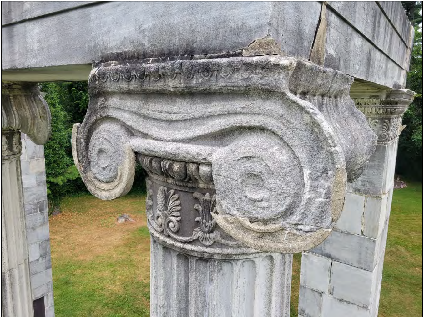
Photo 19: View of the south side of the southeast column capital showing old cementitious patch repairs; these are soundly attached.
