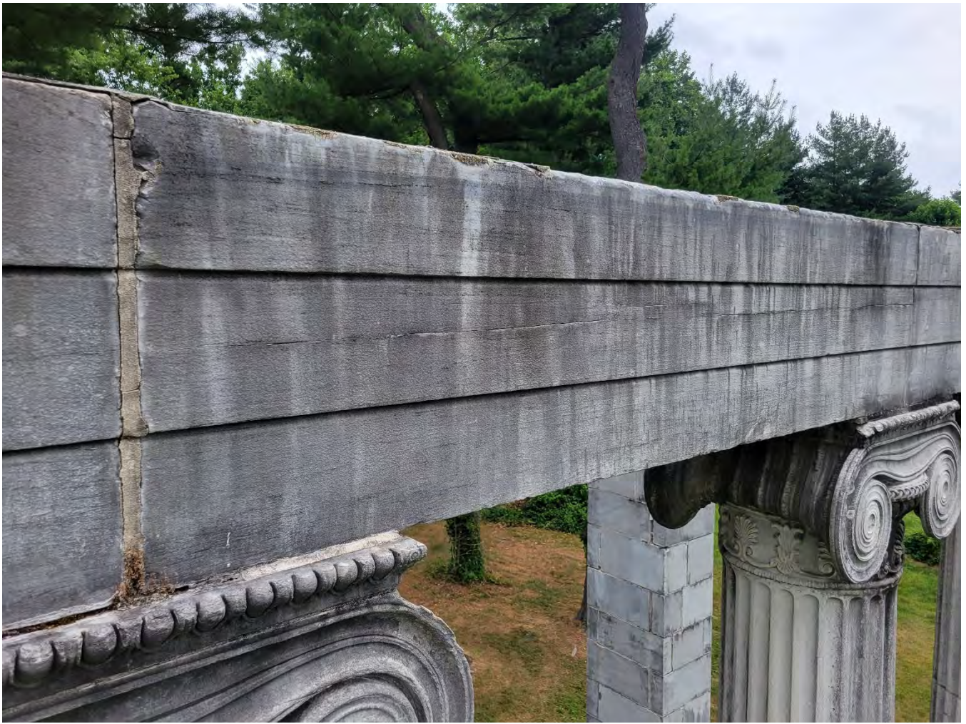
Photo 22: Fissures in the central stone at the south elevation. The condition of the mortar joints in the architrave and between the architrave and column capital is typical.
