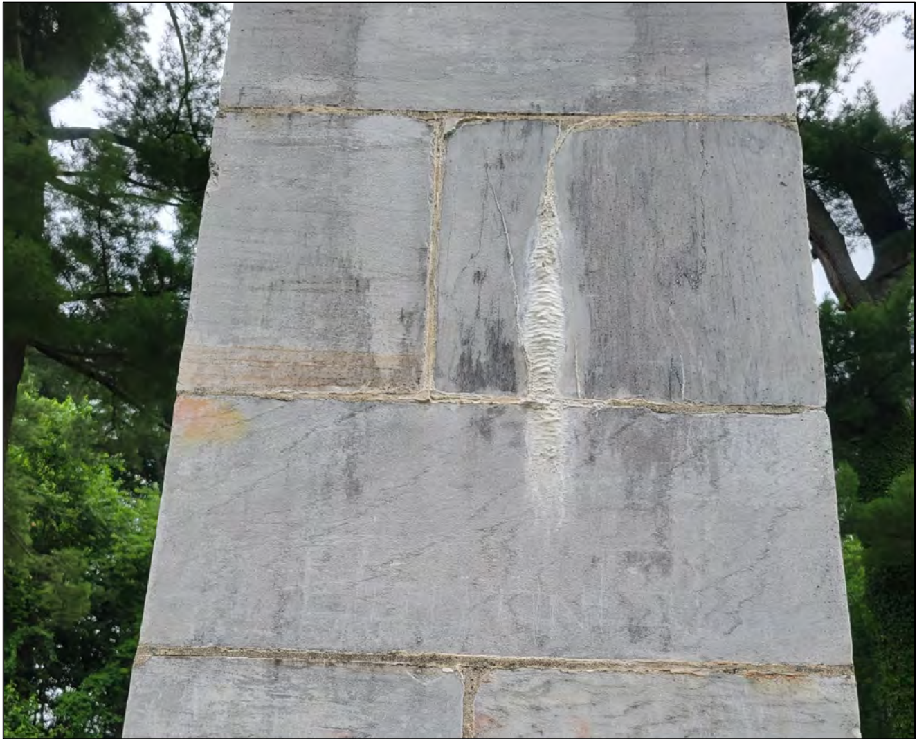
Photo 12: Detail of the cracked stone shown in Photo 10. The orange discoloration is biological.
