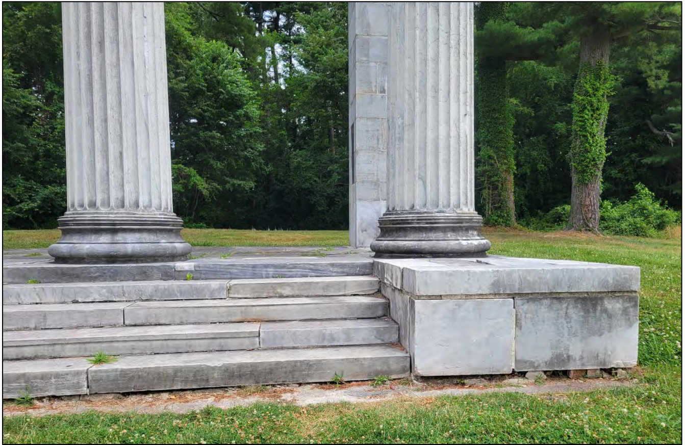
Photo 6: View of the east end of the stairs and the east cheekwall. There is concrete along the base of the stair, but also exposed brick at the bottom of the cheekwall.
