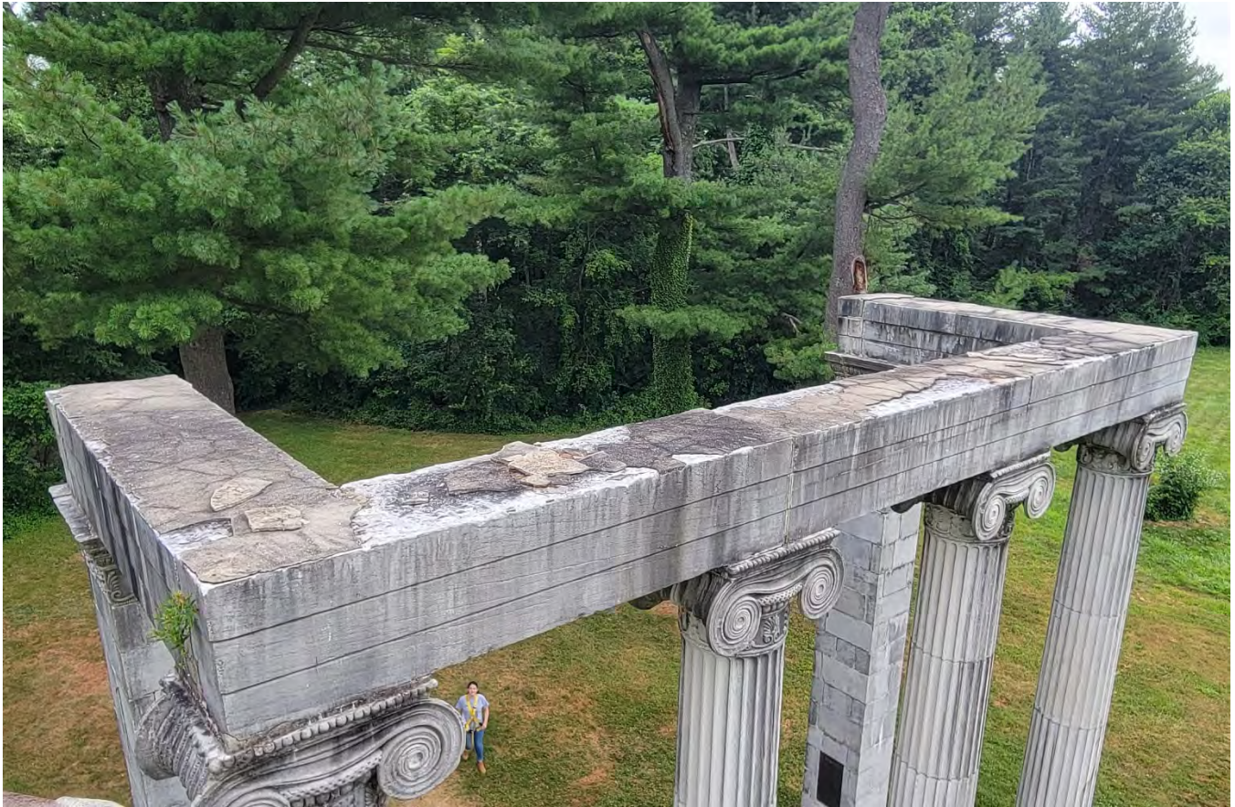
Photo 10: View of the top of the colonnade showing the deteriorated cementitious parging covering the surface. The parging is detached from the surface of the stone and there are many loose, displaced fragments.
