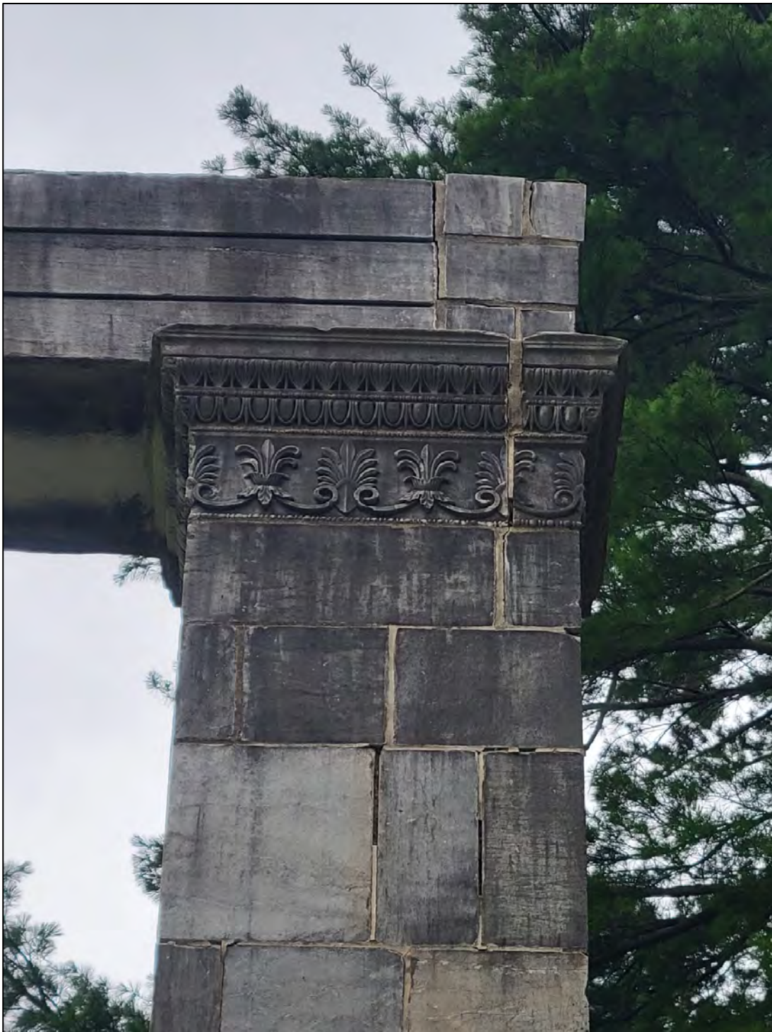
Photo 9: View of the east side of the west pier. Compare with Photos 4 and 8. The conditions at the top of the pier are less severe, but similar deterioration and movement is apparent. The detached parging at the top of the architrave is also just visible. There are also open joints.
