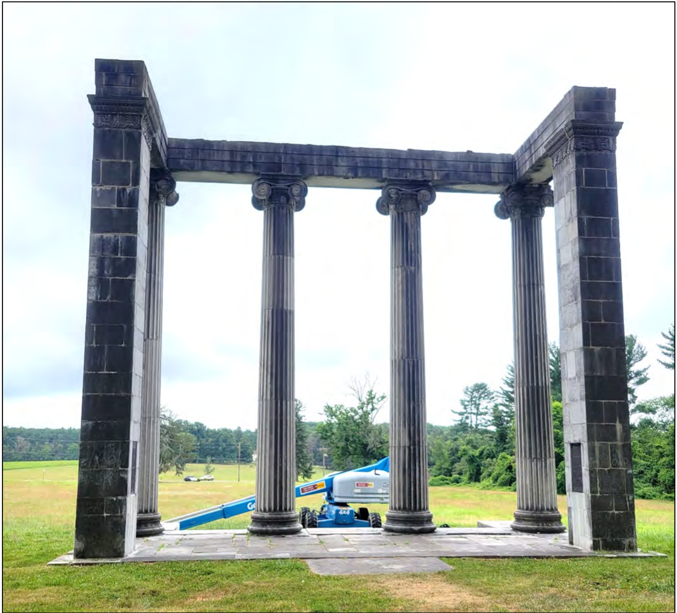
Photo 5: View of the north elevation showing that the construction is open to the rear. The white streaking visible on the piers is indicative of water moving through the masonry.
