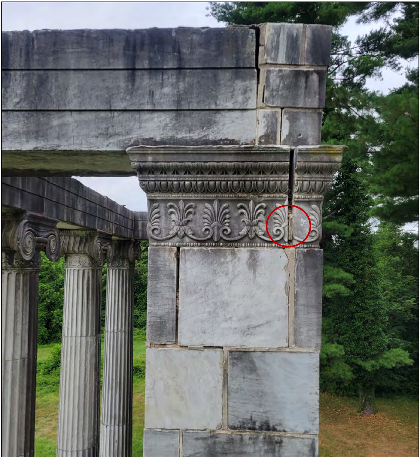
Photo 8: View of the east side of the east pier showing the displaced masonry and deteriorated mortar joints. The condition of the masonry above the west pier is not as severe; see Photo 9. The circled joint was loose and was removed.
