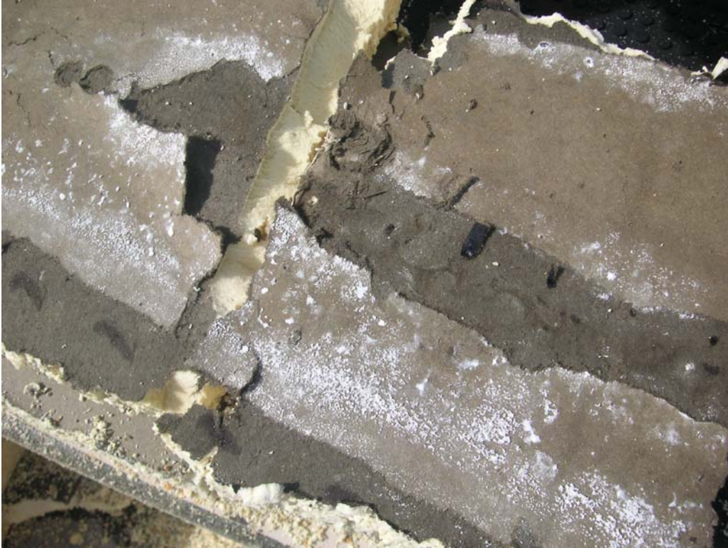
82. Bottom of insulation wetted with bloated facing sheet and mold throughout
