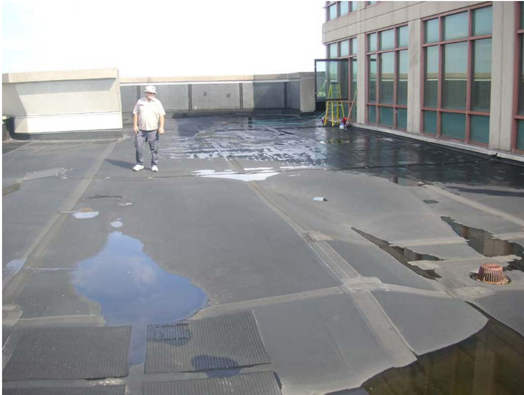
54. Large deformation in membrane
