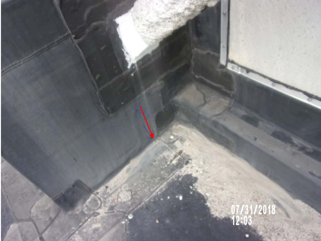
1. Roof Area D : Slice in the EPDM membrane at the base of the wall.
