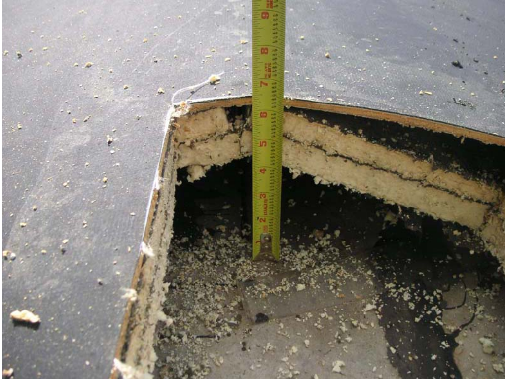
90. 4" heave in insulation
