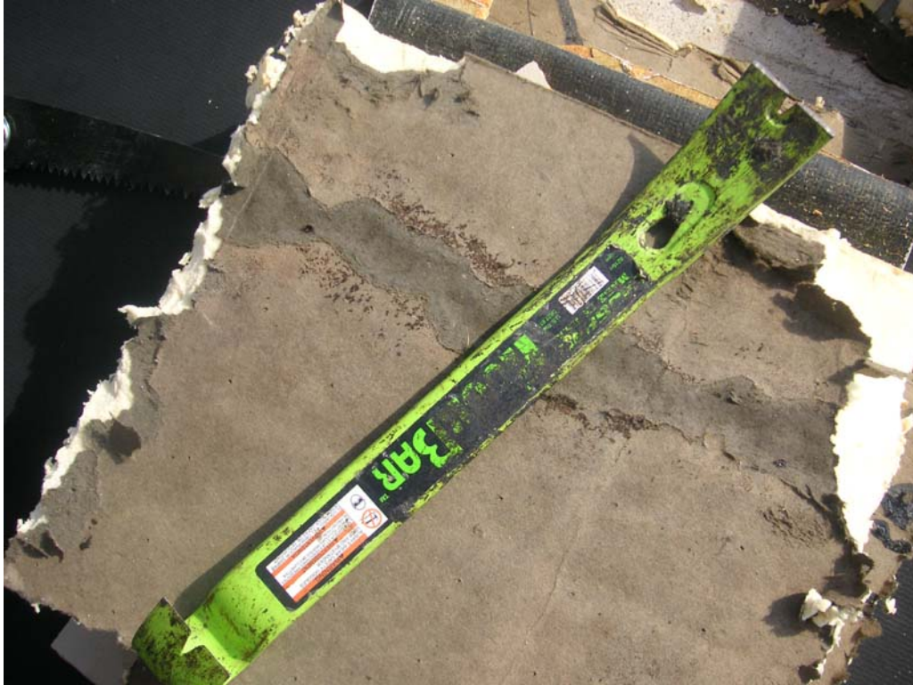
38. Underside of top insulation board has moisture damage
