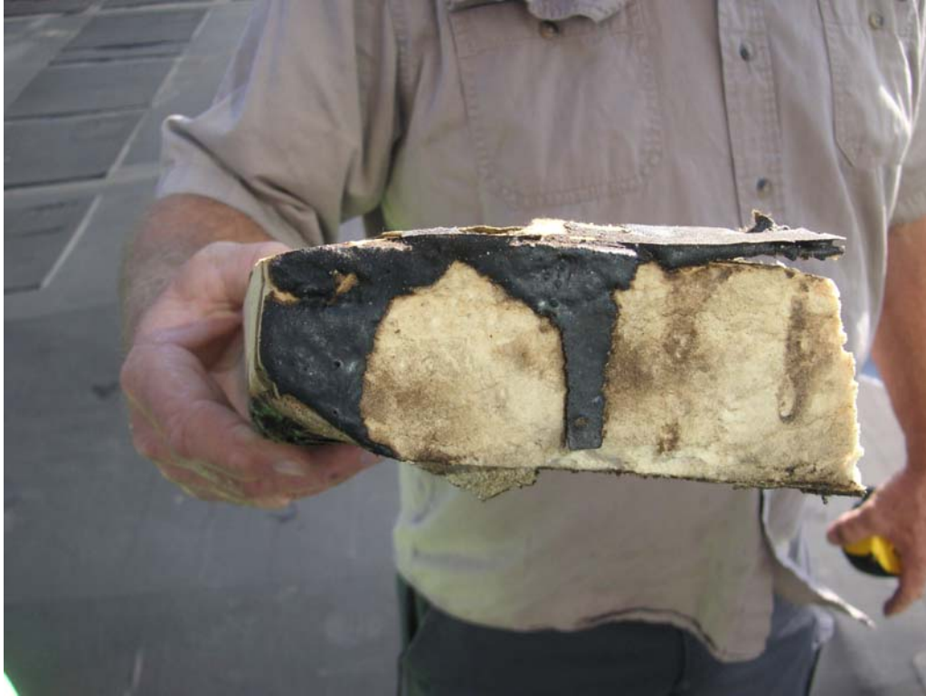
15. Board was deformed by thermal movement
