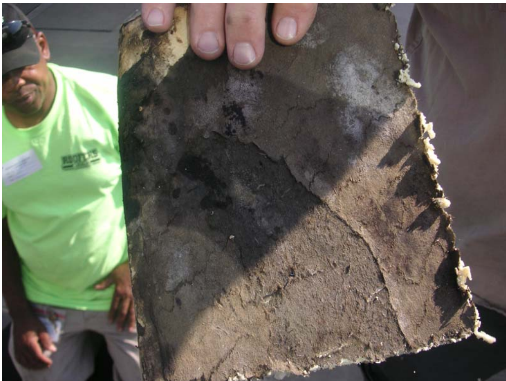
16. Good attachment between insulation that sheared
