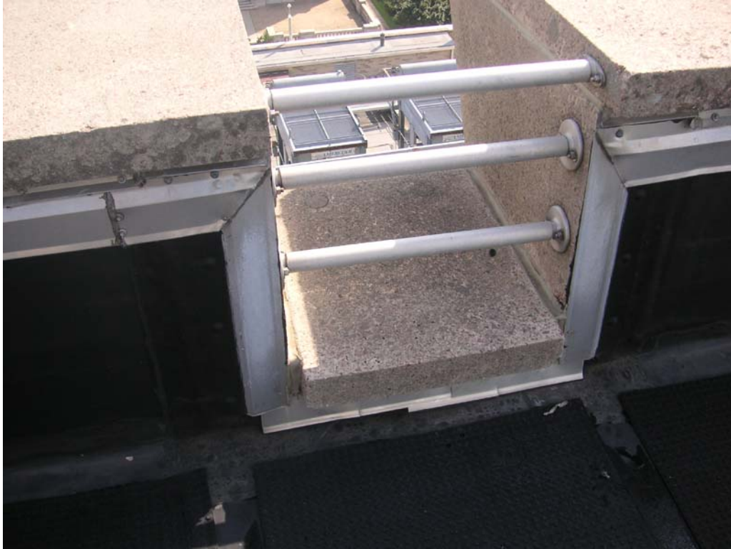
42. Cut-out is called a “crenel”, which is the bottom section of a merlon and crenel
