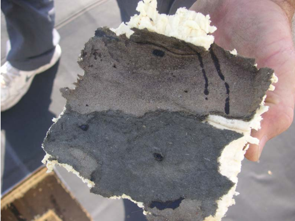
25. Bloating of facing sheet due to moisture
