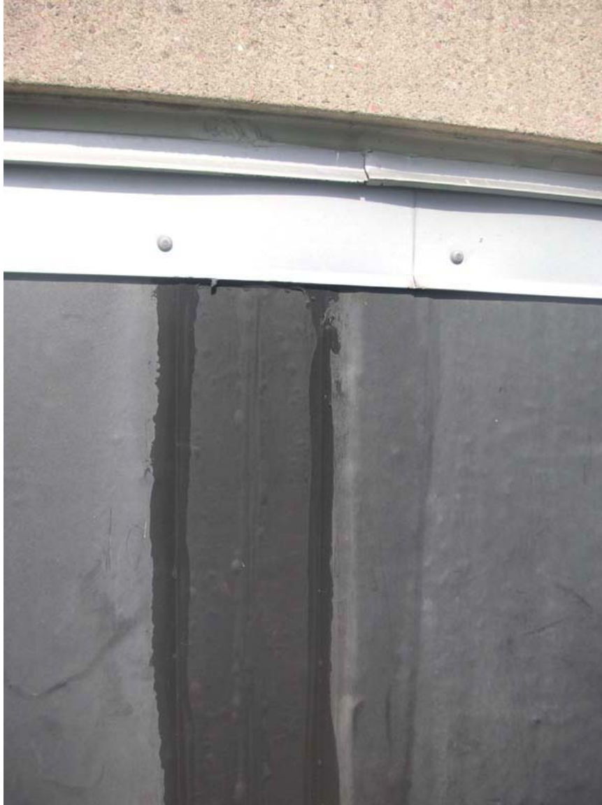
58. Extensive leakage at wall and metal connections
