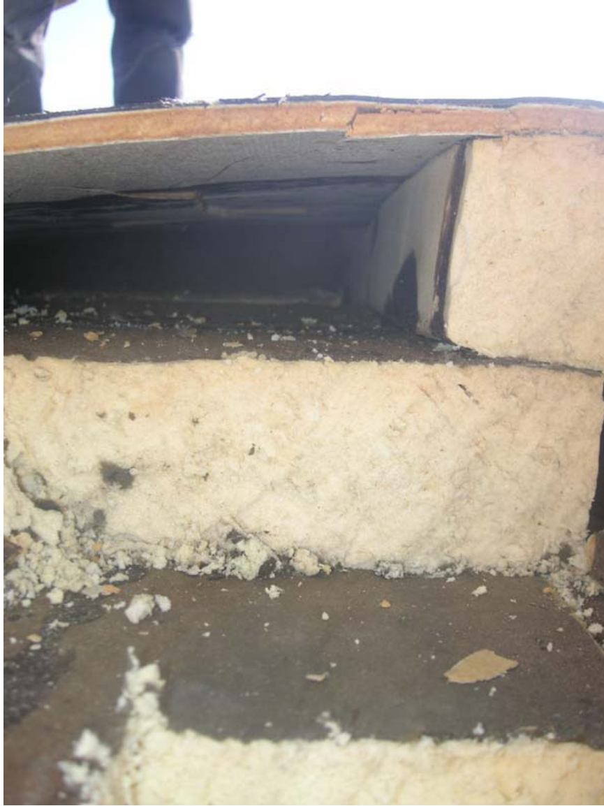
12. Open gap under board
