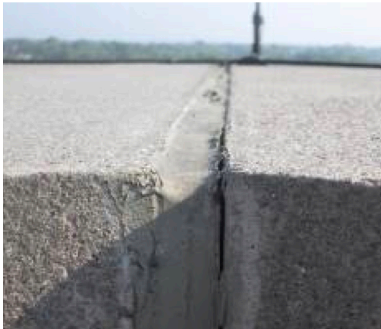
8. Coping Split in caulk at shoulder of cast stone.
