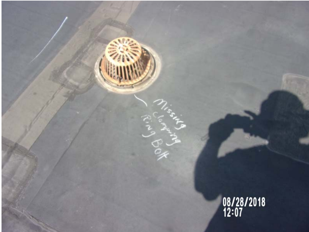
2. Roof Area C : Missing drain clamping ring bolt.
