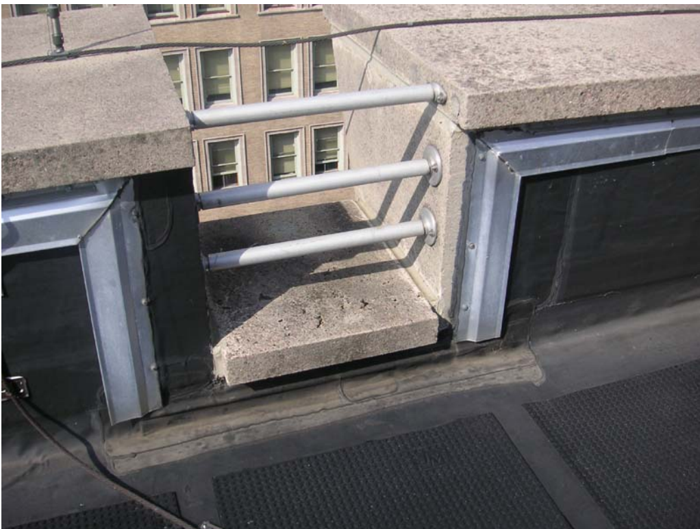
57. Crenel sections that leaked
