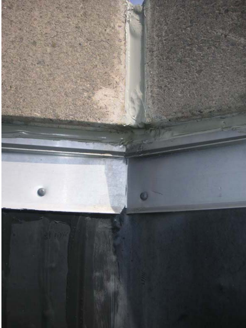
50. Constant overflow of water over counterflashing
