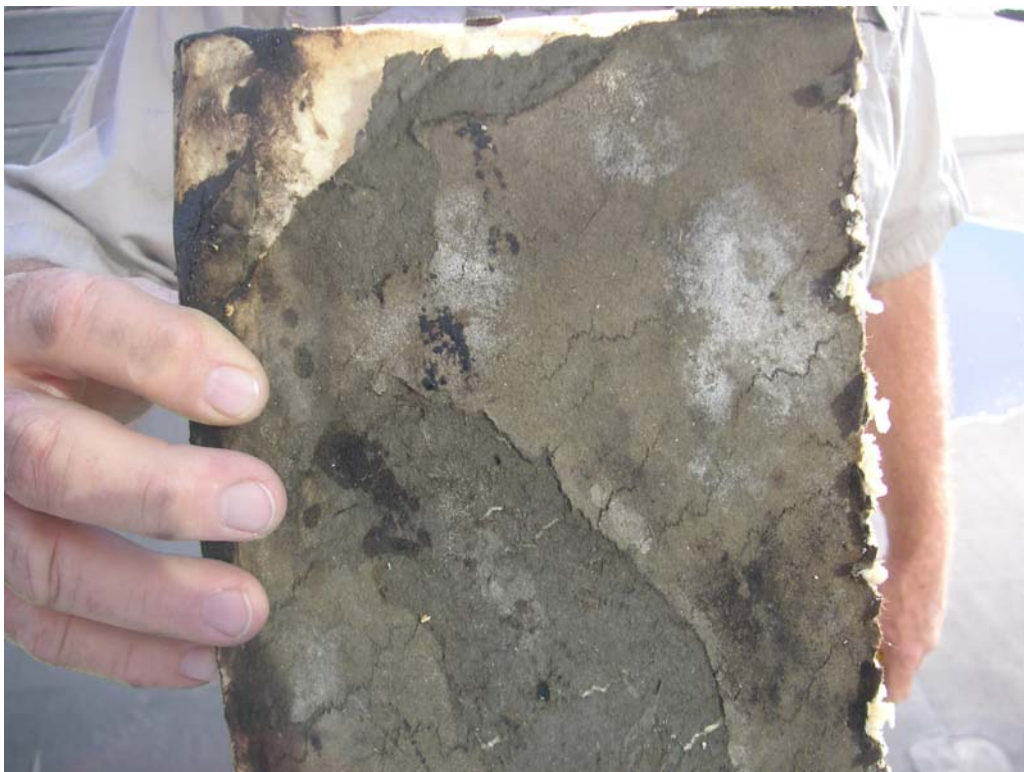
14. Mold growth on underside of top layer of insulation
