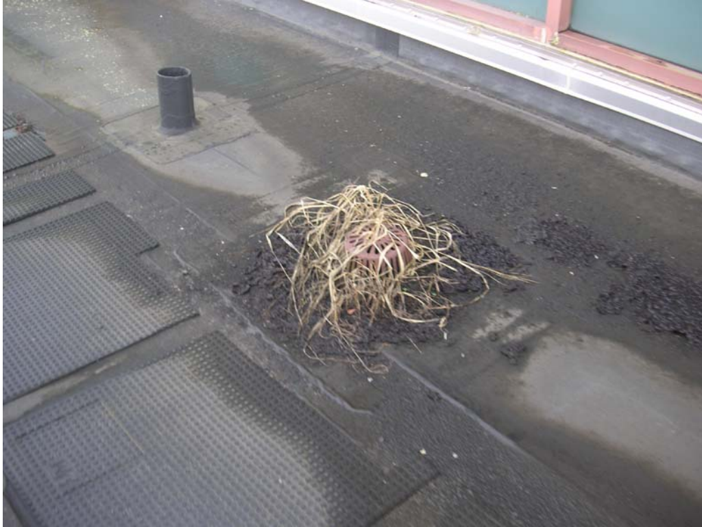
62. Lack of maintenance
