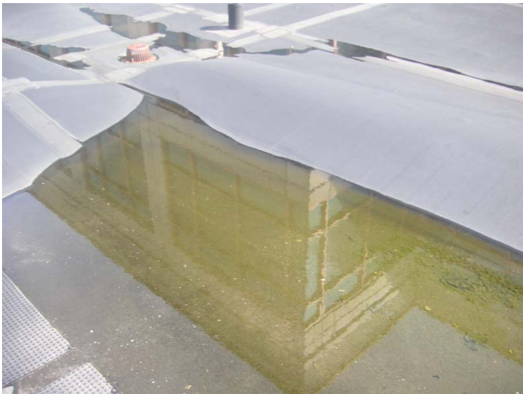
55. Ponding due to deformation
