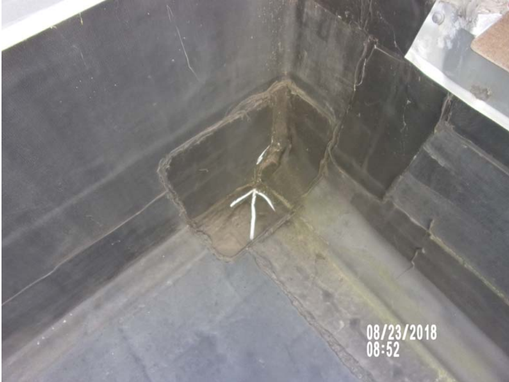
1. Roof Area Q : Typical delaminating inside corner patch.
