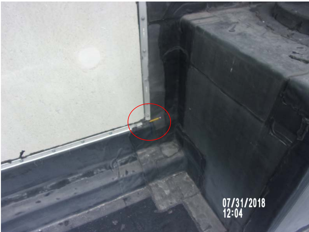
2. Roof Area D : Pencil indicating an opening.
