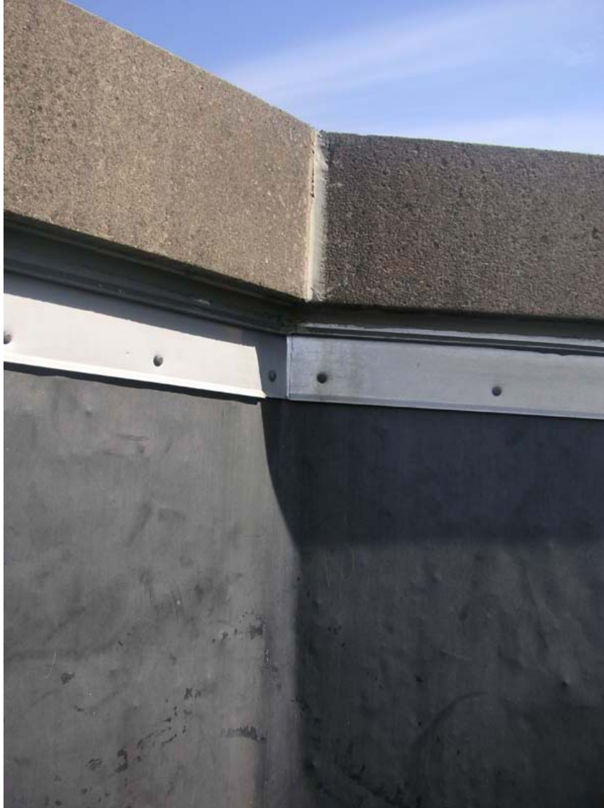
59. Constant leaking of water from stone work
