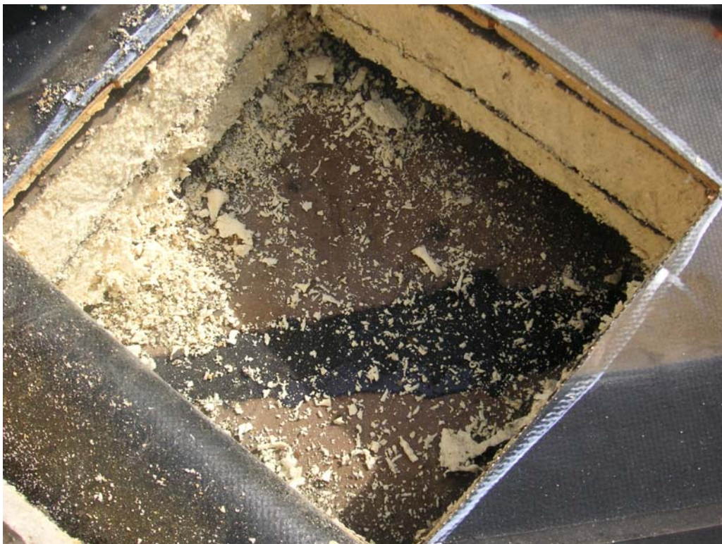
71. Saturated concrete deck
