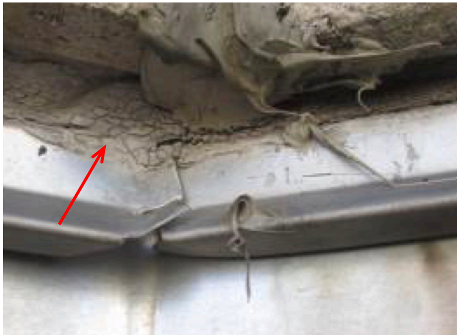
10. Caulking at Windows. Original caulk 31 years ago never removed to allow water intrusion to base of system
