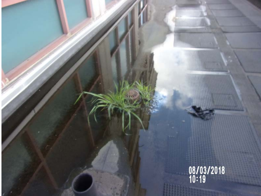
1. Roof Area B: Vegetation growth obstructing drainage.
