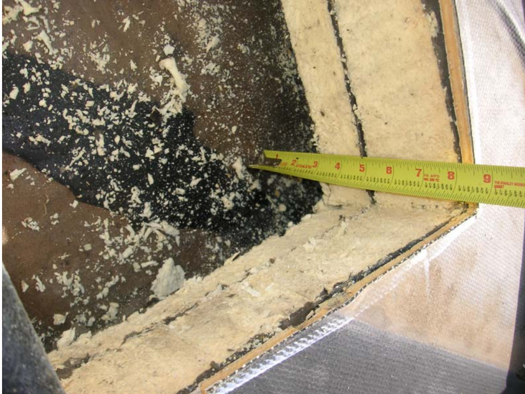
72. Total insulation with 3" delamination
