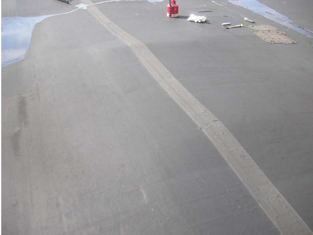
40. Large hump in the membrane
