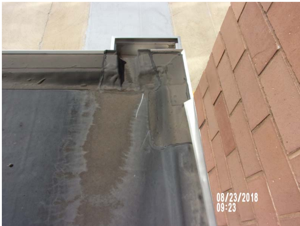
1. Roof Area S: Typical delaminating membrane.
