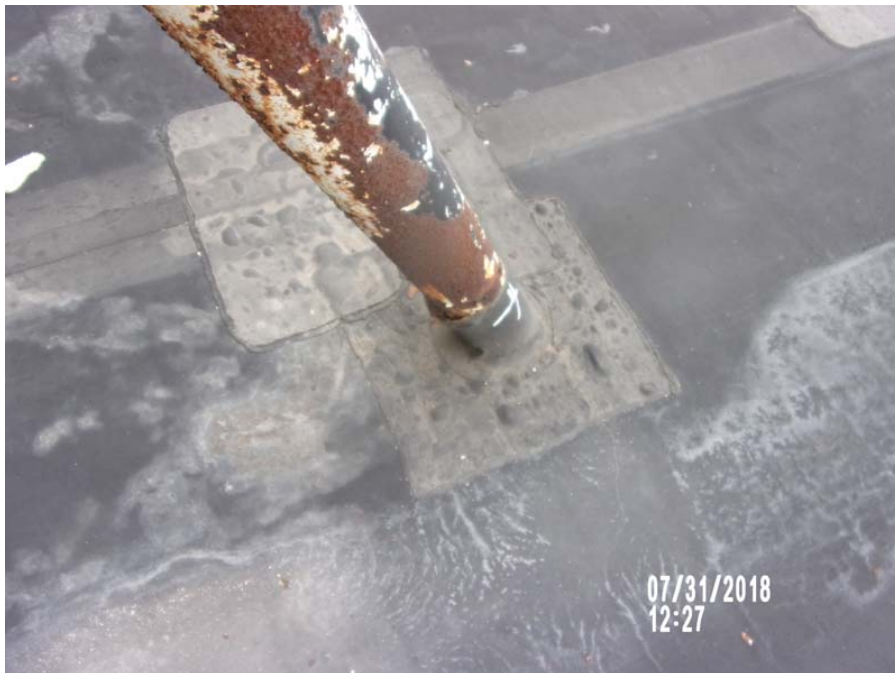
2. Roof Area D1 : Typical open EPDM membrane wrap at the base of a curtain wall pipe support.
