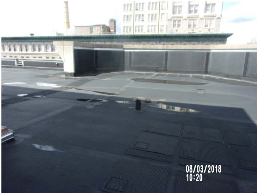
2. Roof Area B: Partial overall view of an area the insulation has delaminated from the concrete deck.
