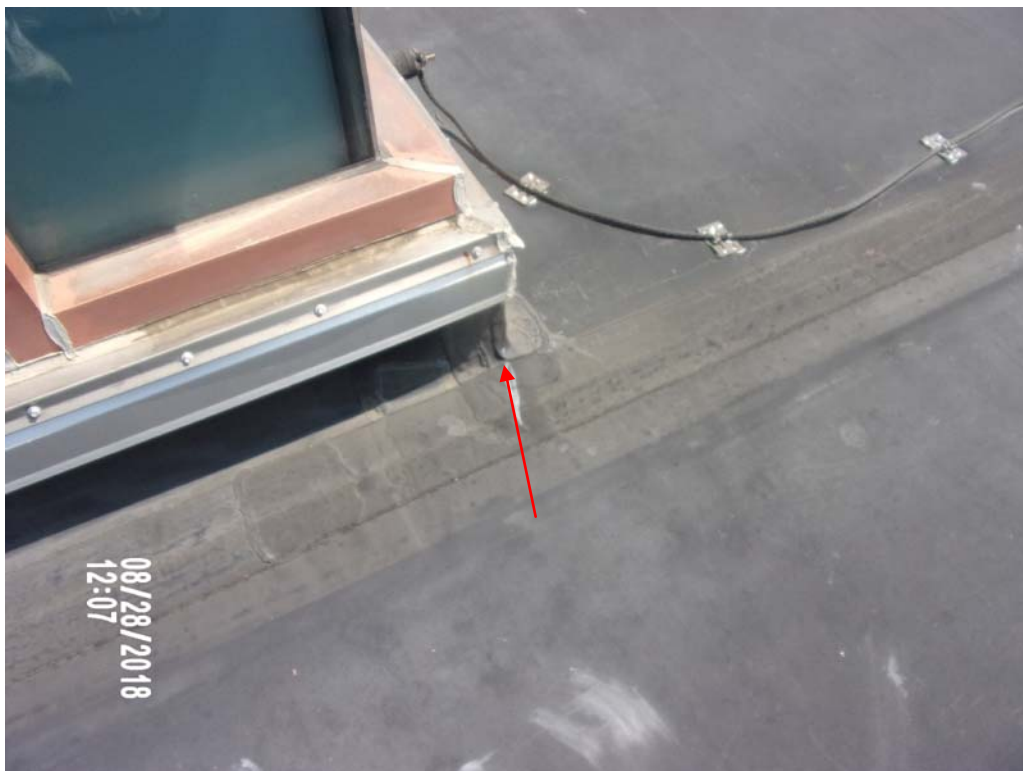
3. Roof Area C : Delaminating corner patch at the inside window wall.
