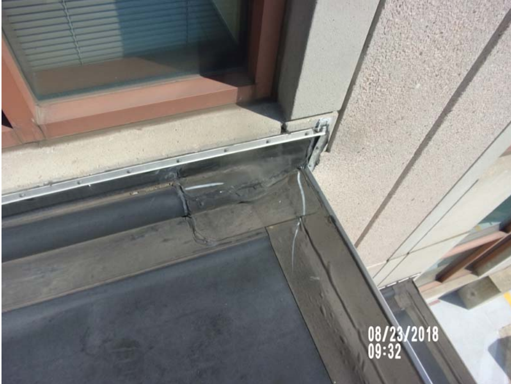
2. Roof Area R: Delaminating expansion joint end corner.
