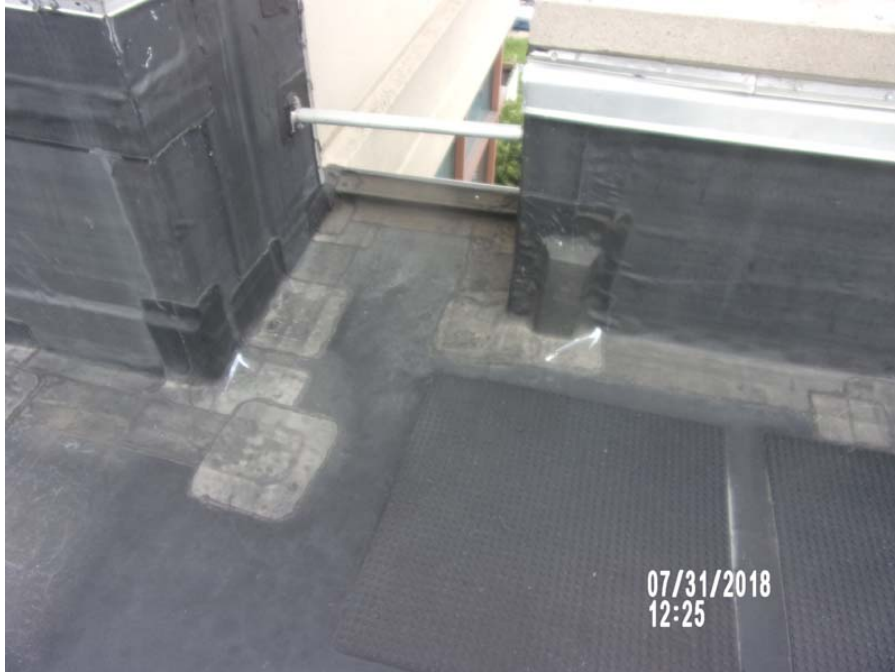
1. Roof Area D1 : Typical open EPDM membrane open vertical lap seams on parapet wall.
