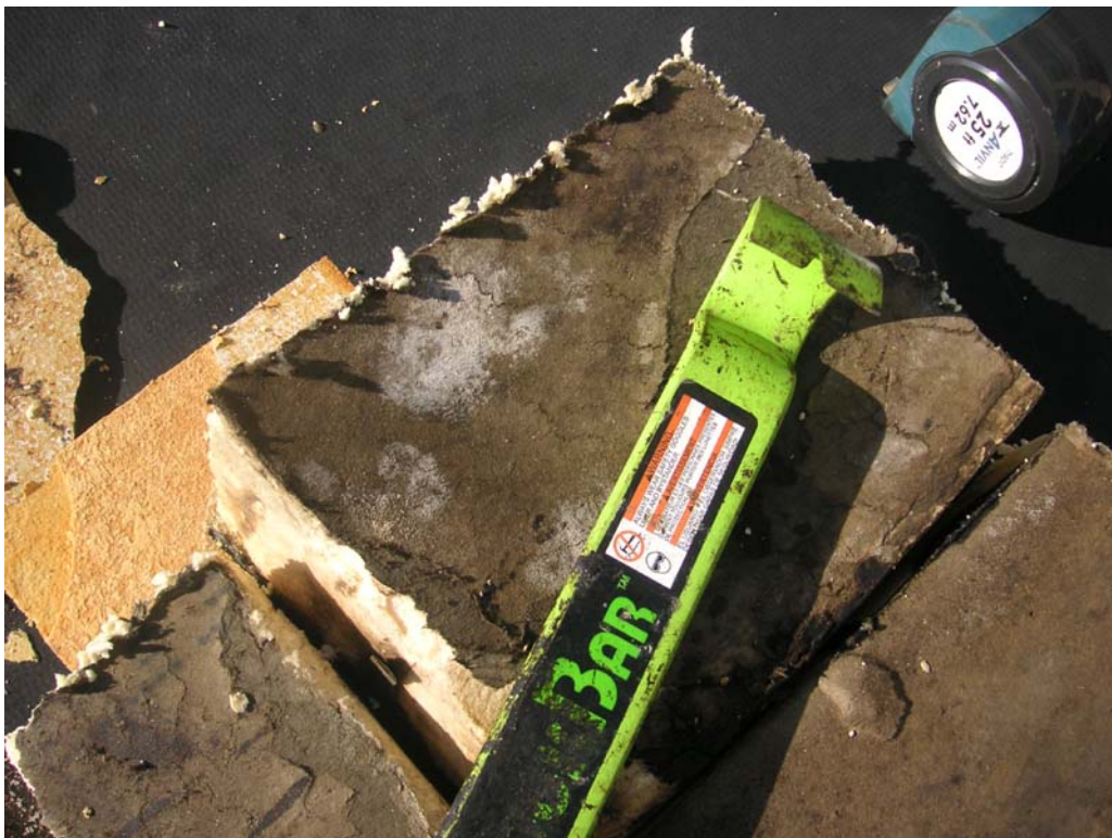
6. Mold in under side of top layer of insulation; facing sheet bloated from moisture
