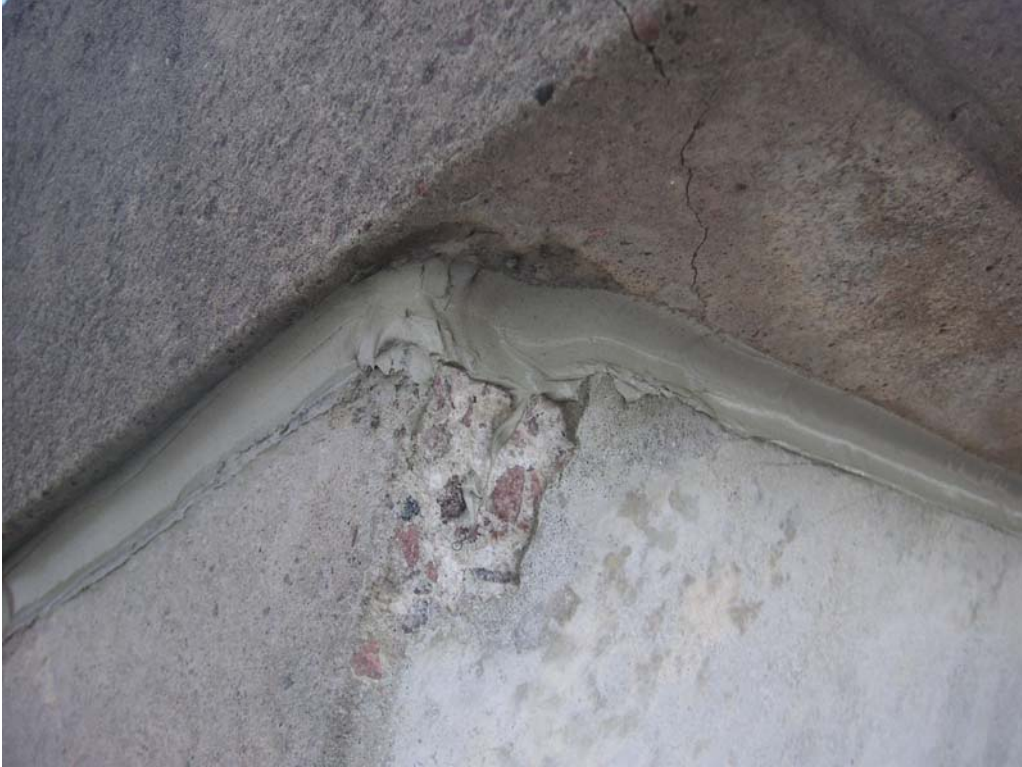
48. Caulking at cast stone – note cracks in stone
