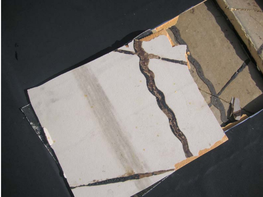
30. Bottom of hard board showing adhesive line – 8" apart
