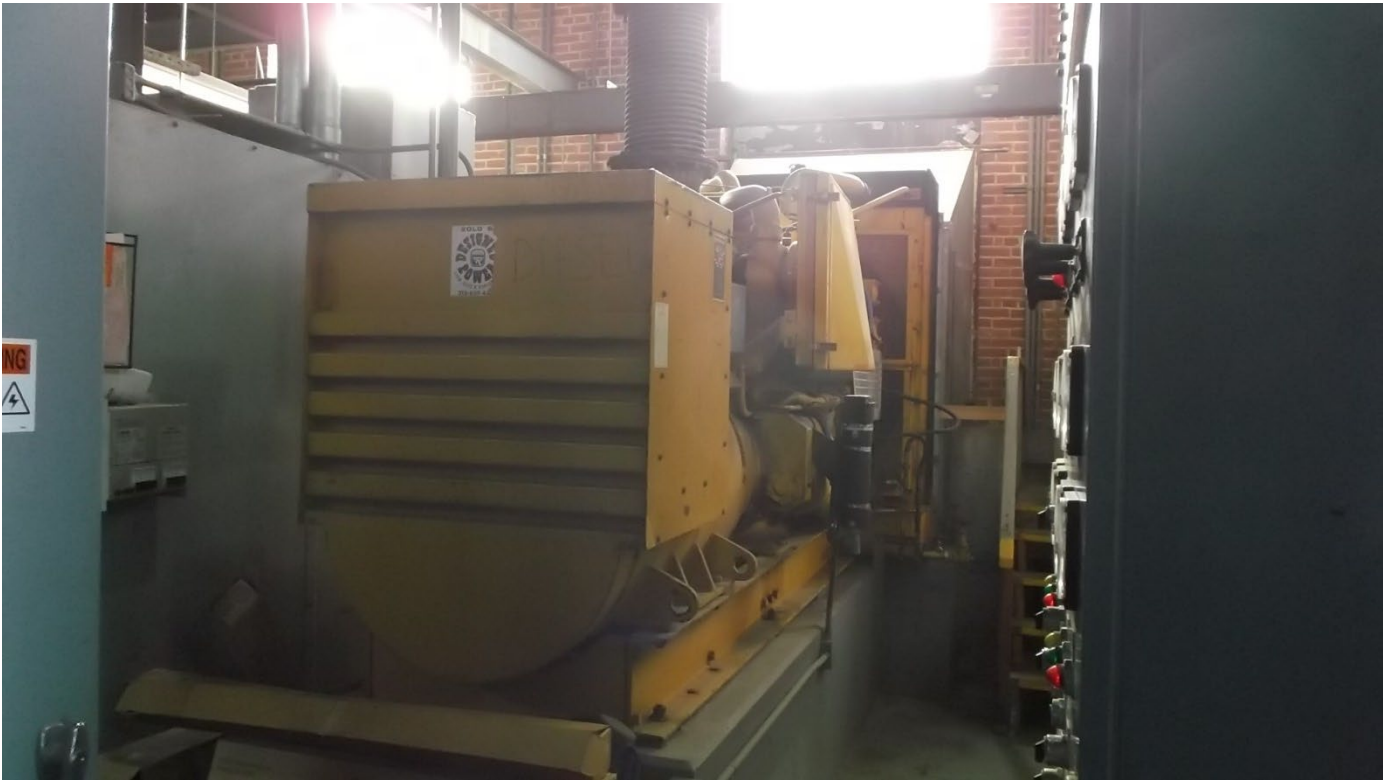
Caterpillar generator to be removed and not replaced.
