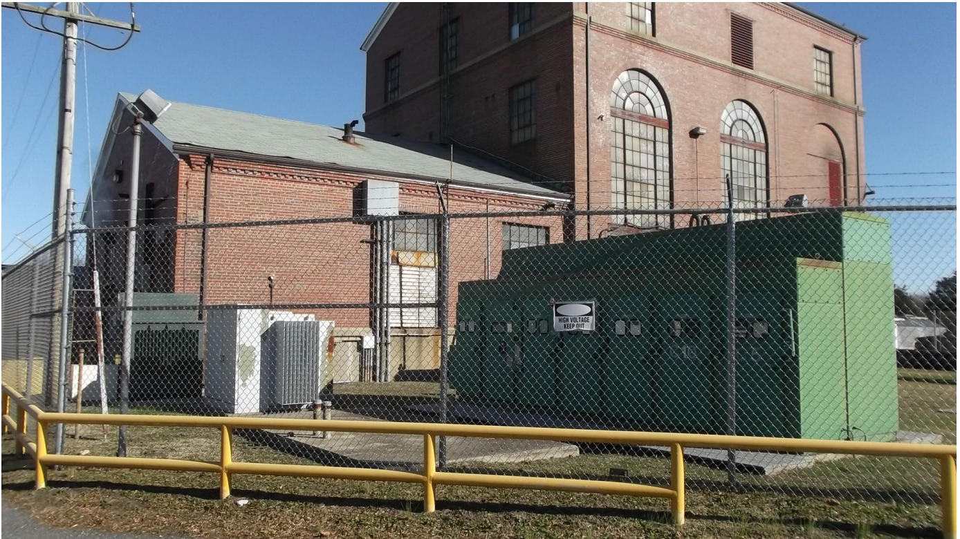
Main utility entrance from pole on left. 12.47KV and 2.4KV switchgear in green cabinets.
