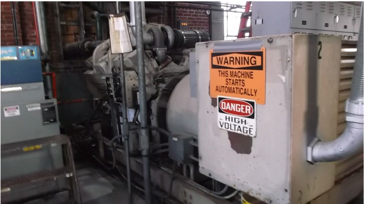
One of two 750KVA generators to be replaced. Other is similar and to the left.
