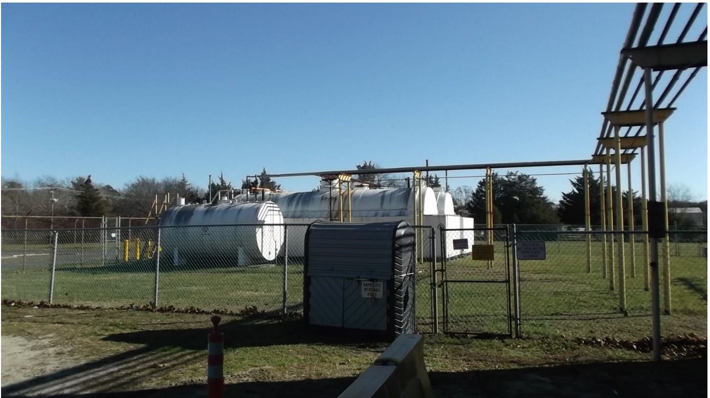
Smaller tank is fuel tank for generators. To be evaluated.
